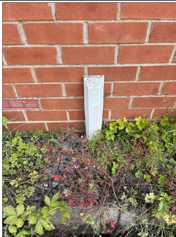
TS07 - Electric supply against exterior wall
