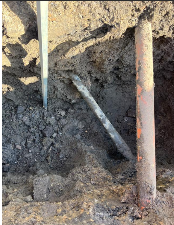
TS05 - Closer view of BT duct
