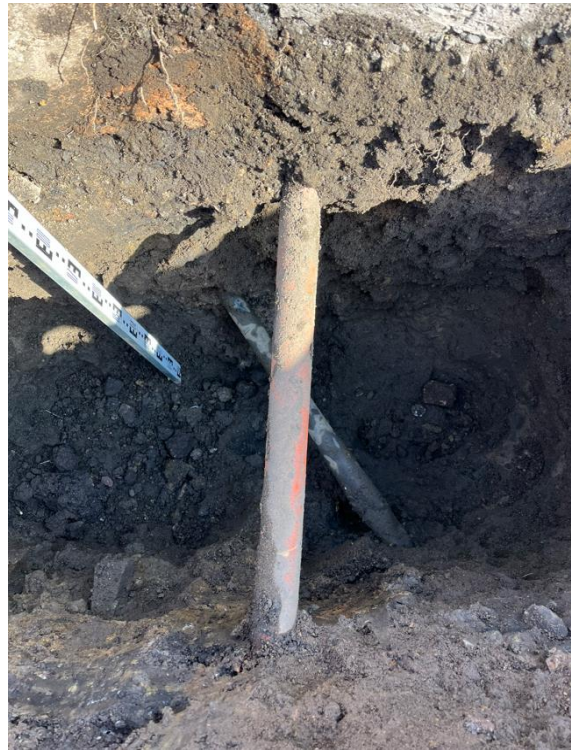
TS05 - Closer view of low voltage electric duct
