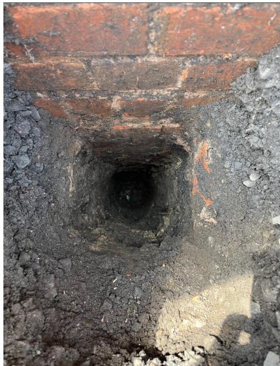
TP103 - Closer view of the pit
