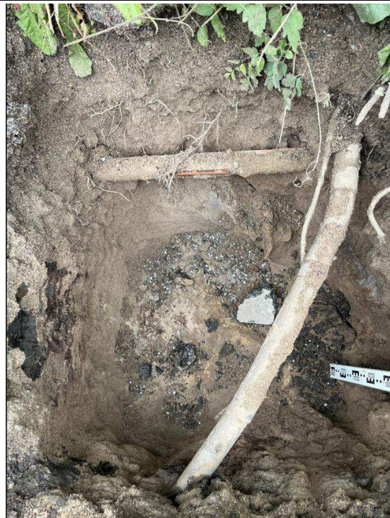
TS12 - Closer view of services
