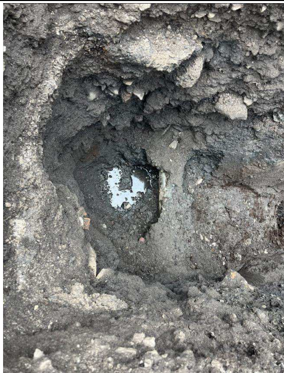
TS10 - Closer view of BT duct
