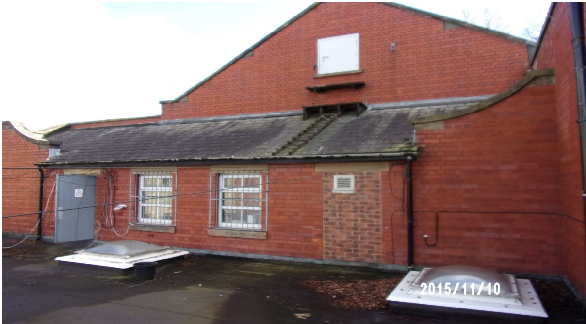
PHOTO 5: Showing mono-pitch out-rigger to the first floor along with old timber roof ladders ( very dangerous in /after wet weather ) to access the loft hatch door to the ceiling of the first floor. It is proposed to put a access platform across this elevation in order that operatives can cross from the front elevation to the rear after gaining access vis a spiral stair.
