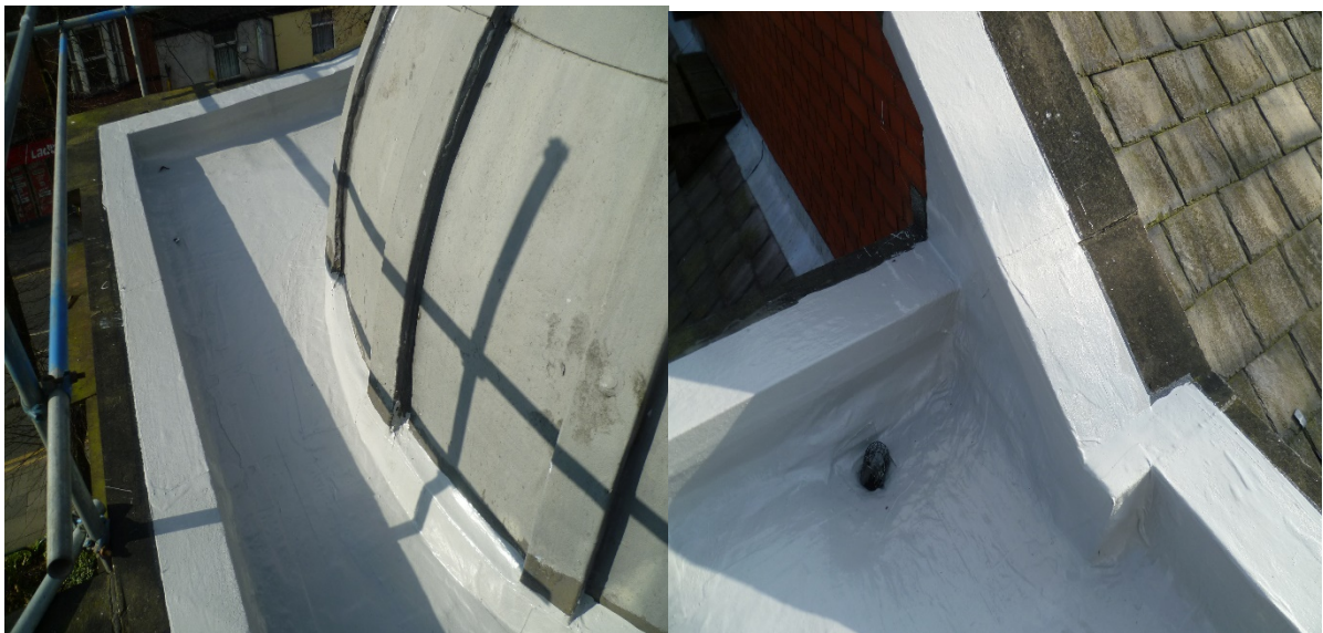
PHOTOS 3 & 4 : Taken when the liquid roofing system had been applied after ever section of code 5 lead had been stripped by thieves.
