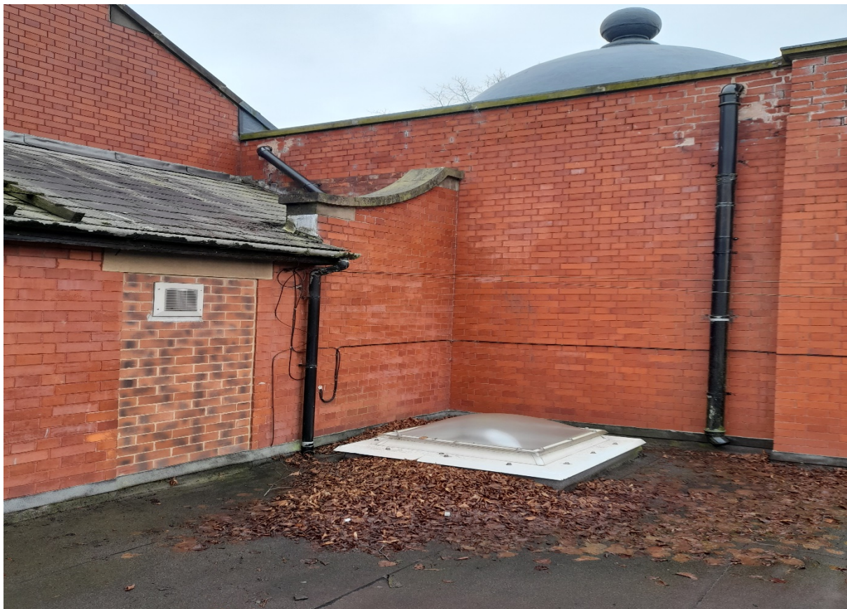
PHOTO 6 : Looking towards the wall in the last picture – you can see the amount of leaves to the lower roof that build-up but the situation is worse at roof level because of the narrow parapet detail
