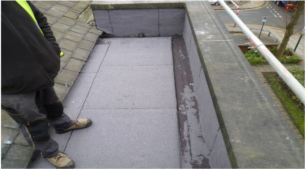
PHOTO 2 : Is a smaller big width section to the roof that has had a felt
