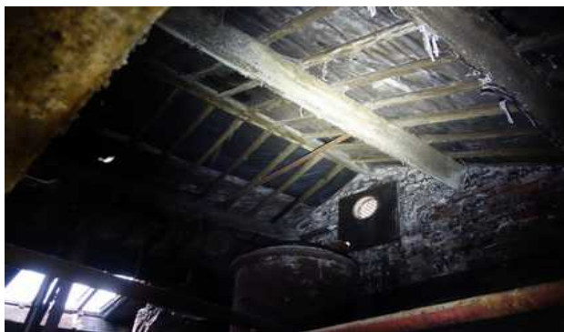
Exposed slates with evidence of considerable water penetration.
