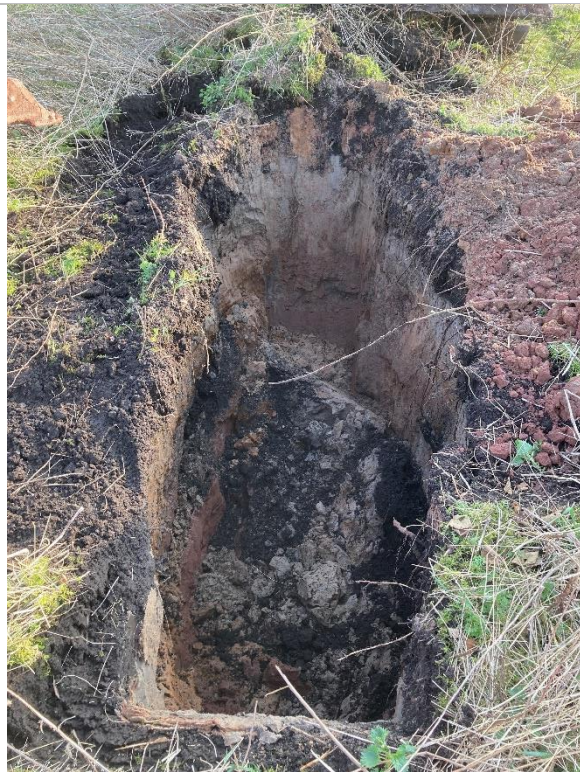
PLATE 14 UNSTABLE TRIAL PIT
