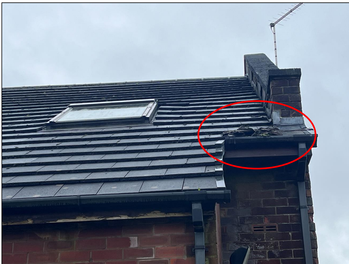
Plate 15 – Eroded roof tile at north-western corner of building
