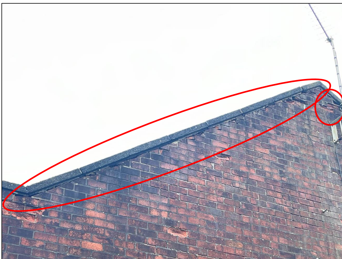
Plate 16 – PRFs in brickwork of western gable elevation
