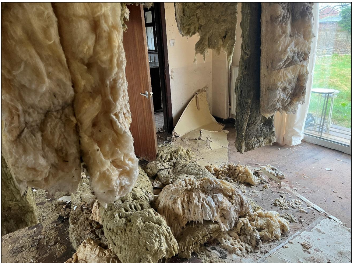
Plate 20 – Collapsed nature of the loft space floor
