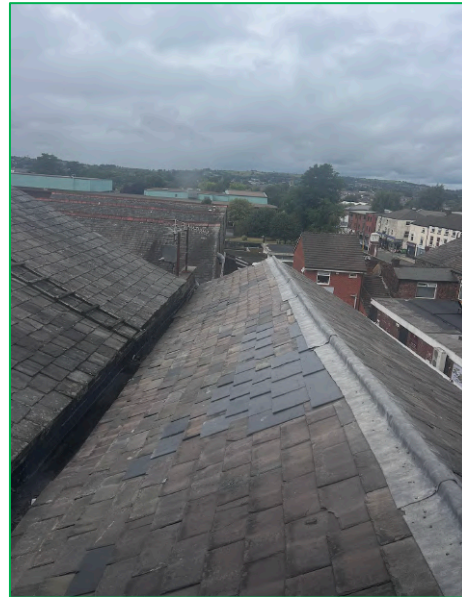
Showing the generally well-fitted slates on the western end of the building. Newer slate show some small crevices
