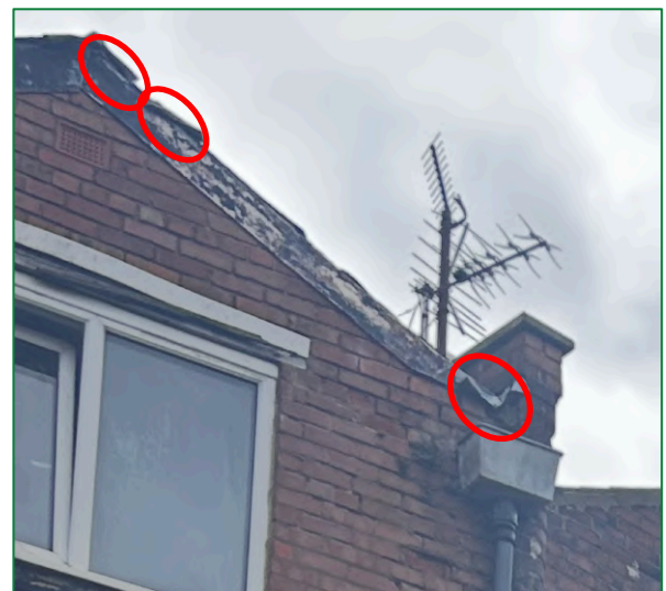
Showing crevices under slates and under lead flashing on the west elevation
