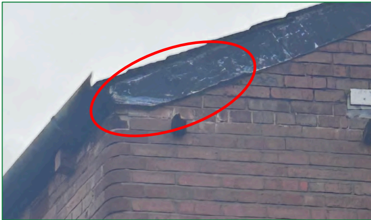
Showing a gap under the fascia on the west elevation
