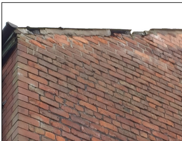
Plate 2 Missing mortar at gable end of B1 provides potential roosting habitat for bats
