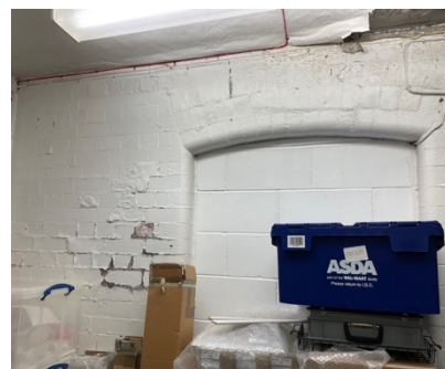
20 Water ingress and failing finishes in LG0021 (2023)
