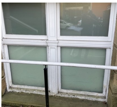
12 Decayed timber cills on WLG06 (2023)
