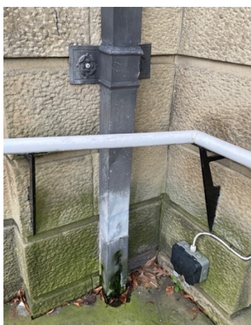
06 Damage to leadwork of RWP01 at ground level (2023)
