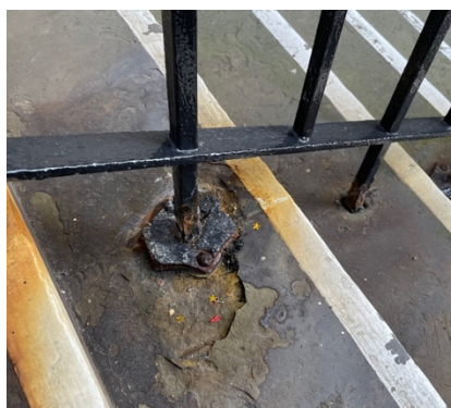
16 Corrosion in handrails (2023)
