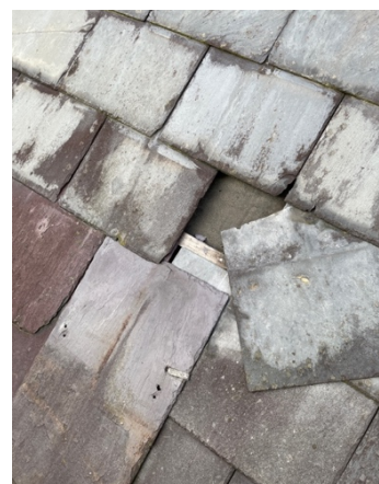
05 Slipped slates to the north of RL04 (2023)
