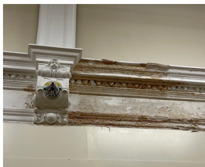
19 Significant water ingress to F0015 and consequent damage to plasterwork (2023)
