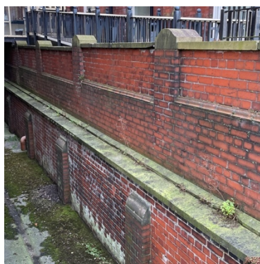
15 Growth on retaining wall and plinth (2023)
