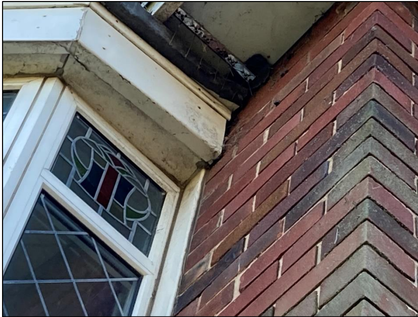
Photograph 2 showing the small gap on the bay windows
