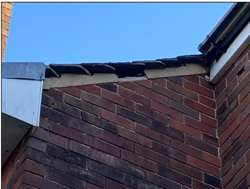
Photograph 5 showing the area of the damage on the mortared sections of the roof
