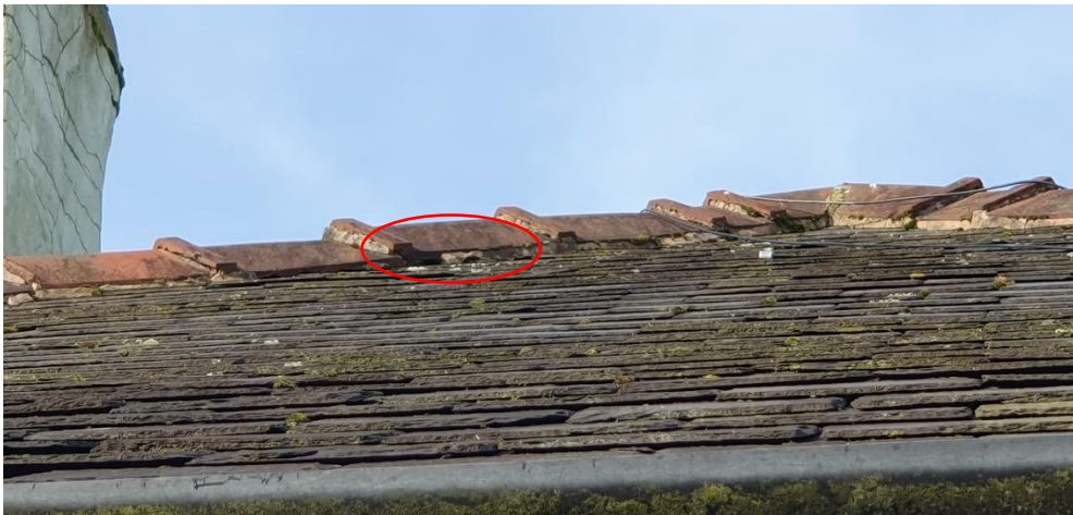
B1 – area of missing mortar under eastern ridge tile
