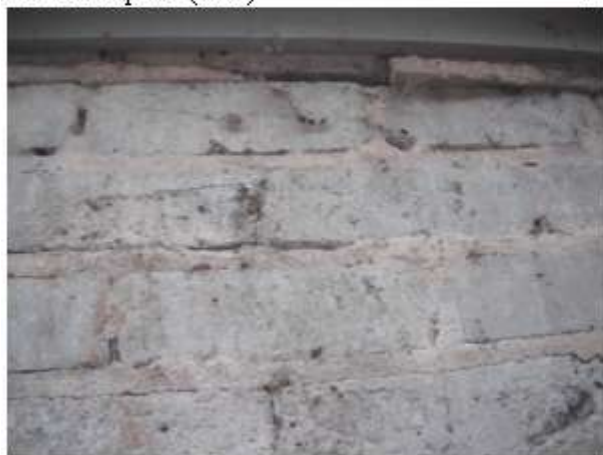
P5 Gap in masonry, building 6
