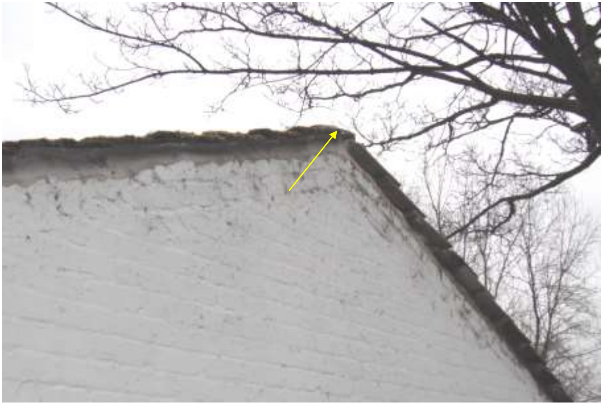
P7, as P4 with ridge tile removed
