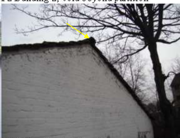
P4 NW gable (building 1) gap under ridge tile
