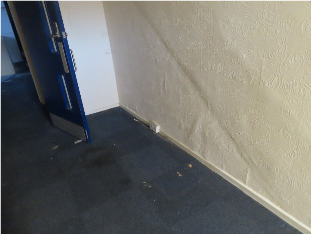
Outline of removed staircase to number 20 and area of dampness.
