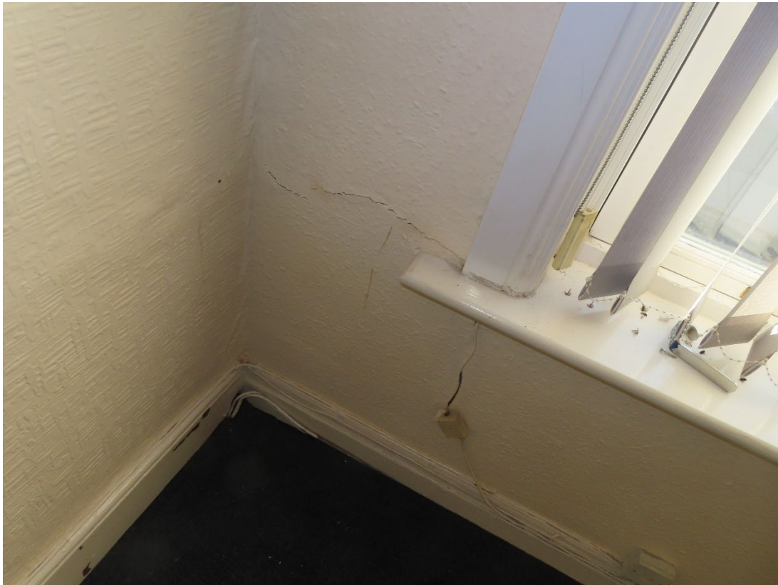
Horizontal cracking to front wall to the first floor small office to number 20.
