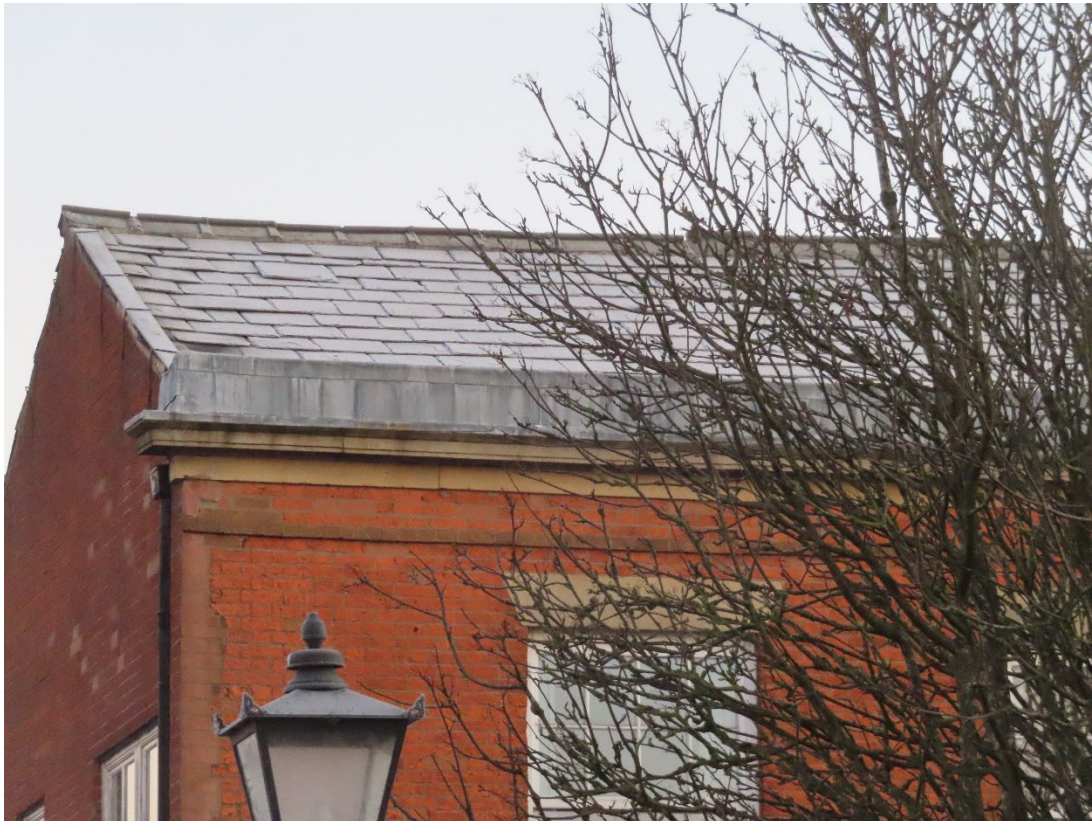
Slipped slate to front roof of number 20.
