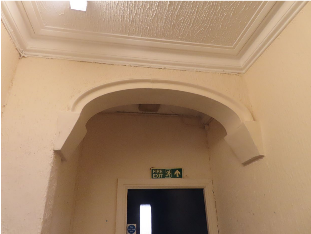
Heavy artexed wall and ceiling and staircase lobby to number 18.
