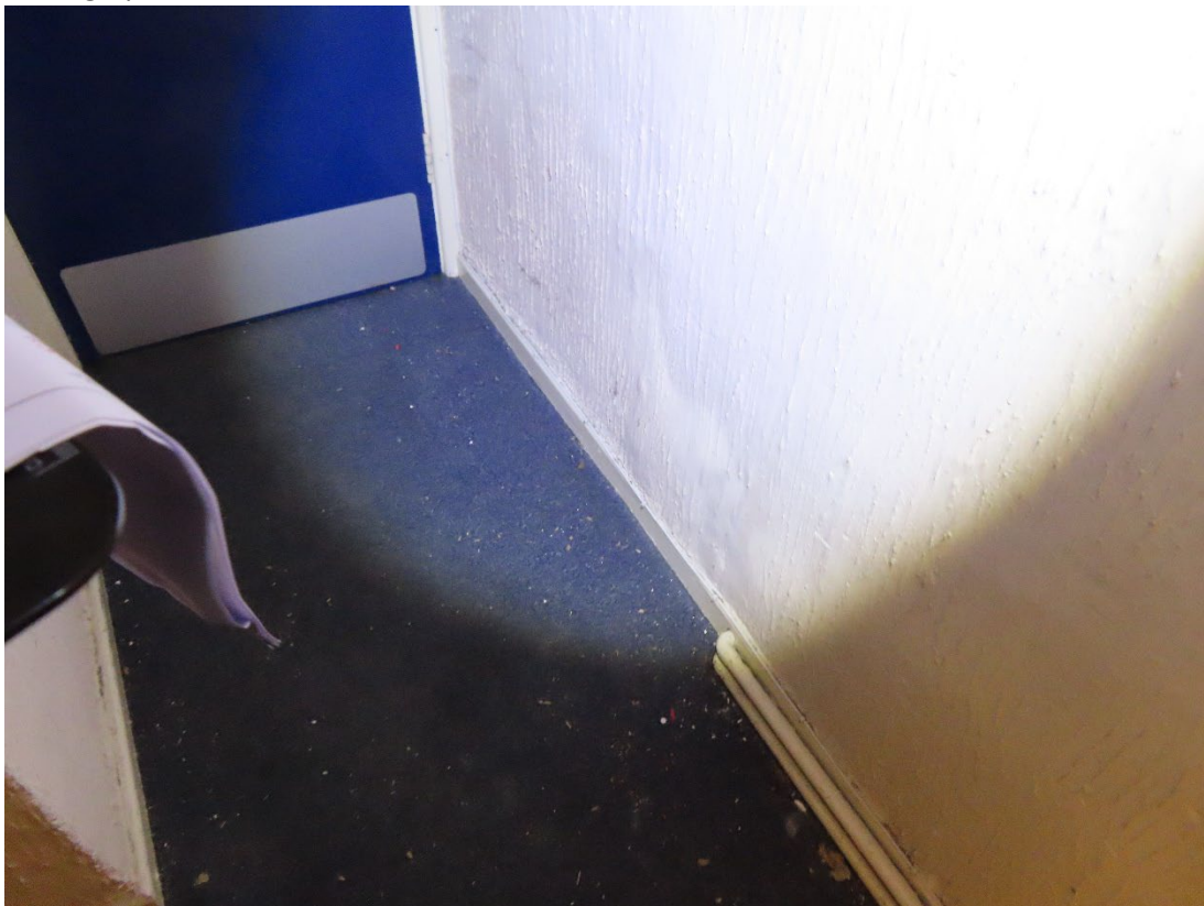
Rising dampness to wall linking number 18/20 rear cellar steps to number 18.
