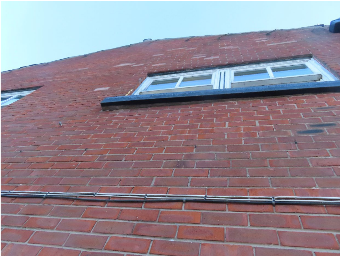
Out of line sill to first floor sill to gable end.
