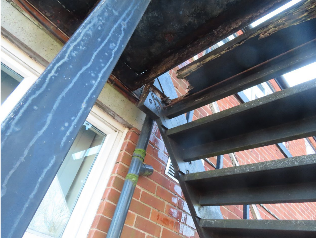
Dangerous tread to first floor fire escape to number 20, also check stringers.
