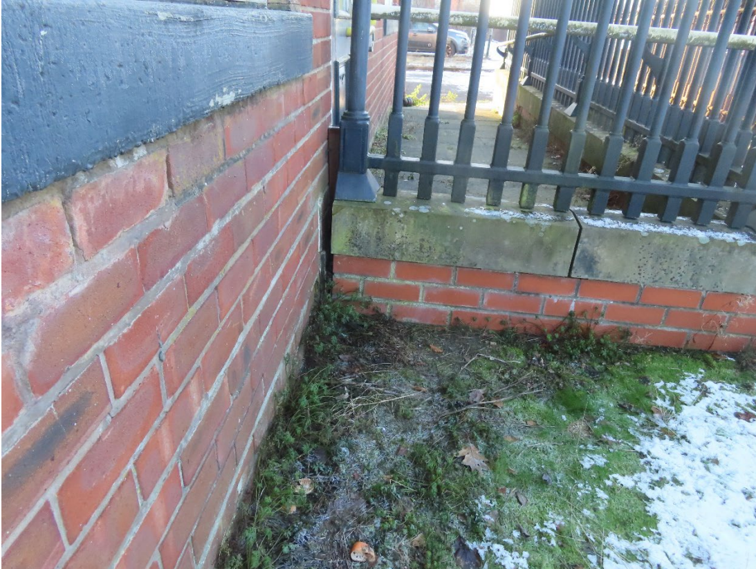
Differential settlement to external ramp detail to rebuild gable to number 20.
