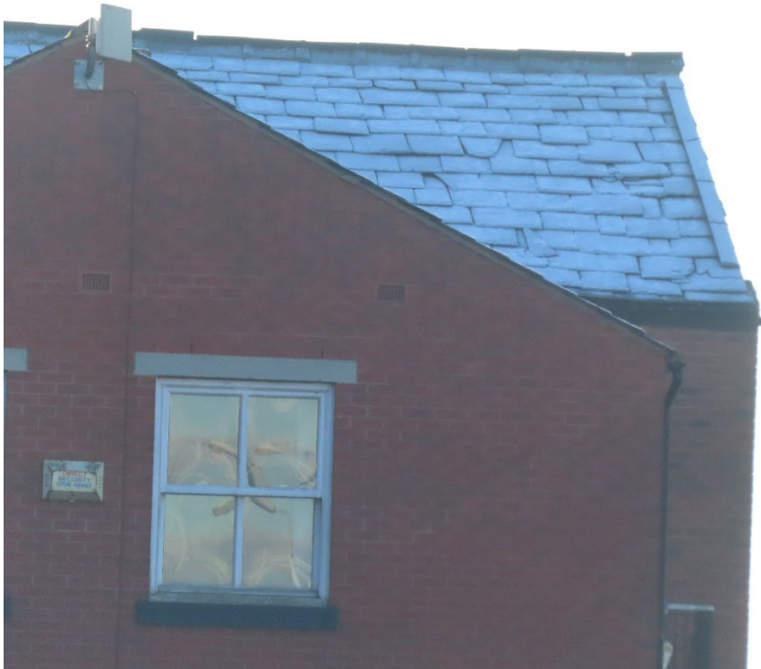
General poor condition of slate roof to the rear of main building to number 20.
