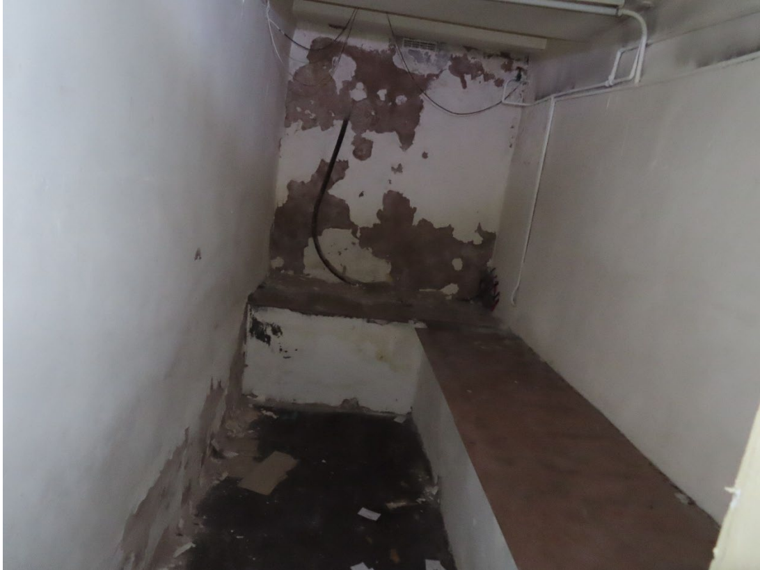
General dampness to basement 3 cellar to number 20.
