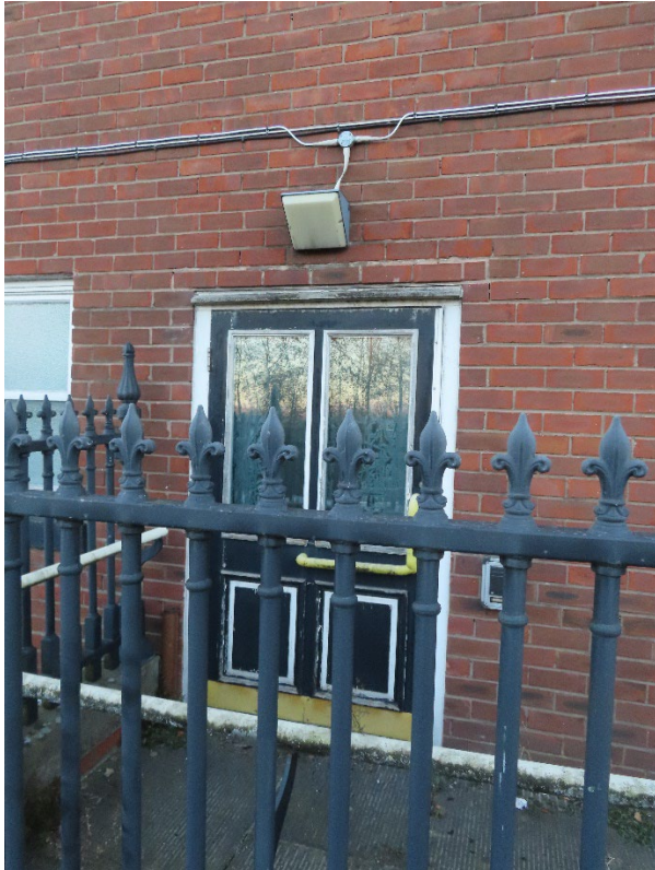
General poor external decorations
