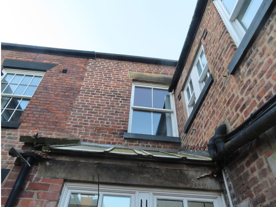
Gutter required to rear outshot of number 18.
