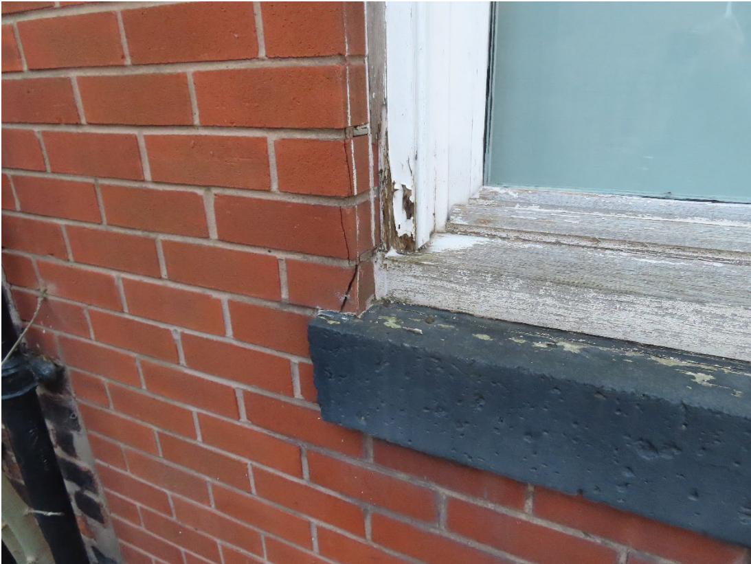
Wet rot to box section of sliding sash window to wc ground floor extension to number 18.
