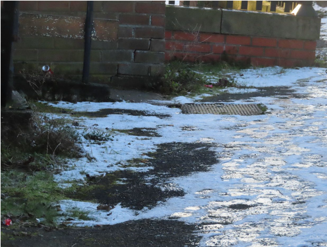
Cracking to brick wall potential cause by drainage (drainage report required).
