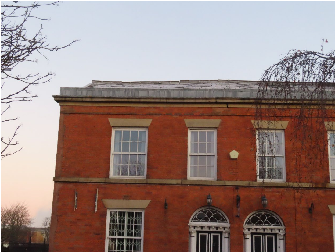
Drop in ridge line due to settlement to number 20.
