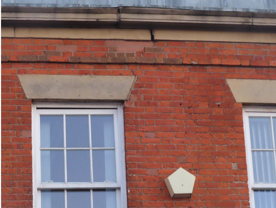
Old differential settlement to front wall party wall line to number 20.
