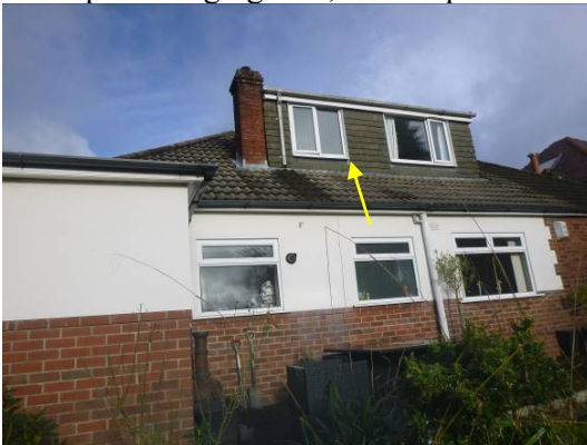
P5 Gaps at hanging tiles, rear aspect
