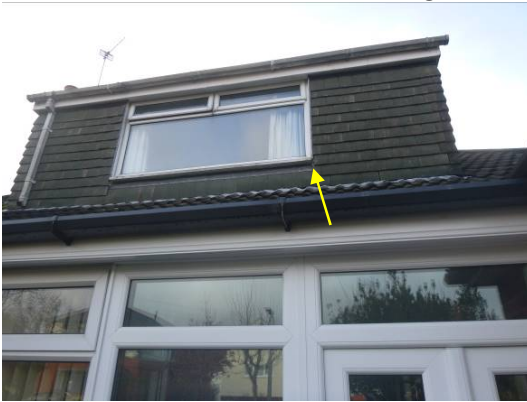
P3 Gaps at hanging tiles, front aspect
