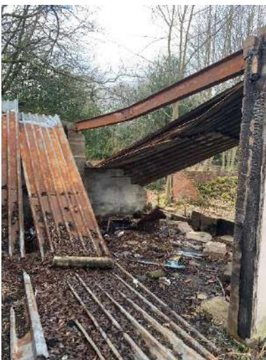
Figure 17 – A more recent outbuilding, also now derelict, with sheet metal roofing rather than suspected ACM.
