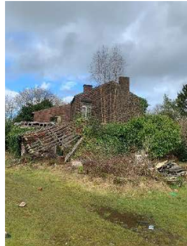
Figure 20 – Looking north towards the on site dilapidated house.
