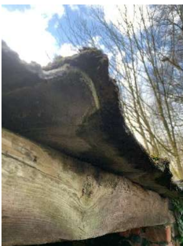
Figure 23 – Suspected ACM asbestos cement roofing still in place on an outbuilding in the north west of site.
