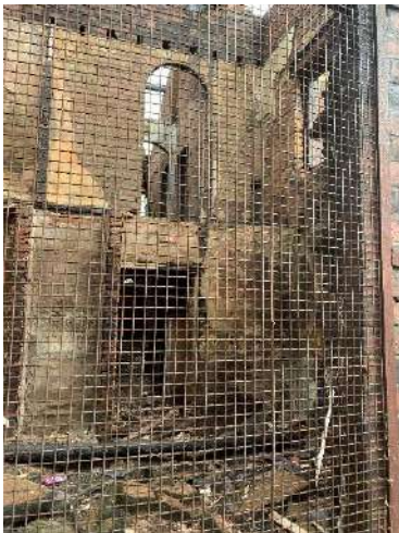
Figure 21 – The inside of the house on site showing the poor condition of the property.
