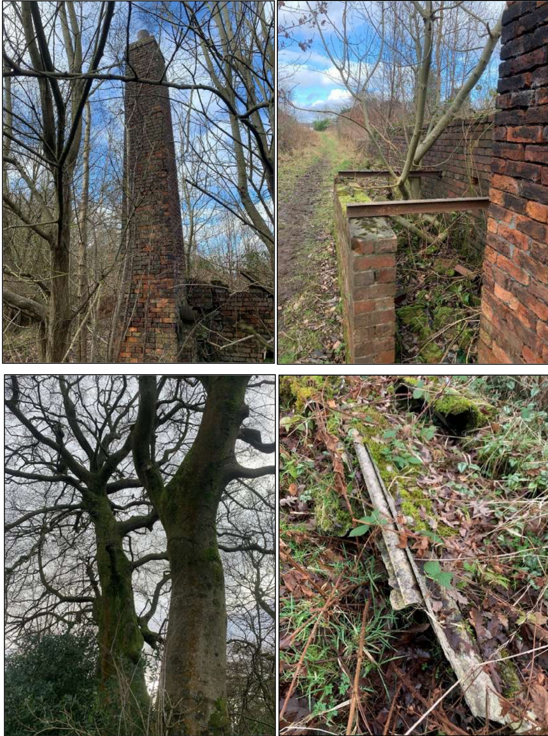
Figure 2; Images from the site walkover: top left – the historic chimney, top right – potential historic above ground tank base, bottom left – one of the mature trees on site, bottom right – a pile of suspected ACM (asbestos cement sheeting).
