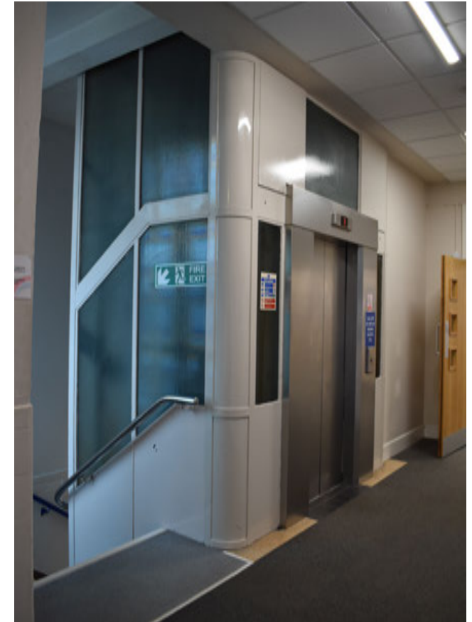
3.77 North entrance lift
