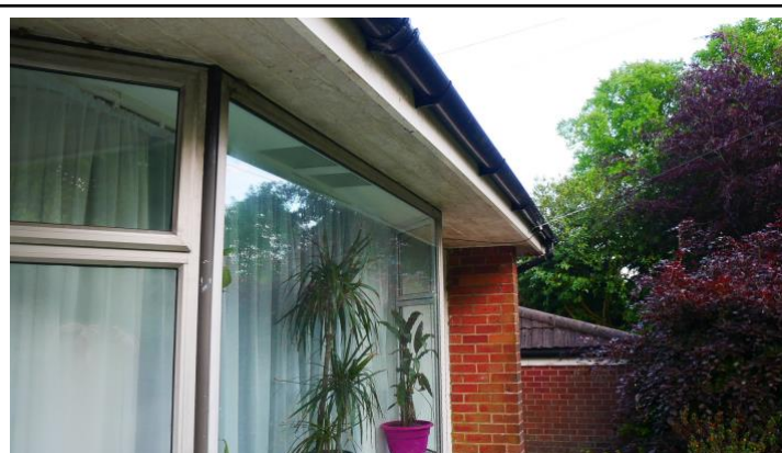
5. All glass surfaces checked for evidence of bat activity – droppings present on surfaces
