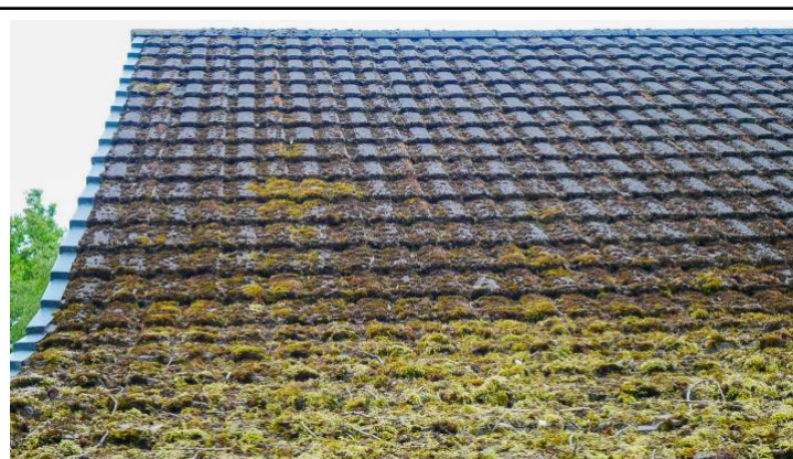
7. Area of front roof heavily mossed
