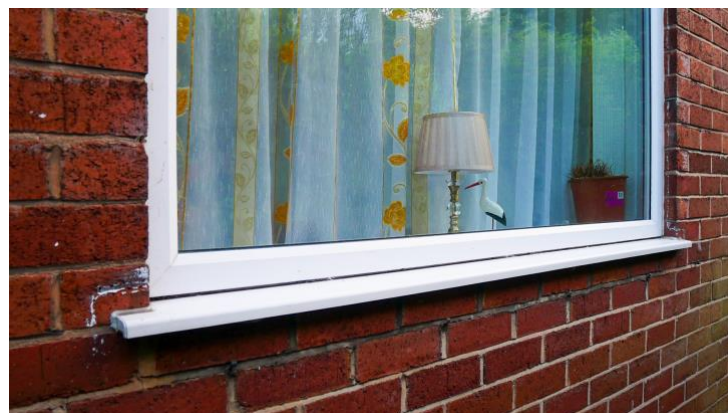
2. All glass surfaces checked for evidence of bat activity – droppings present on surfaces
