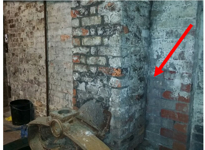
Sample No: 22/3/B/9/IL13. B.01 Basement Area 1 - Old Boiler Room – Wall. Residual insulation to wall containing: Amosite & Chrysotile.
