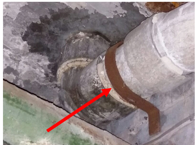
Sample No: 22/3/B/8/IL7. B.01 Basement Area 1 - Plant Corridor – Flue. Woven gaskets / seals to flue joints / sections containing: Chrysotile.
