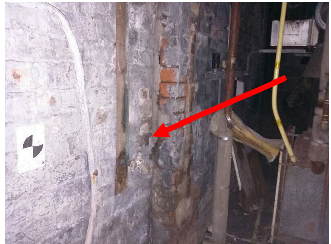
Sample No: 22/3/B/8/IL5. B.01 Basement Area 1 - Plant Corridor – Wall. Residual insulation to wall containing: Crocidolite & Chrysotile.
