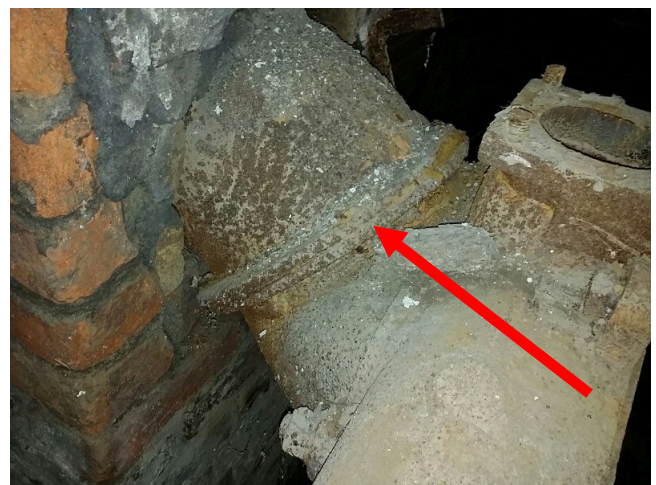
No Sample Taken. B.01 Basement Area 1 - Old Boiler Room - Boiler / flue joint. Flange gasket containing: Chrysotile.
