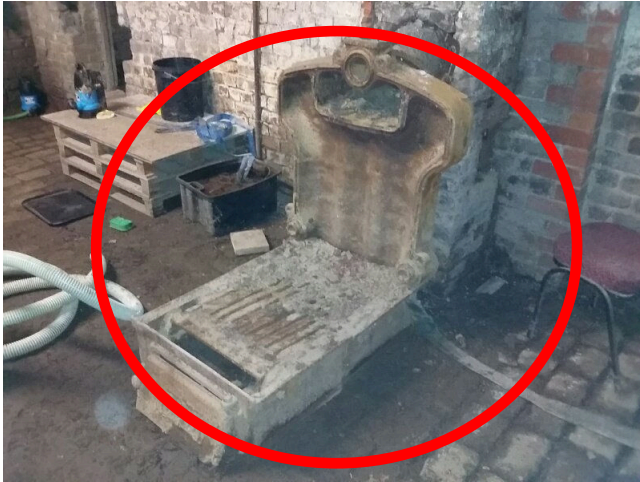
Sample No: 22/3/B/9/IL12. B.01 Basement Area 1 - Old Boiler Room - Redundant boiler. Residuals & debris to redundant boiler containing: Amosite & Chrysotile.
