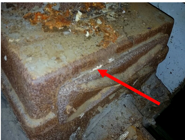
Sample No: 22/3/B/8/IL2. B.01 Basement Area 1 - Plant Corridor - Gas Boiler. Woven gaskets to boiler hatches containing: Chrysotile.
