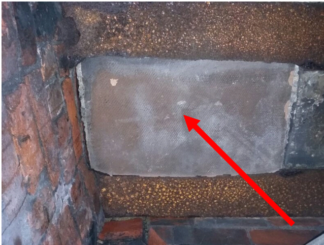
Sample No: 22/3/B/8/IL4. B.01 Basement Area 1 - Plant Corridor – Ceiling. Localised cement shuttering to ceiling containing: Chrysotile.
