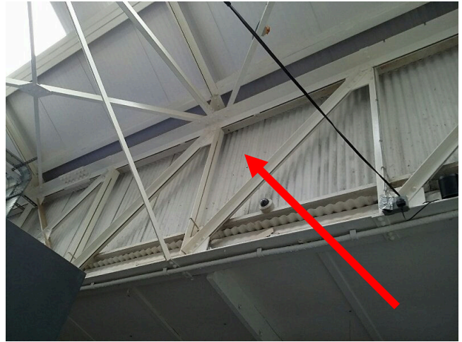
Sample No: 22/3/B/9/IL22. G.02 Market Hall Circulation Area - High level perimeter wall. Corrugated cement wall sheets containing: Chrysotile.
