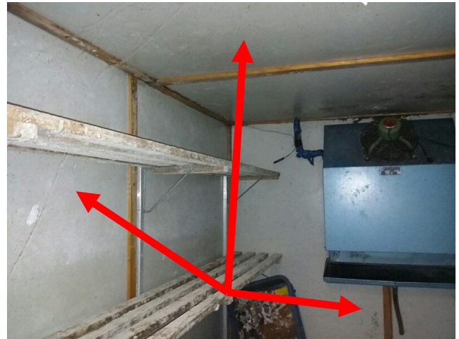
Sample No: 22/3/B/9/IL18. B.02 Basement Area 2 - Walk-in Fridge. Internal wall & roof linings containing: Chrysotile.
