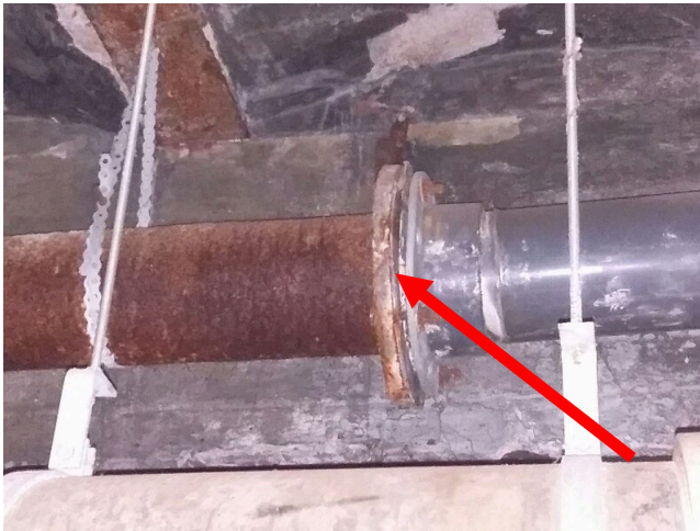
Sample No: 22/3/B/8/IL8. B.01 Basement Area 1 - Plant Corridor – Pipework. Pipework flange gaskets containing: Chrysotile.
