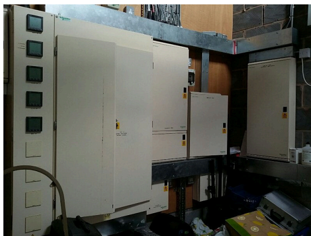
Room: G.12 - Modern electrical plant / equipment.
