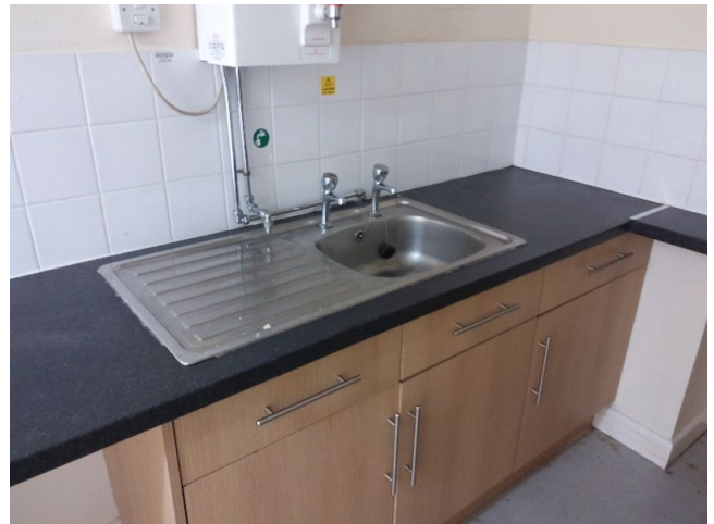
Sample No: 22/3/B/21/PK3 B.03 Welfare / kitchen Sink Bitumen pad No Asbestos Detected
