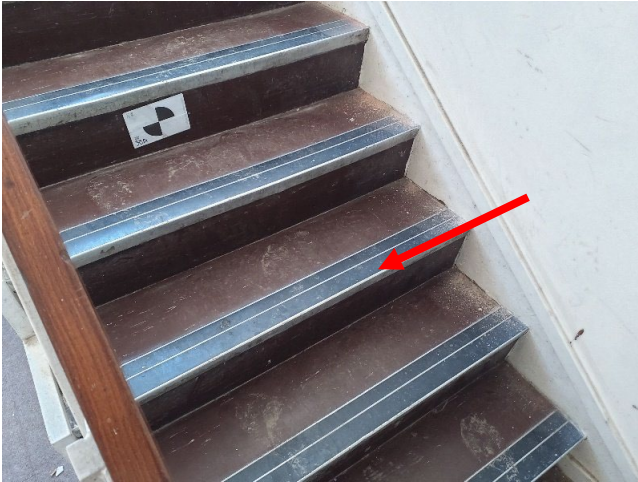
Sample No: 22/3/B/22/PK14 G.13 1st floor stairwell Stairs Vinyl stair nosings containing: Chrysotile
