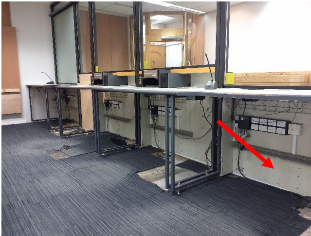
Sample No: 22/3/B/21/PK6 G.07 Staff area Customer counter Fibrous lining panels to counter No Asbestos Detected
