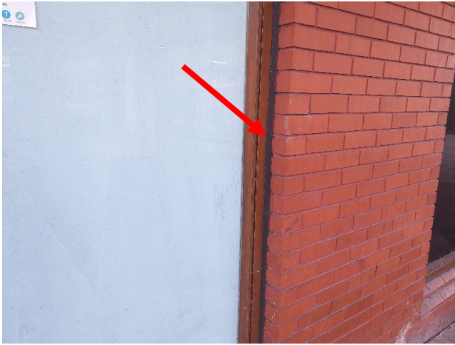
Sample No: 22/3/B/22/PK10 External Windows Mastic seal to frames containing: Chrysotile
