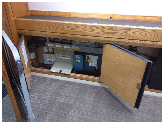
Modern electrics in G.02 customer area
