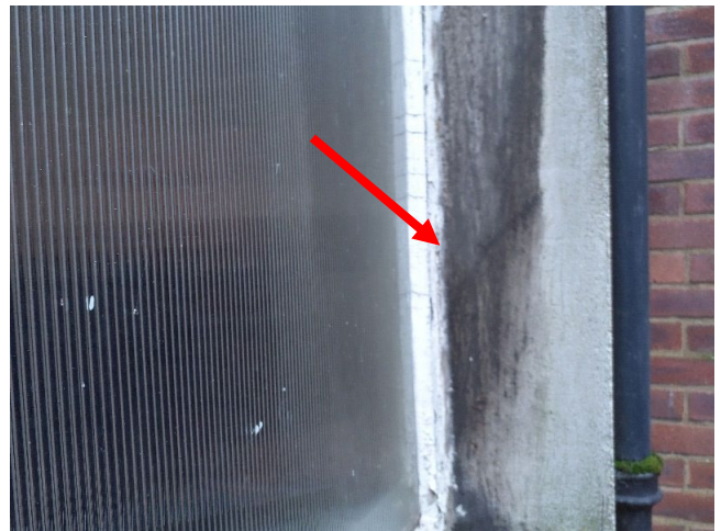
Sample No: 22/4/B/4/PK19 External Windows Mastic seal to window frames containing: Chrysotile
