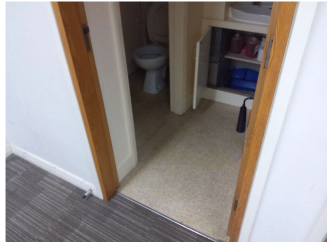
Sample No: 22/3/B/21/PK7 G.08 Male WC Floor VFC No Asbestos Detected
