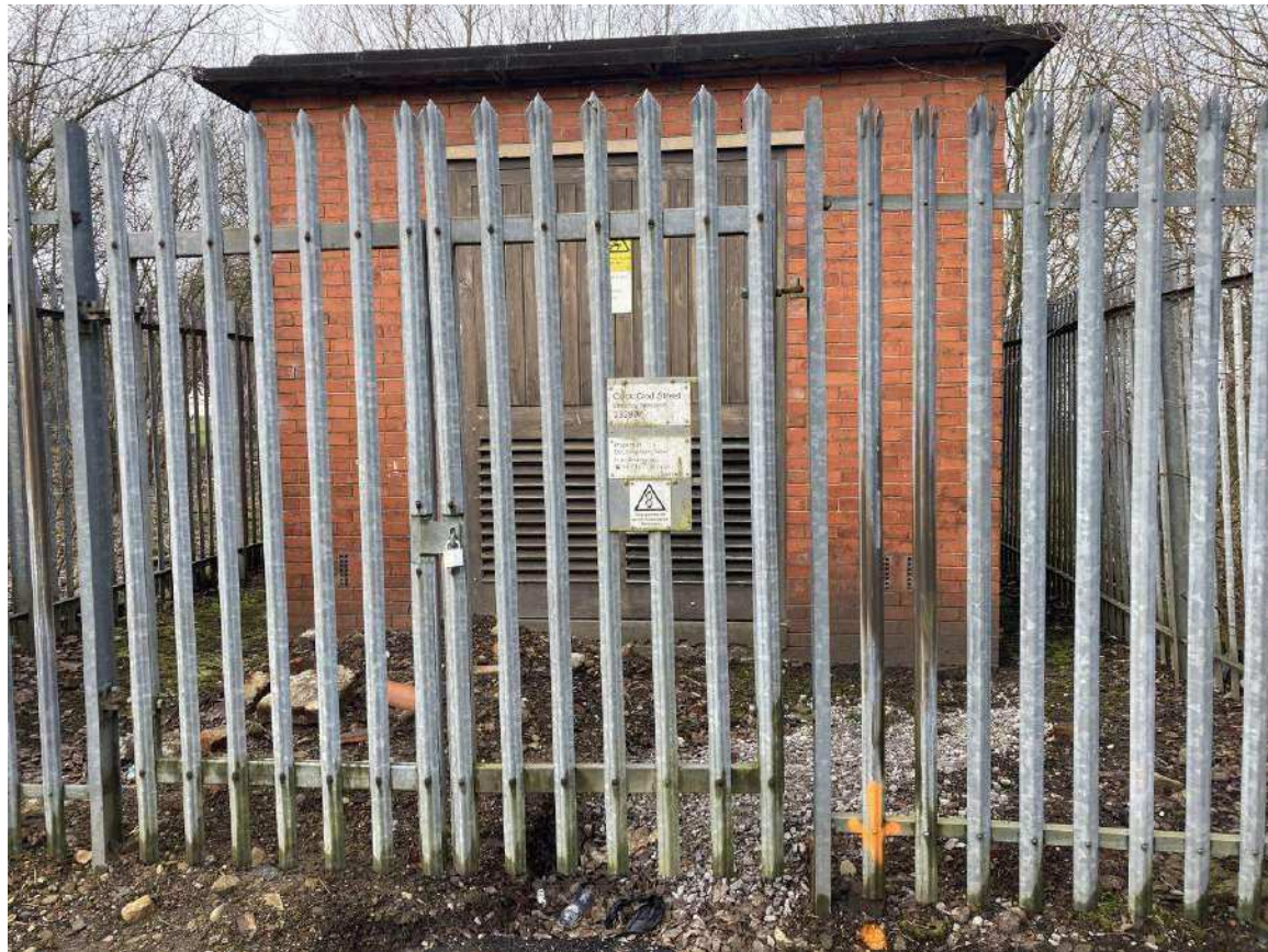
Plate 15 – Electrical substation in north west corner
