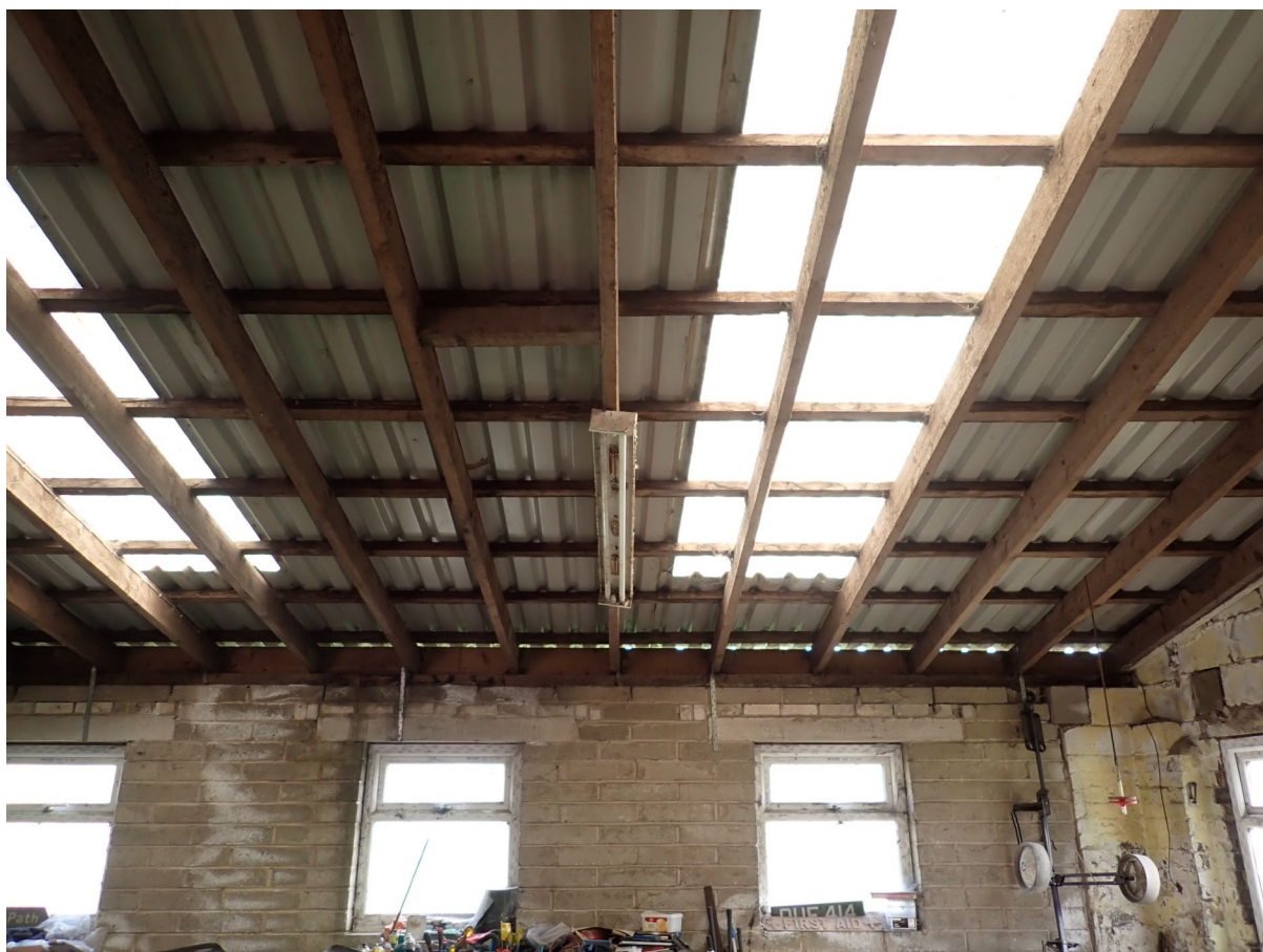
7 – The western section of the roof is not lined.
