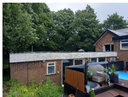
Photograph 2: View of derelict pool building. Note overhead power lines and cracks beneath damaged lintels.
