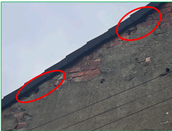
Showing gaps in the brickwork on the west elevation
