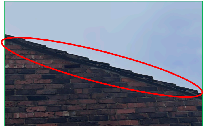
Showing crevices under tiles on the south elevation where mortar has fallen away
