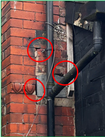
Showing crevices in the brickwork on the north elevation
