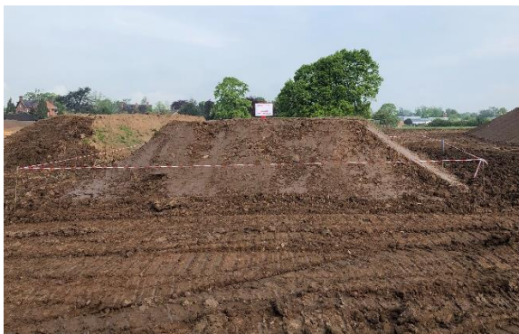
Stockpile sealed and cordoned off with warning sign
