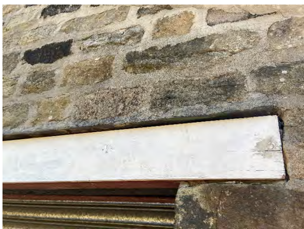
Photo 12: Gaps around wooden lintel of garage door
