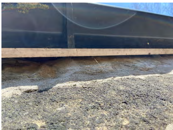
Photo 8: Gaps between gutterboard and stone walls
