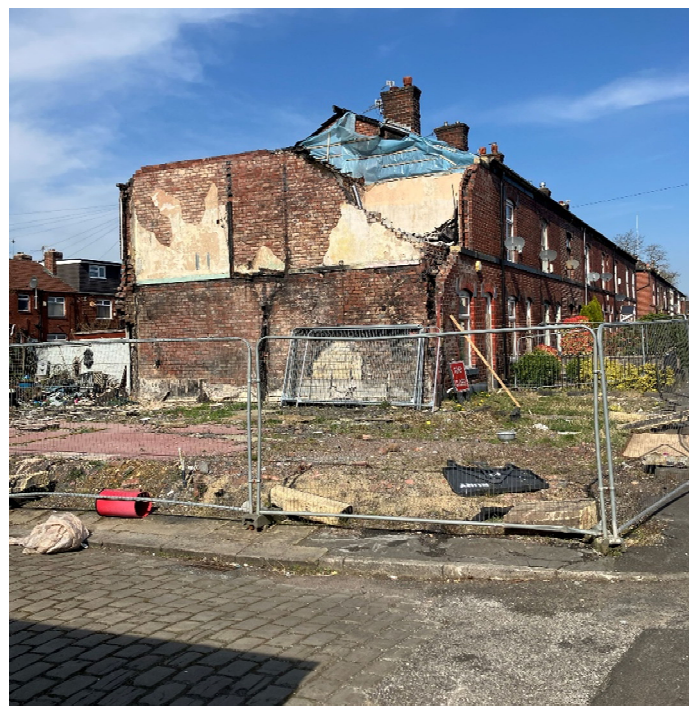
11.4 Photo taken post-damage and in its existing condition, viewing from the side South Elevation, from Back Gigg Lane.
