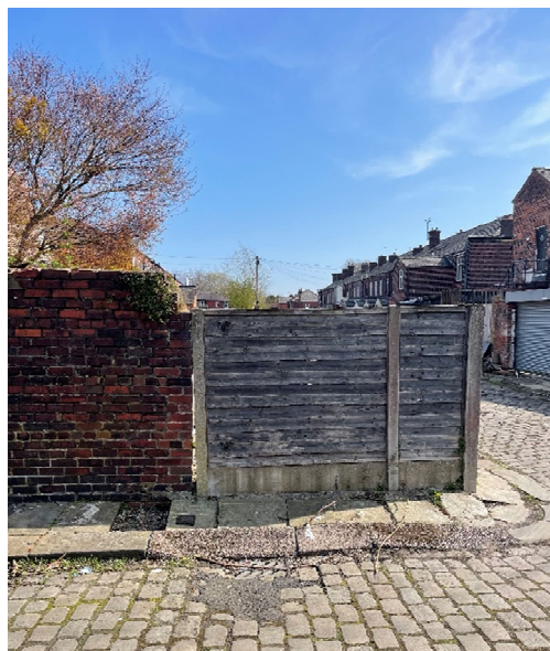
11.6 Photo taken post-damage and in its existing condition, viewing from the rear East Elevation, from Back Nelson Street South.
