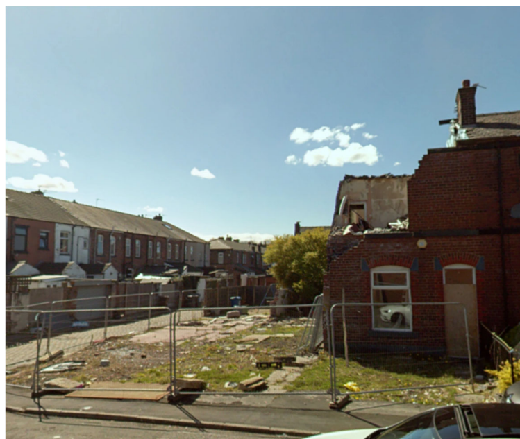
11.2 Photo taken post-damage and in its existing condition, from front West Elevation.
