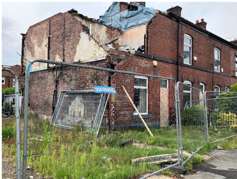
11.2 Photo taken post-damage and in its existing condition, from front West Elevation.
