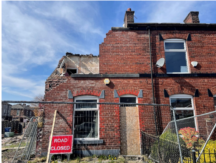
11.3 Photo taken post-damage and in its existing condition, from front West Elevation.
