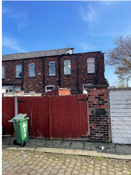
11.5 Photo taken post-damage and in its existing condition, from rear East Elevation.
