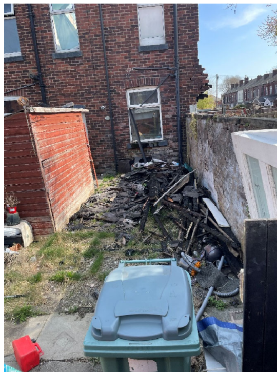
11.6 Photo taken post-damage and in its existing condition, from rear East Elevation.
