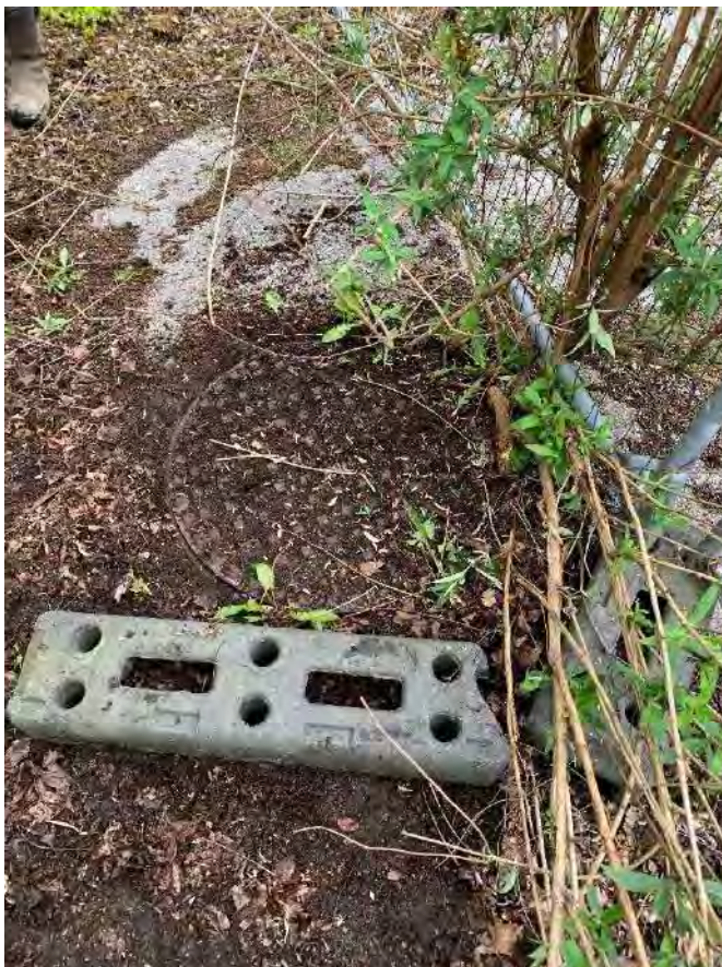
2 – MH on pipe
