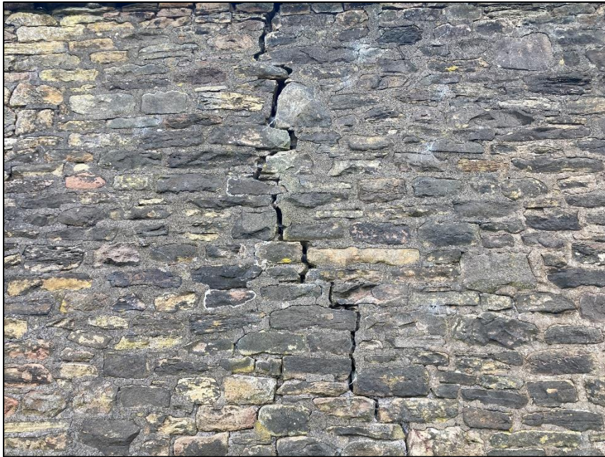
Photograph 3 showing the crack within the stone wall
