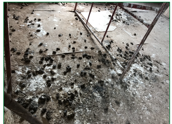
Scattered barn owl pellets and droppings in the building in August 2022
