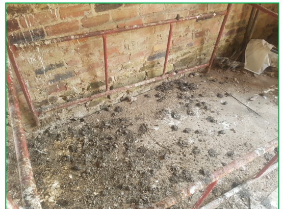
Scattered barn owl pellets and droppings in the building in August 2024
