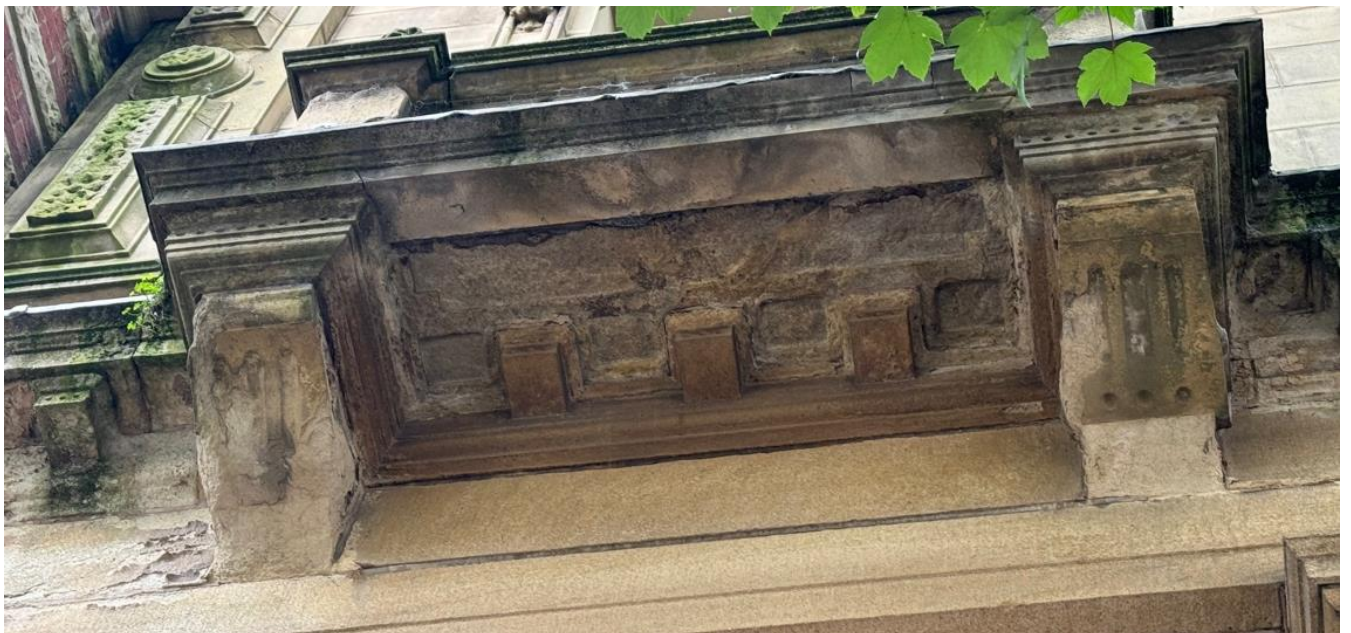
Photo 3: Decayed balcony Bank Street
