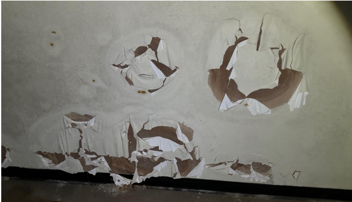
Photo 43: Ground floor rear, damp walls
