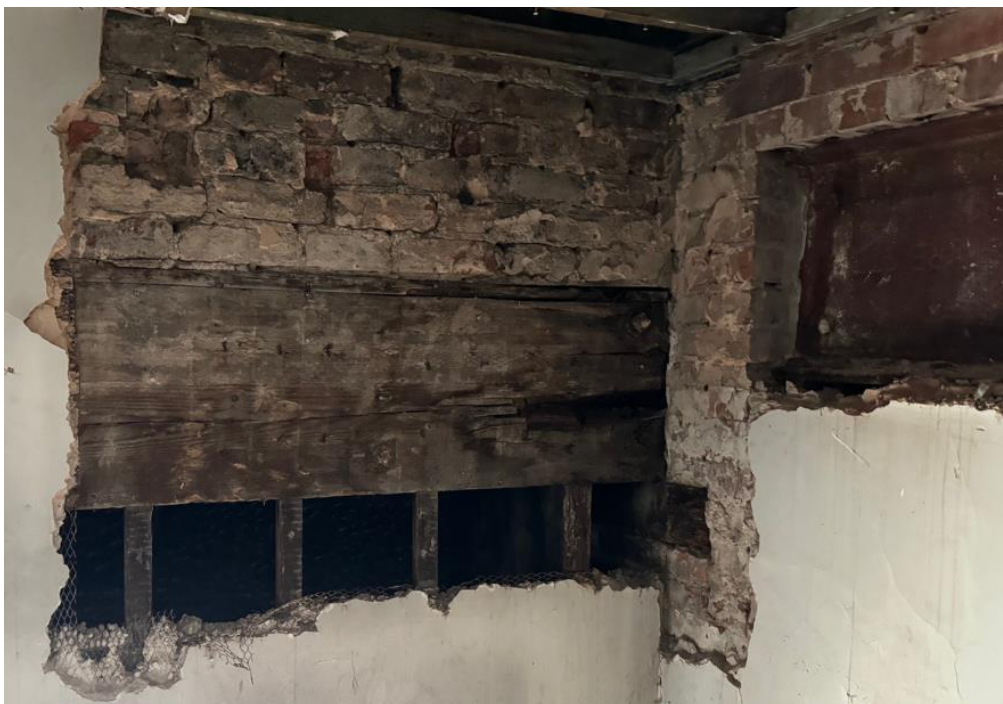
Photo 21: Ground floor mezzanine, room 1 rotten lintel and exposed steelwork
