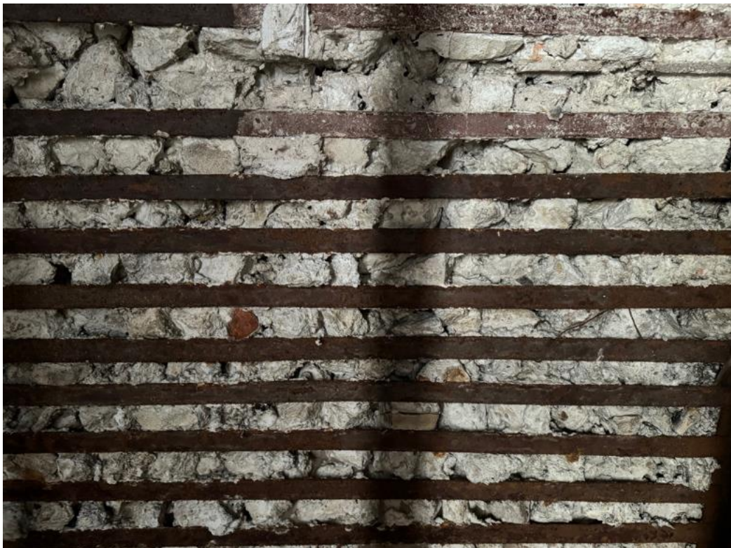
Photo 23: Ground floor mezzanine, hallway corrugated reinforcement and failed slab (from above)
