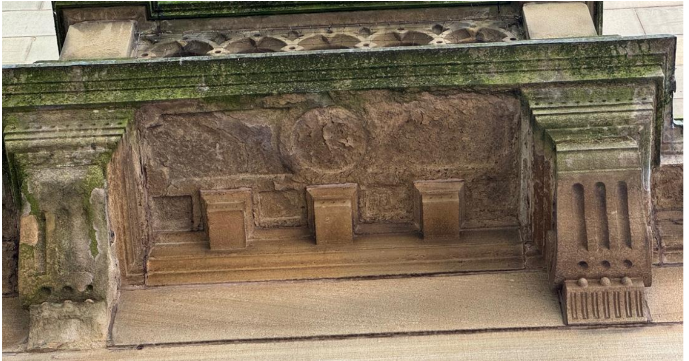
Photo 2: Decayed Balcony, Bank Street
