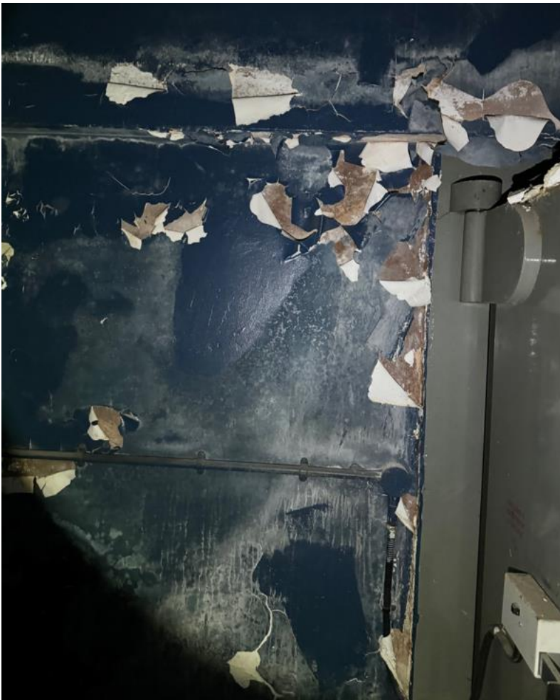
Photo 38: Ground floor rear, damp and peeling paint
