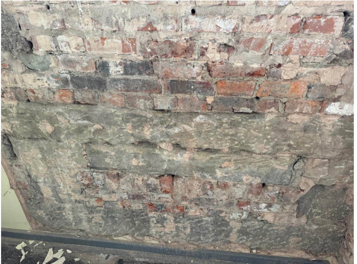
Photo 6: Damaged masonry and stone plinth First floor Stairwell
