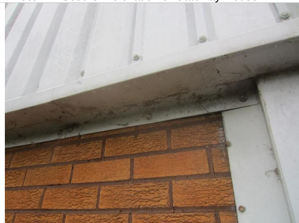
Photo 16: Southern elevation of Gateway House showing sealed fabrication
