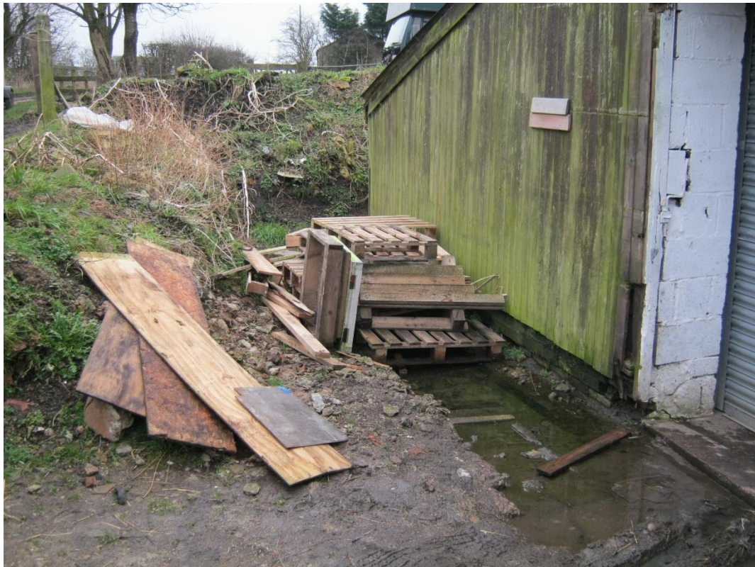
Photo 3: Wooden pallets and standing surface water in front of the entrance to the barn.
