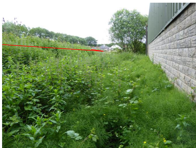
Tall ruderal vegetation off the buildings NW elevation.
