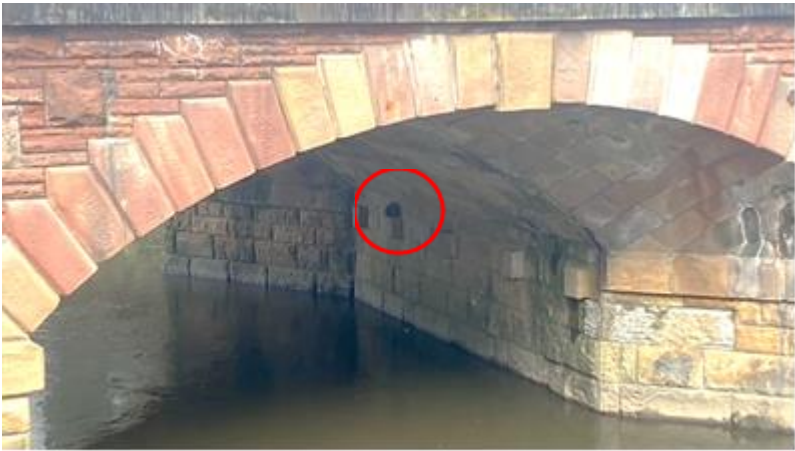
Photo 3.6: Bird Nest – Underneath Arch, Viewed From Eastern Elevation
