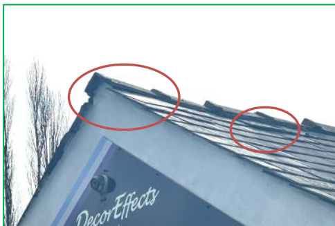
Showing crevices under ridge tiles and slates on the northeast and northwest elevation of the single-storey extension.
