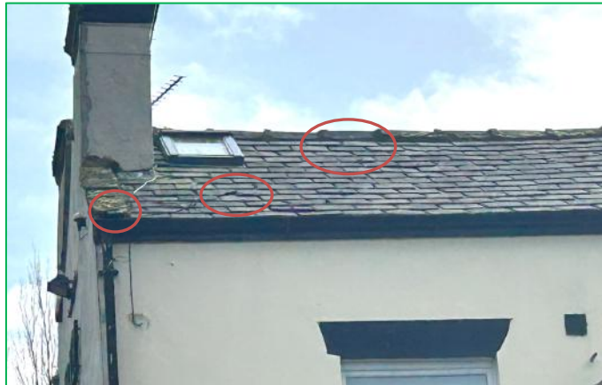
Showing crevices under slates and ridge tile on the northwest elevation of the main body of the building.
