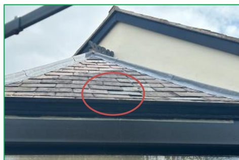
Showing crevices under slates on the northwest elevation of the conservatory.
