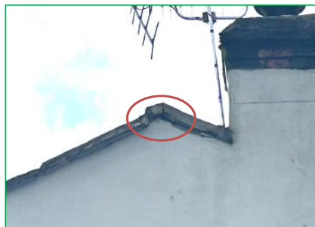
Showing a crack in the gable in the northwest elevation of the main body of the building.
