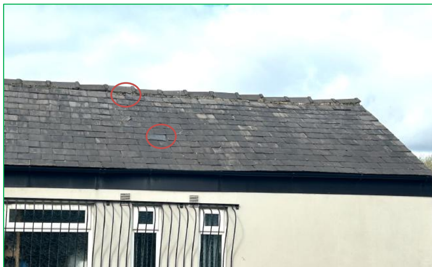
Showing crevices under slates and ridge tile on the southeast elevation of the single-storey extension.
