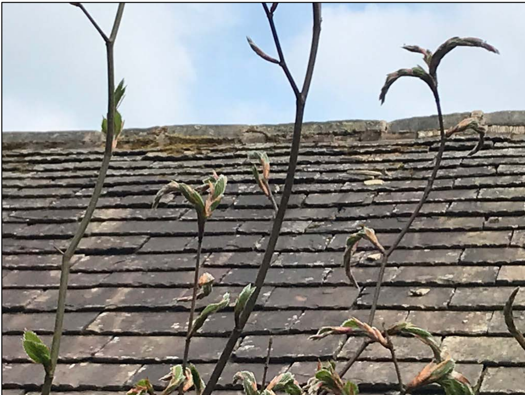
5.5 Damaged pointing and moss growth to stone ridge capping.
