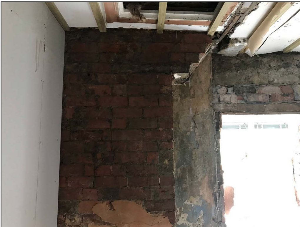
5.1 Saturated brickwork beneath southern chimney caused by defective flashing.
