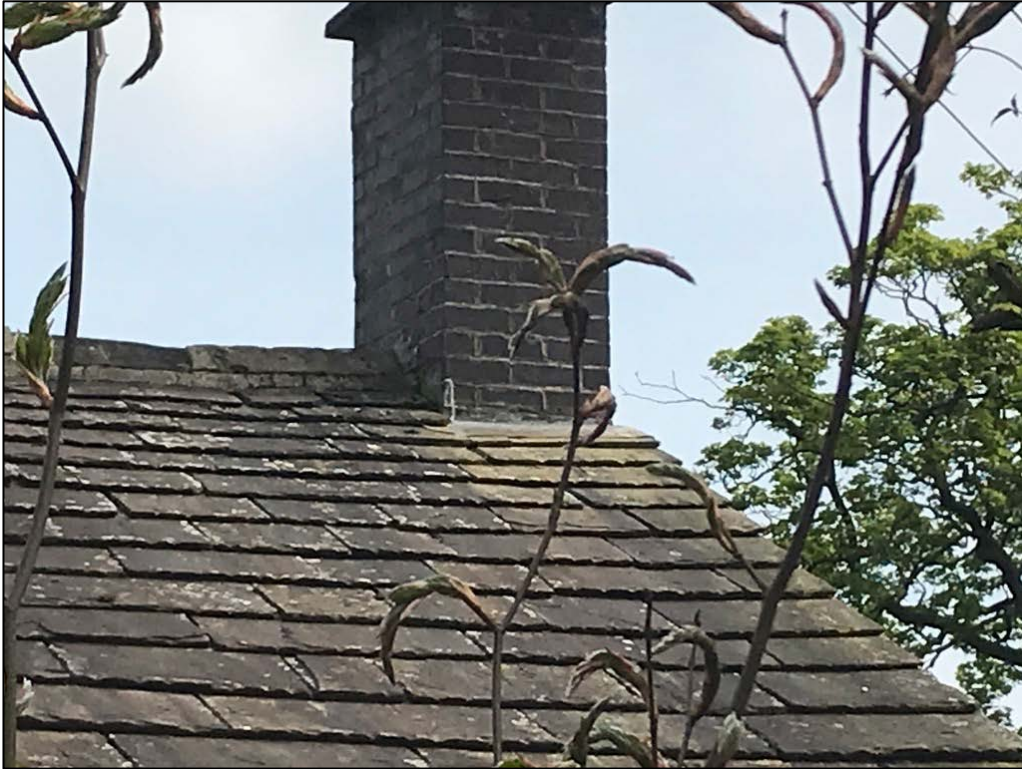
5.2 Evidence of defective flashing to exterior of southern chimney stack.
