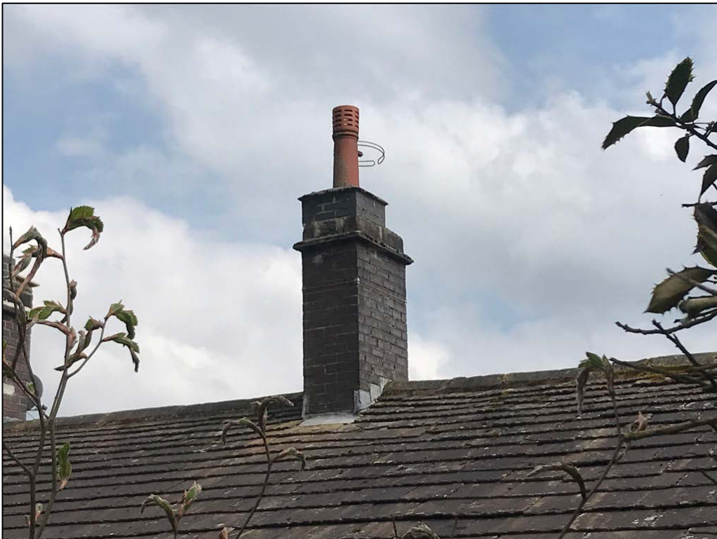
5.3 Uncapped chimney pot and moss growth visible to central chimney stack.
