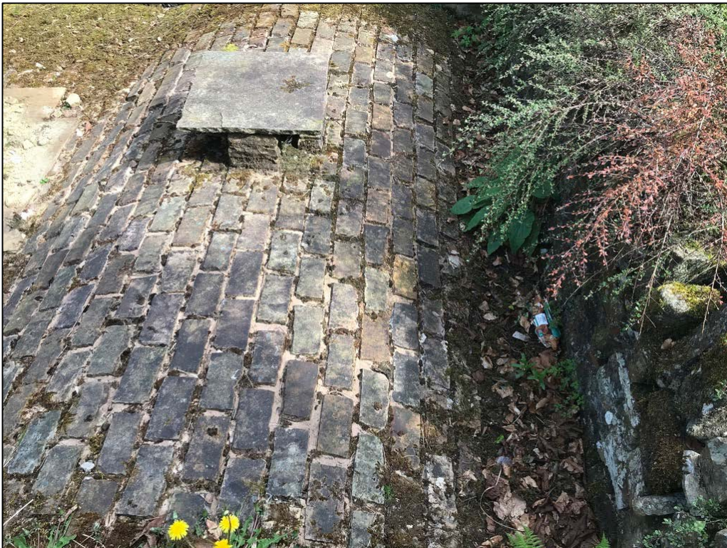
5.13 Recessed pointing style to modern stone setts allows water to pool between setts.
