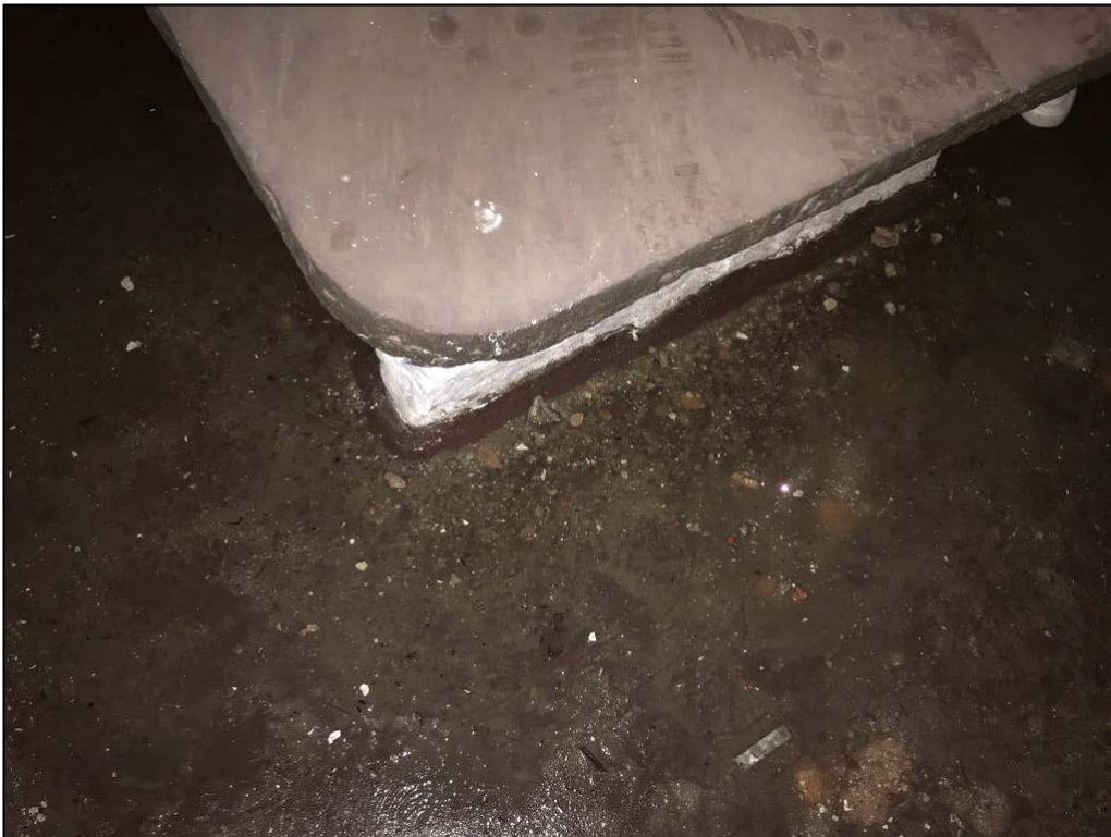
5.11 Significant water ingress to cellar area with standing water visible at ground level.
