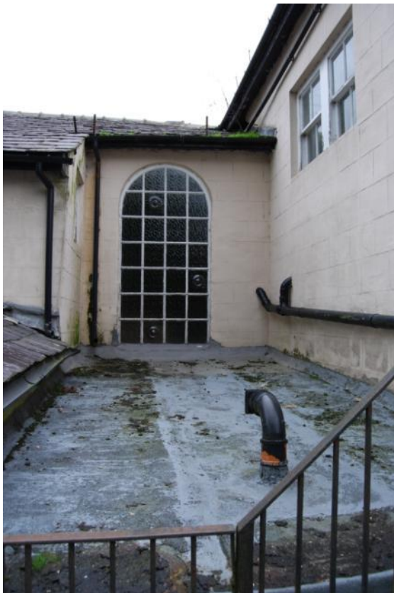
Figure 9. Flat roof over store (looking east) in a failing condition. Built in to the original staircase window.
