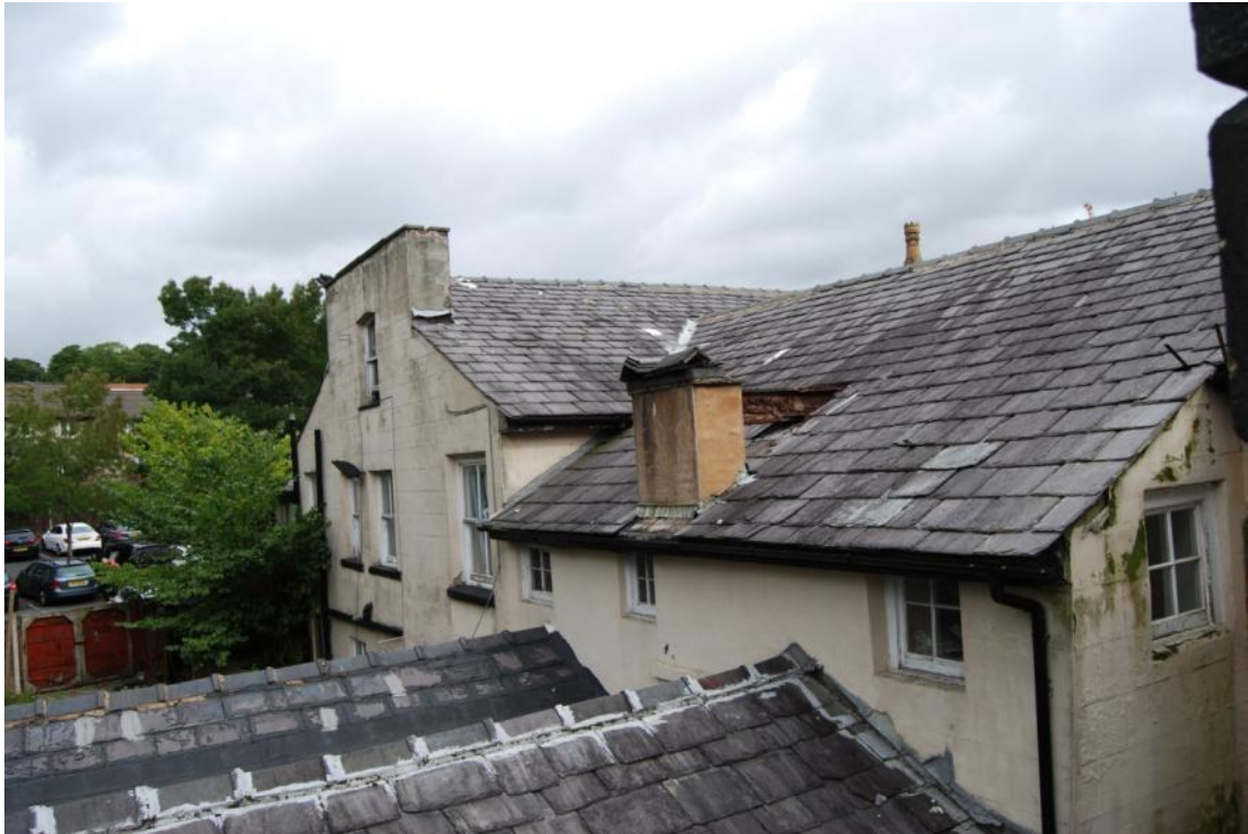
Figure 8. Existing roofs over kitchen in poor condition and the main roof chimneys and elevations in need of repair and restoration. Windows in poor condition.
