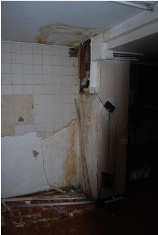
Figure 28. Upper ground floor annex adjacent kitchen with damp penetration and failing walls and ceiling.
