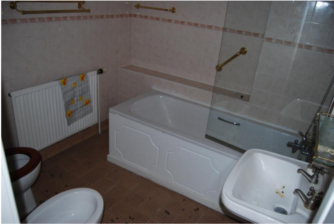
Figure 33. First floor typical en-suite with failing tiled floor finishes, dated wall finishes and dated sanitary ware.
