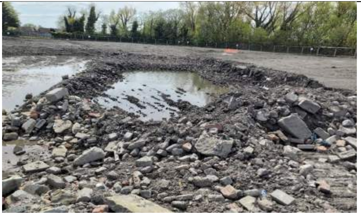
Photograph 12: Standing water and oversize material of temporary road in the southwest.
