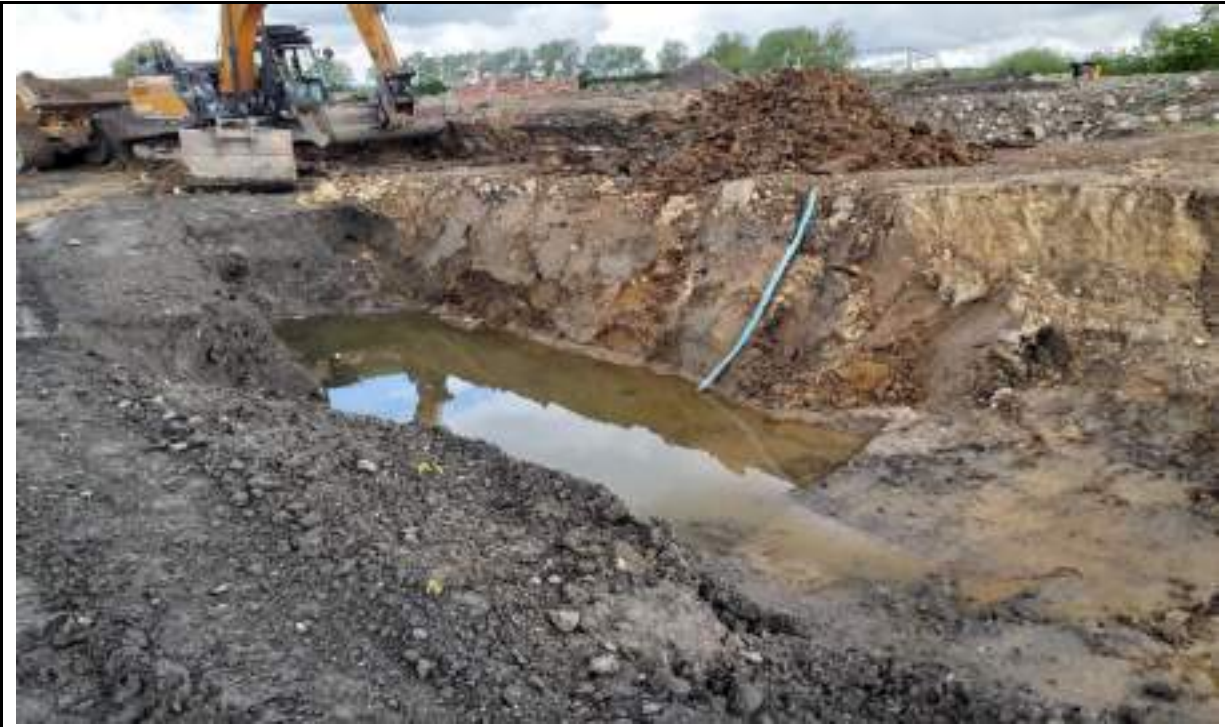
Photograph 3: Standing water next to Glacial Till excavation in the east.
