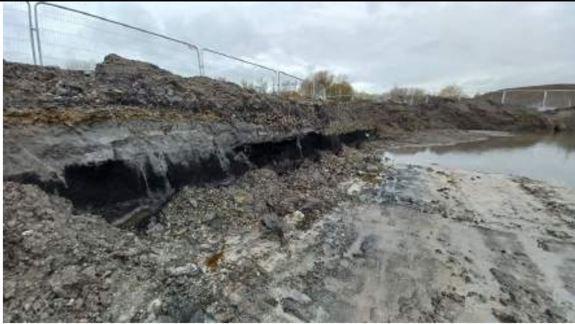
Photograph 5: Some steep excavations noted. Recommend reducing and battering back prior to winter shutdown
