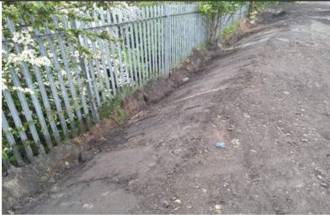
Photograph 9: Slope of battered fill next to slope of the adjacent land in the northwest seems quit deep and unsafe.
