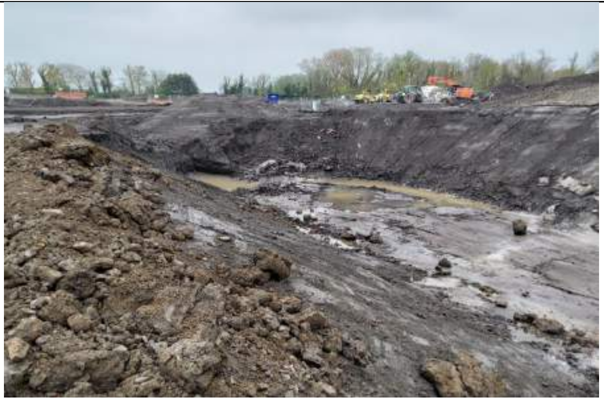
Photograph 6: Standing water in excavation in the centre east.
