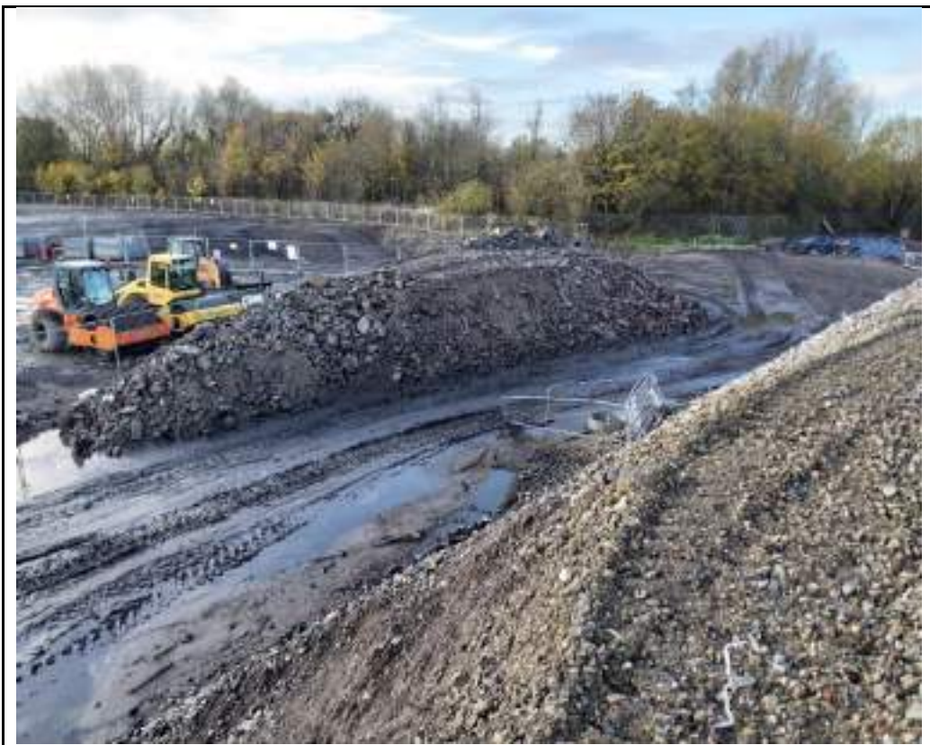
Photograph 10: Stockpile of oversized materials and concrete in the northwest.
