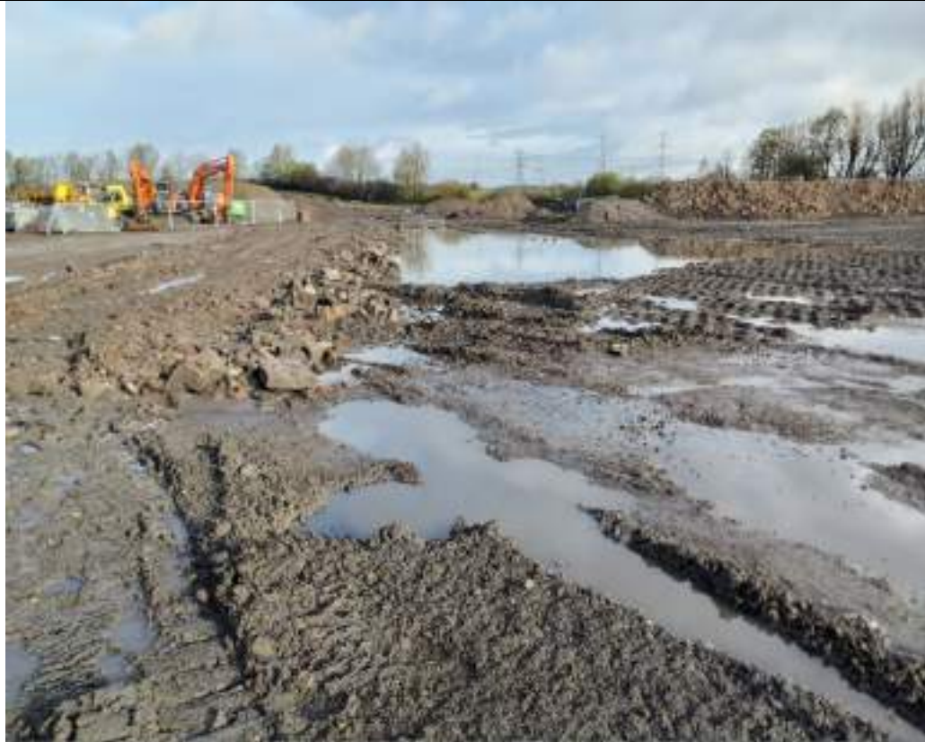
Photograph 15: Standing water in southeastern part of the site.
