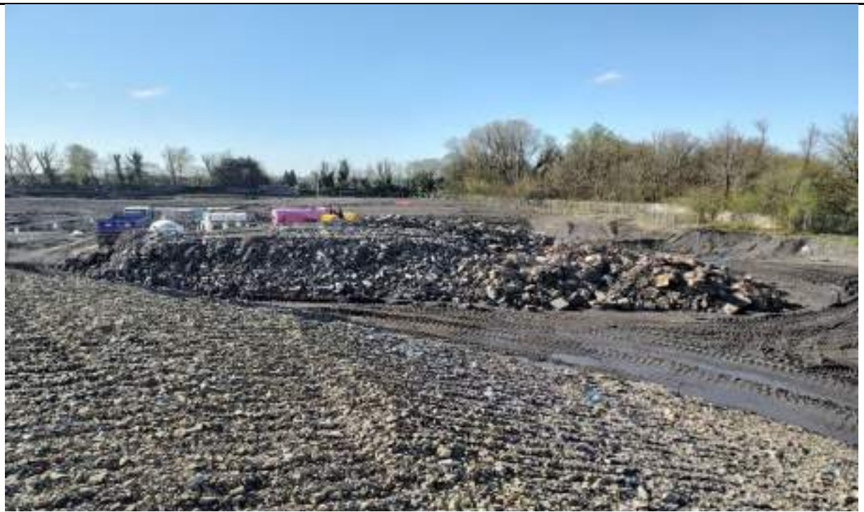
Photograph 14: Stockpile of oversize and deleterious material in the center west.
