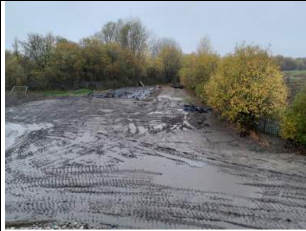
Photograph 11: Stockpile of TPH contaminated materials in the west.
