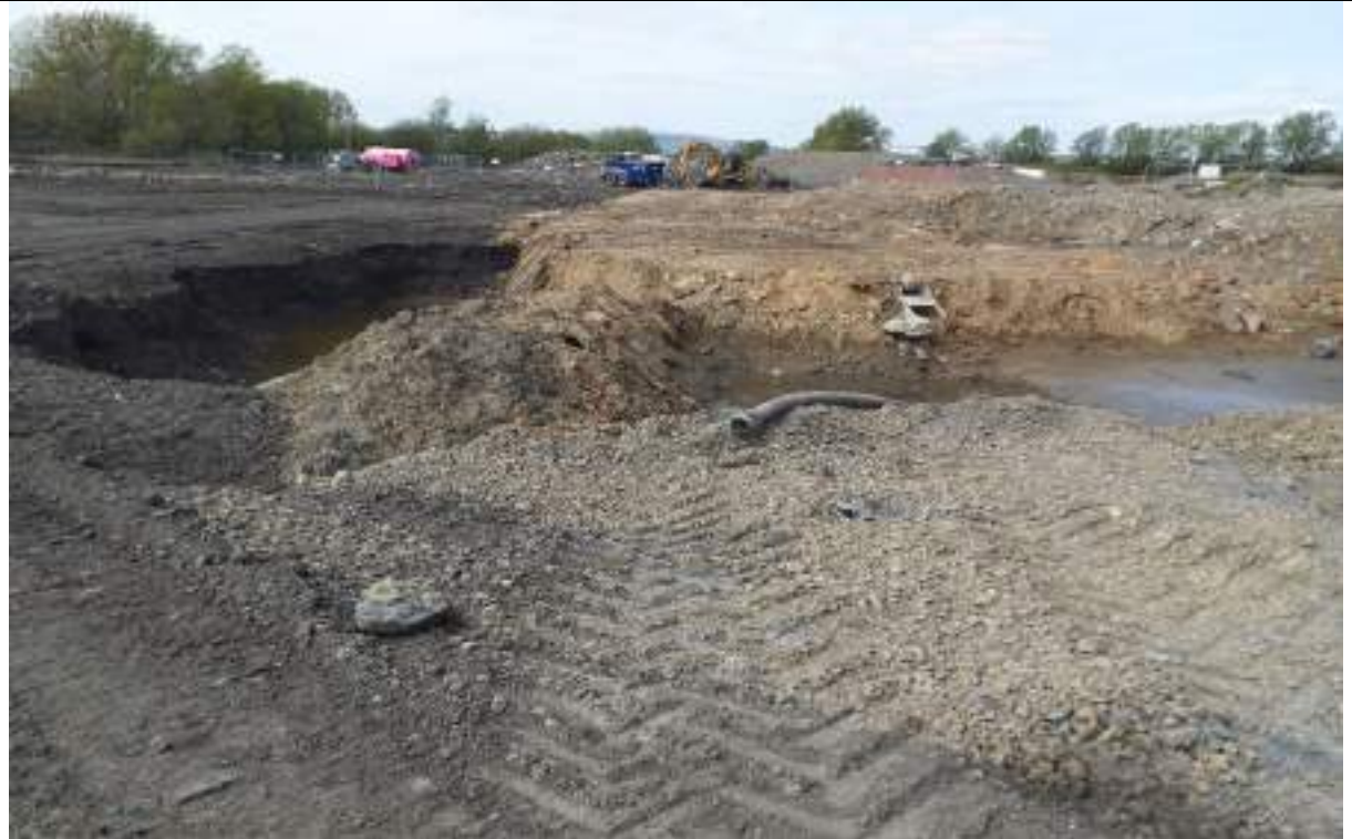
Photograph 15: Standing water next to the unsuitable Glacial Till material stockpile in the southeast.
