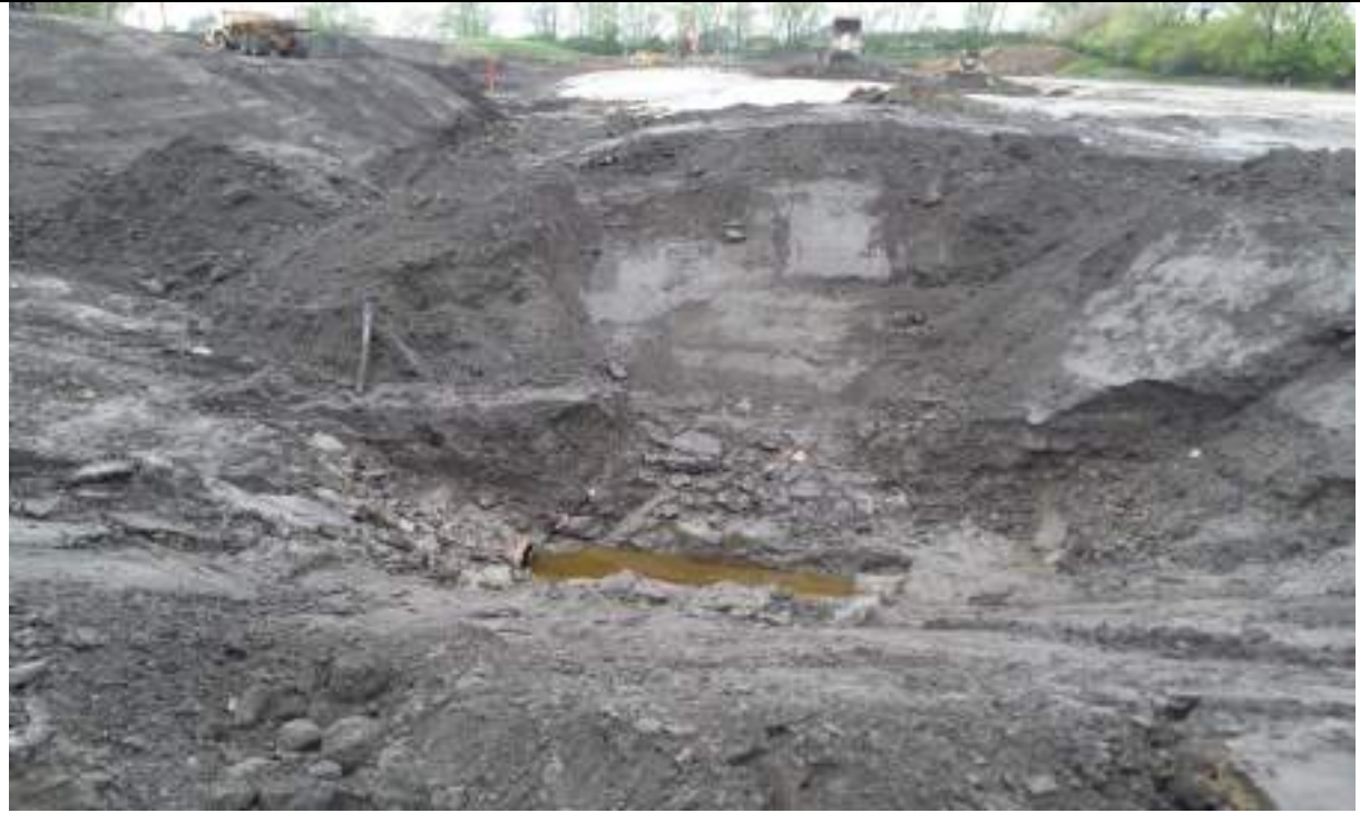
Photograph 5: Damaged drainage pipe in excavation in the centre east.
