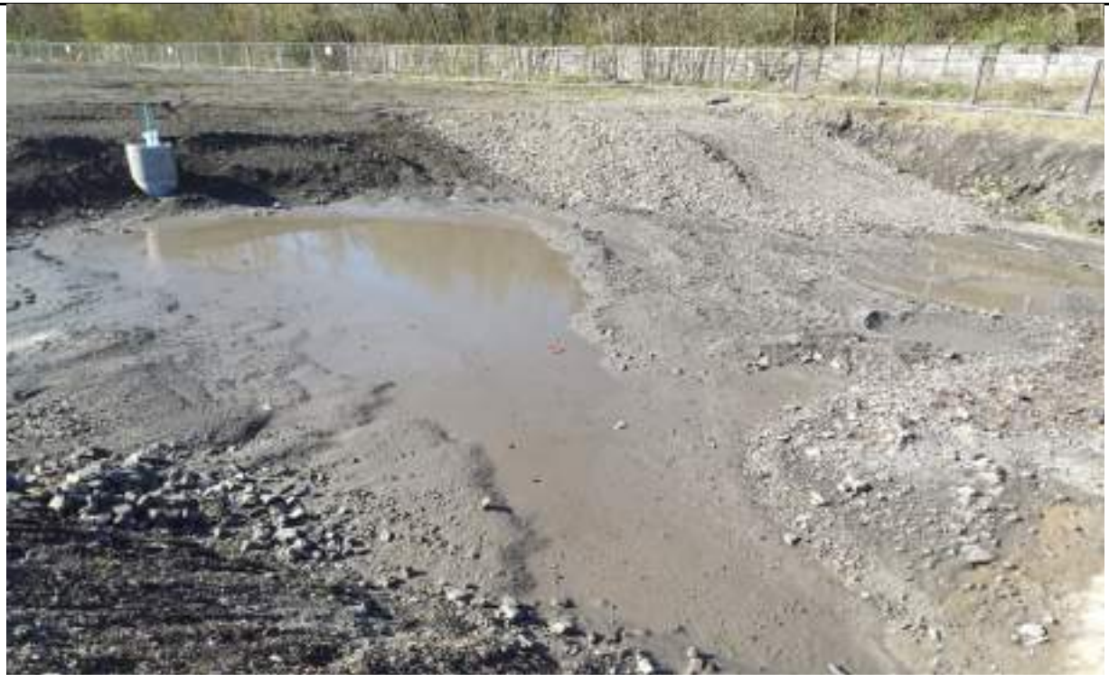
Photograph 10: Standing water in excavation in the west. Water to be removed before placing fill.
