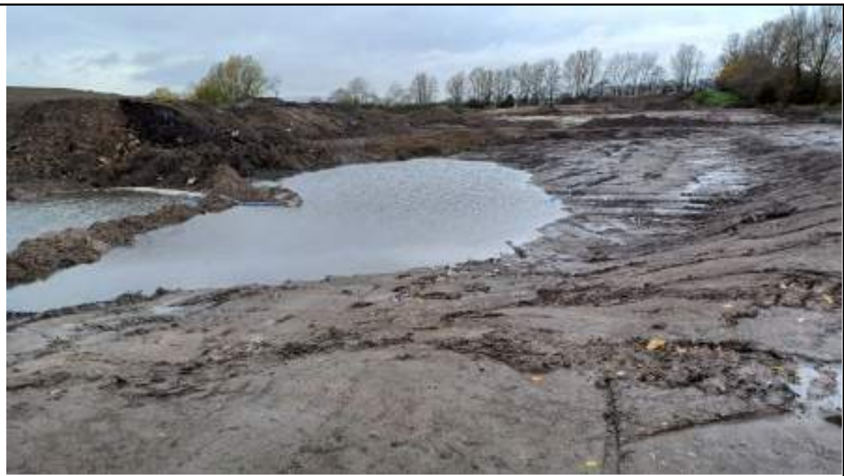
Photograph 4: Fill proof rolled to shed water. Significant standing water
