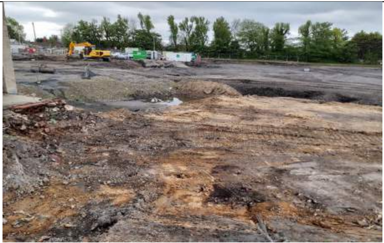
Photograph 2: Standing water in the southeast.
