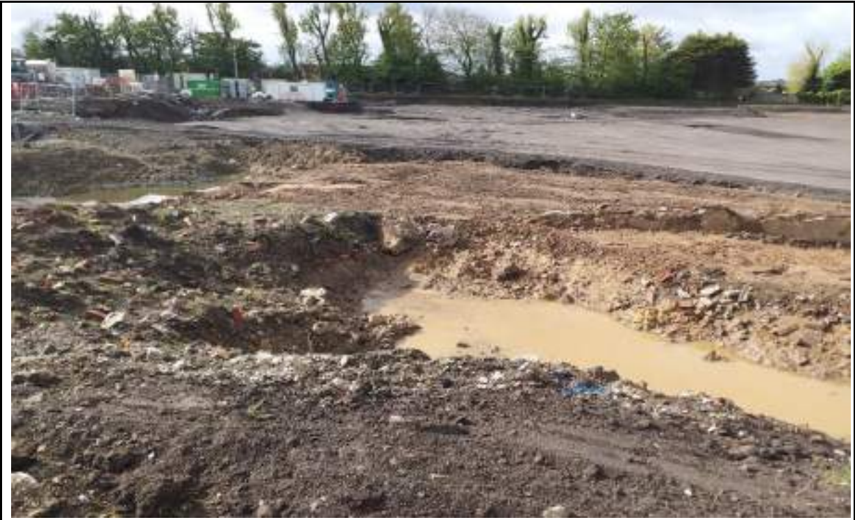
Photograph 3: Standing water in the southeast.
