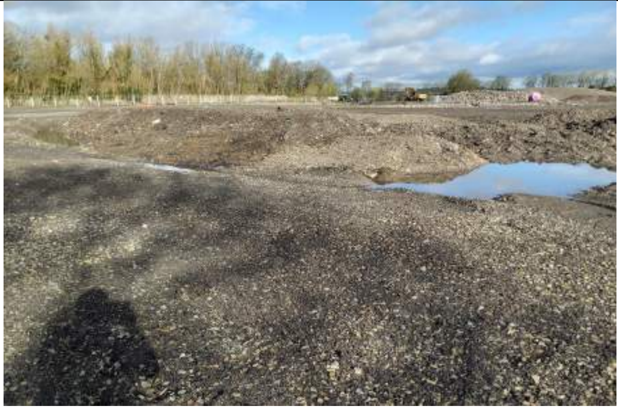
Photograph 11: Standing water in the south.
