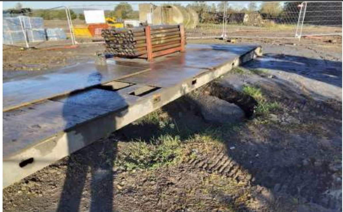
Photograph 1: Settlement of shaft no.7 original backfill.
