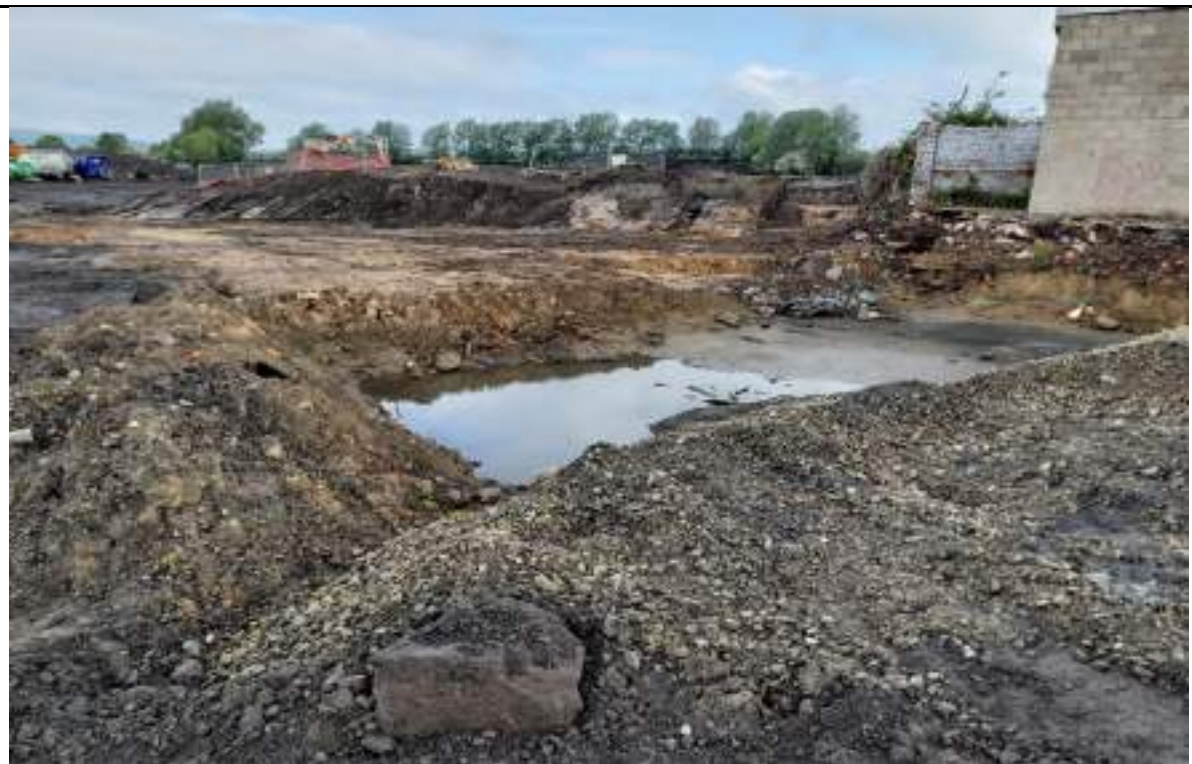
Photograph 14: Standing water in the southeast.
