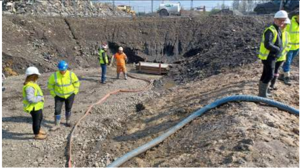
Photograph 9: Over-steepened slopes around abstraction borehole to be re-profiled
