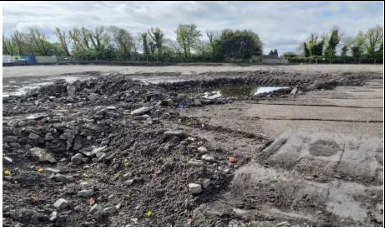
Photograph 11: Standing water adjacent to temporary road constructed with oversize material during the wet season.
