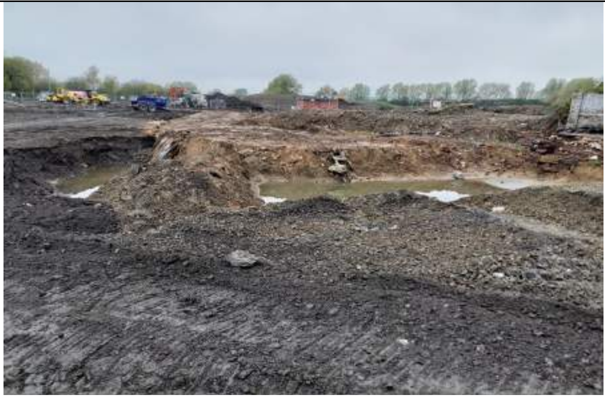
Photograph 1: Standing water in the southeast.
