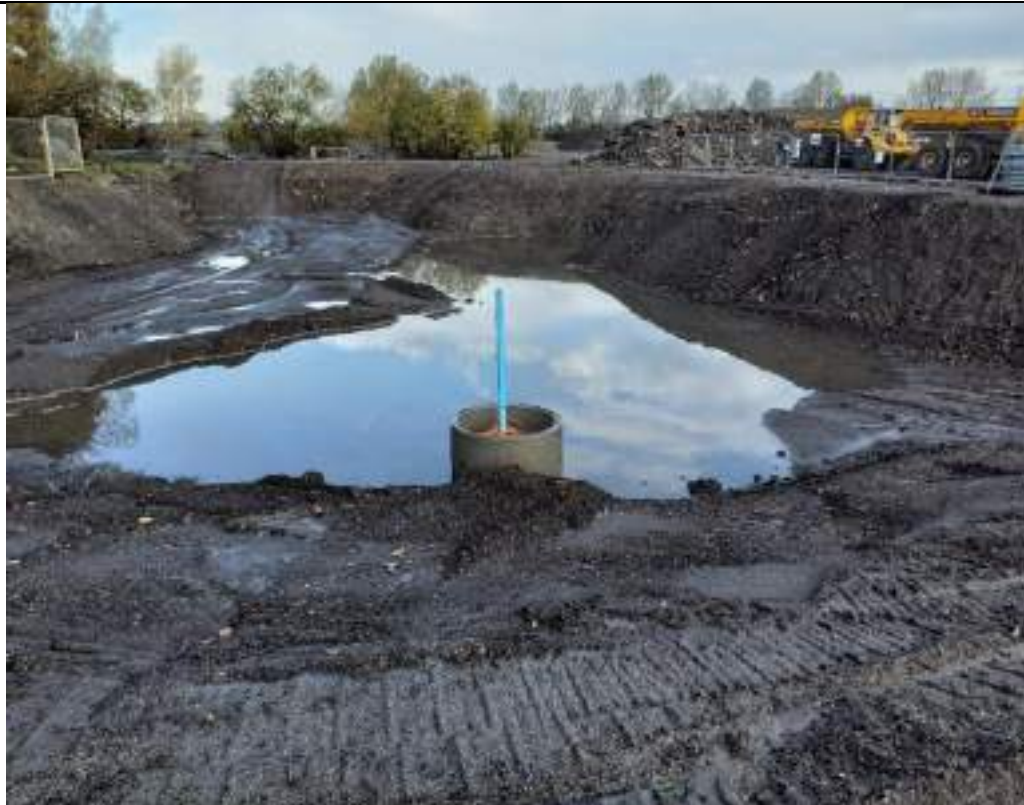
Photograph 16: Standing water in western boundary of the site.
