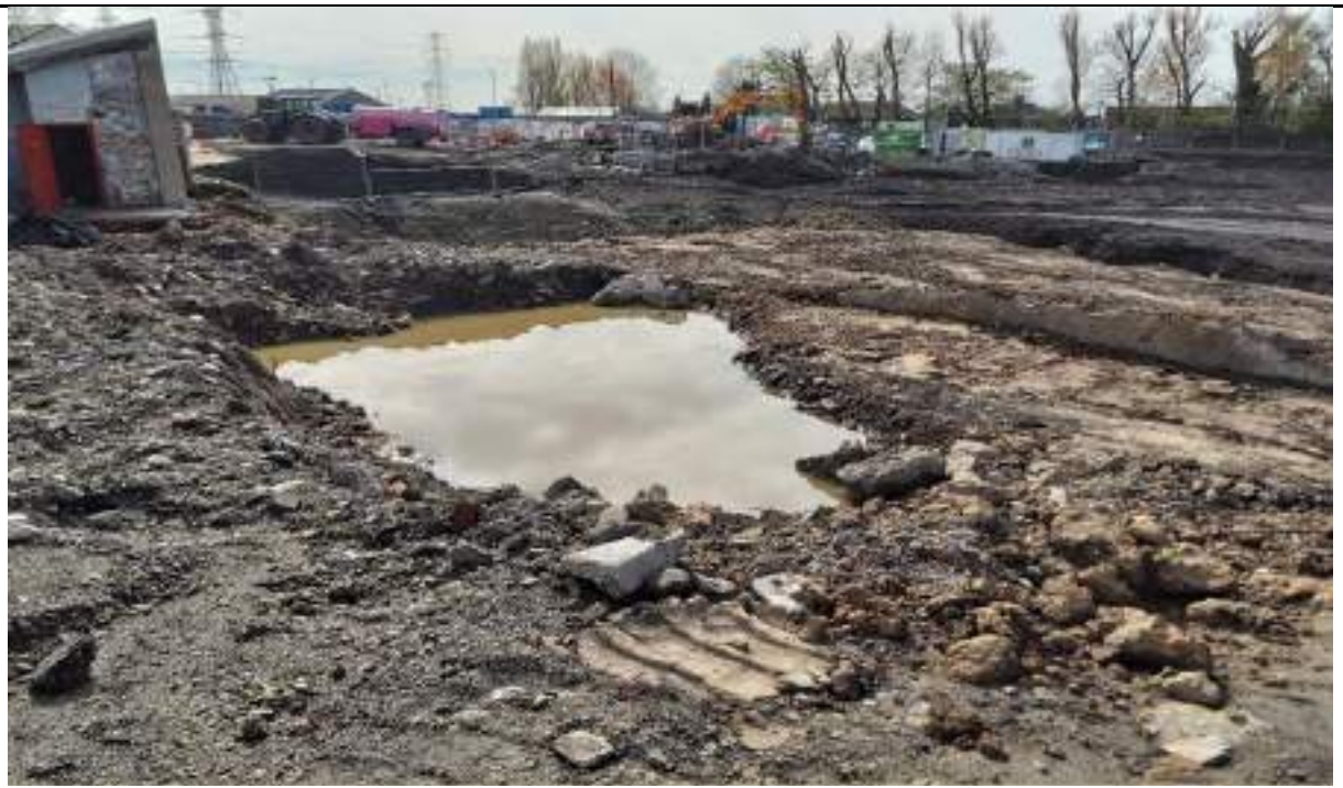
Photograph 14: Standing water in the southeast.
