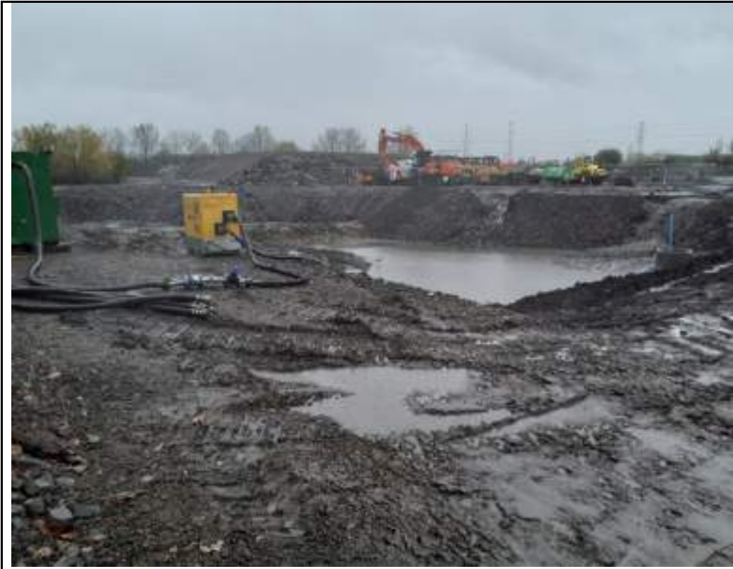
Photograph 15: Standing water and dewatering tools in the west.
