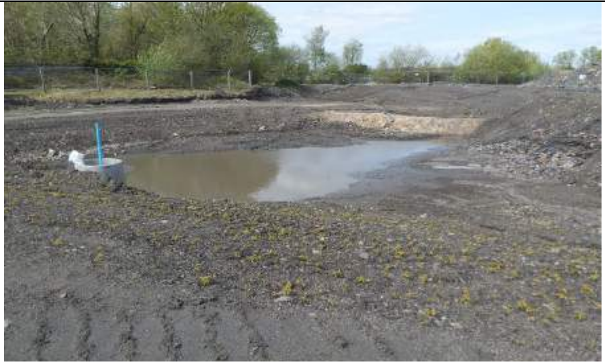
Photograph 13: Standing water in the western boundary.
