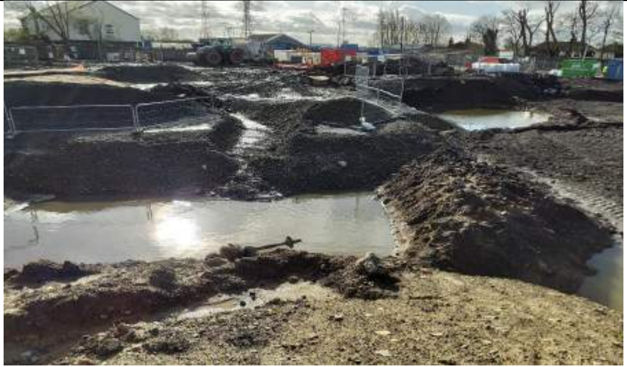
Photograph 15: Standing water in the southeast.
