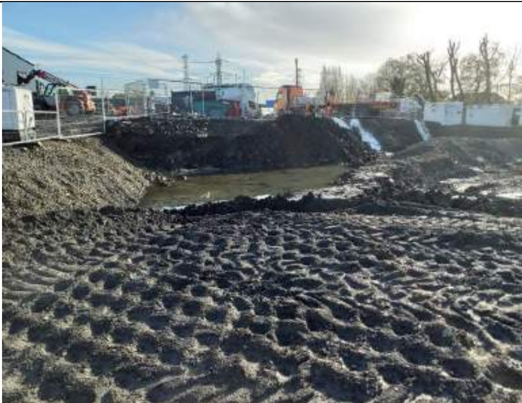
Photograph 22: Standing water in the southwest of shaft treatment platform.
