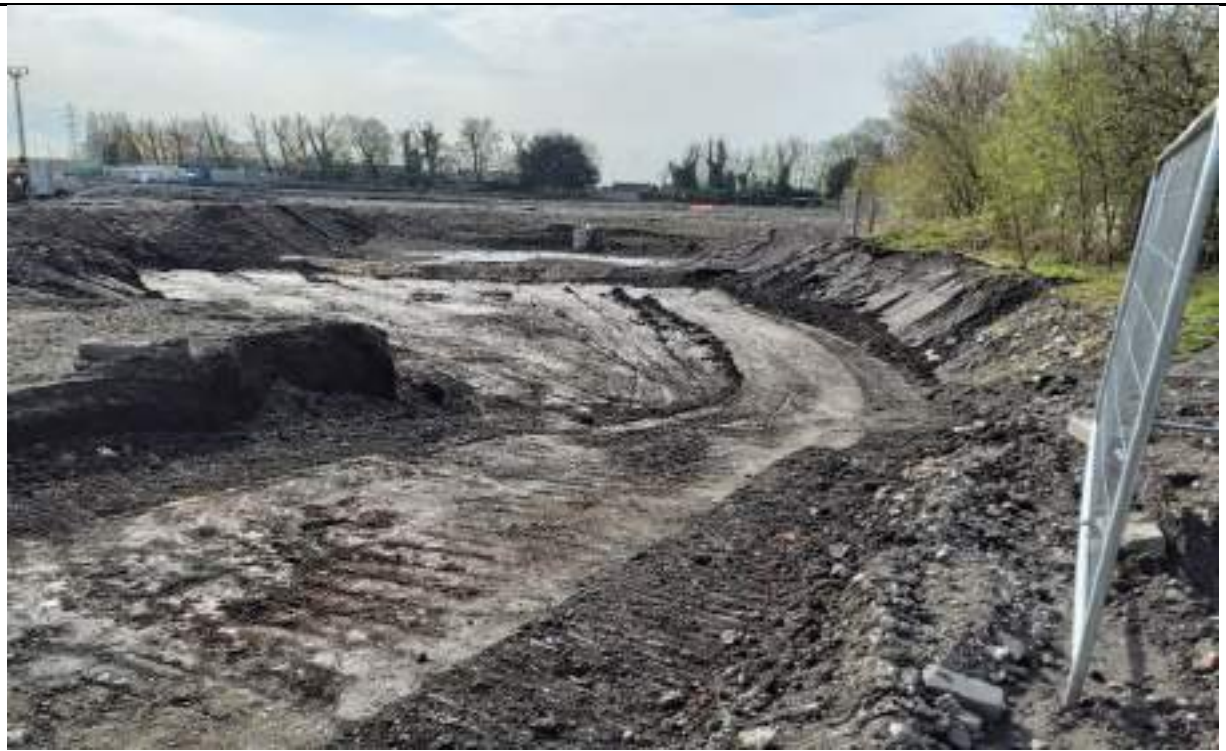
Photograph 12: Standing water and placed fill in the western boundary. Fill material is from hotspot 7 stockpile in the west.
