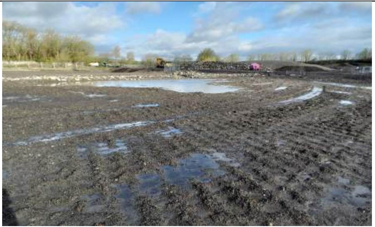
Photograph 12: Standing water in the centre of the site.
