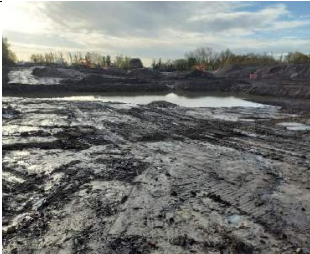
Photograph 8: Standing water in the northeast.
