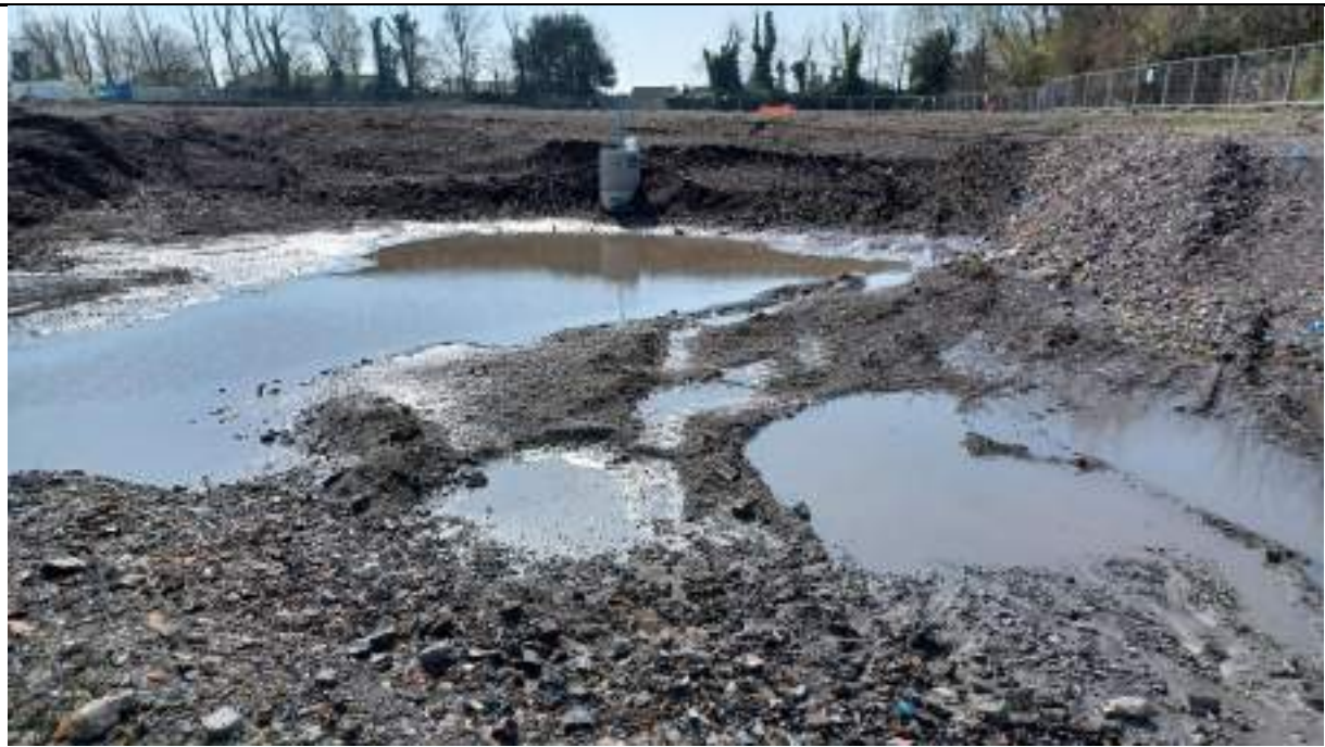
Photograph 8: Standing water in the centre east of the site. Water to be pumped out prior to filling
