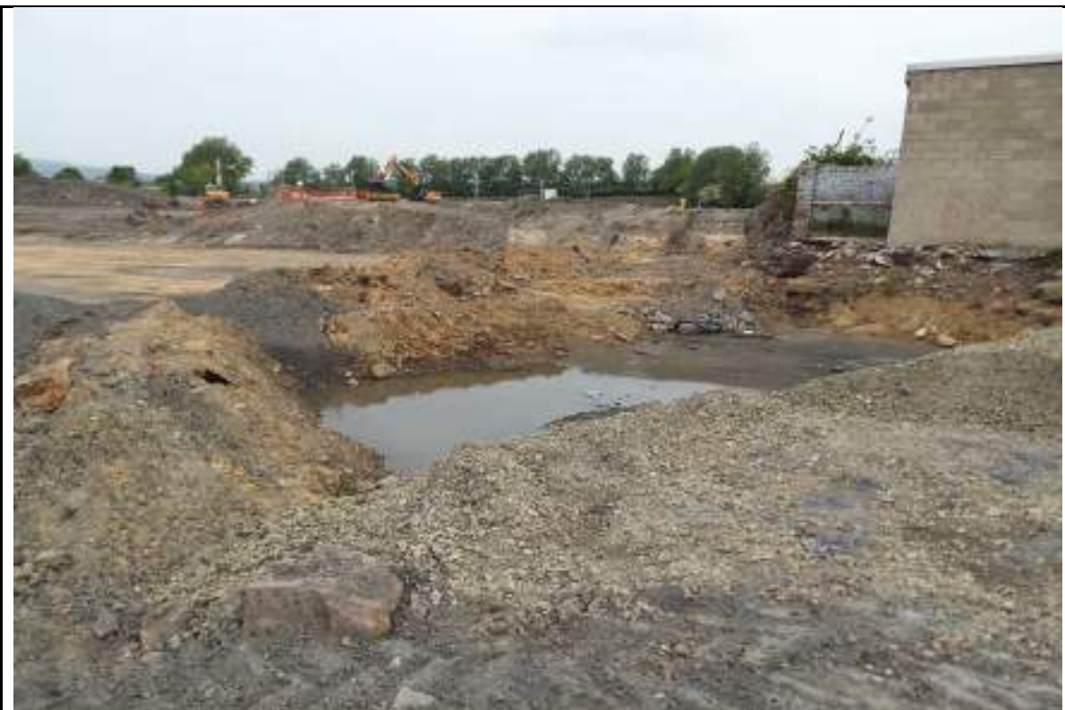
Photograph 8: Standing water in the southeast.
