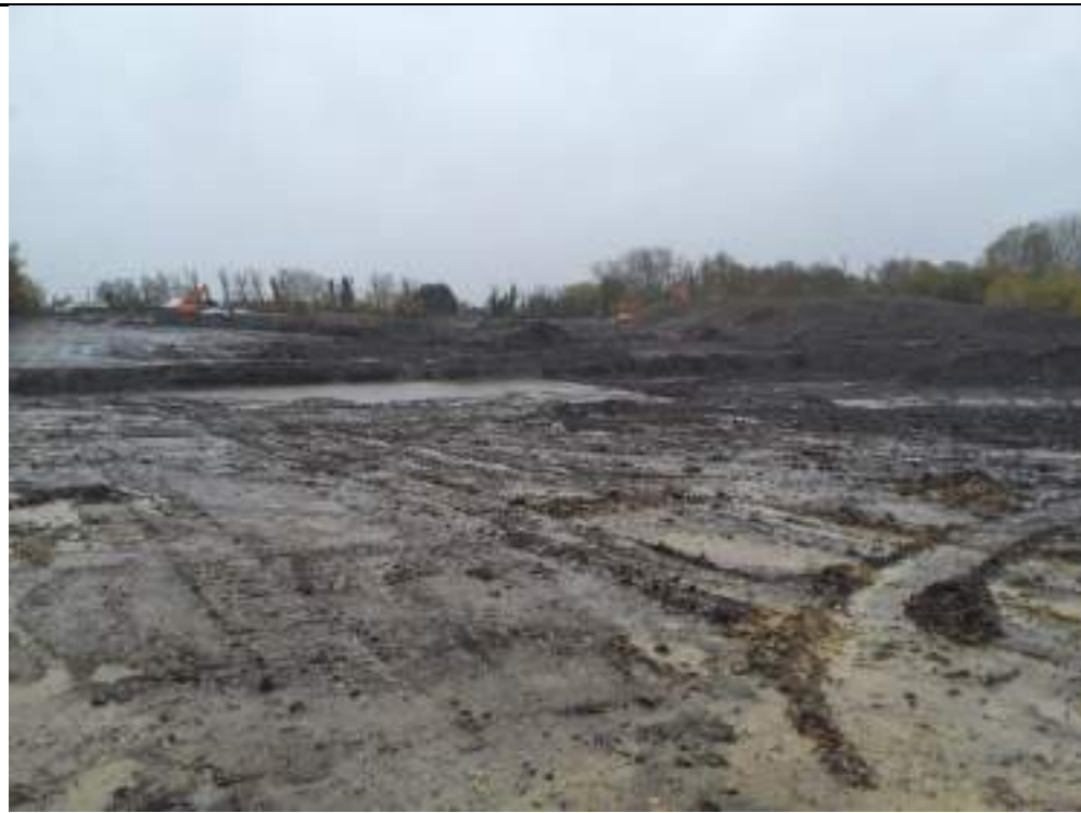
Photograph 6: Standing water in the northeast.
