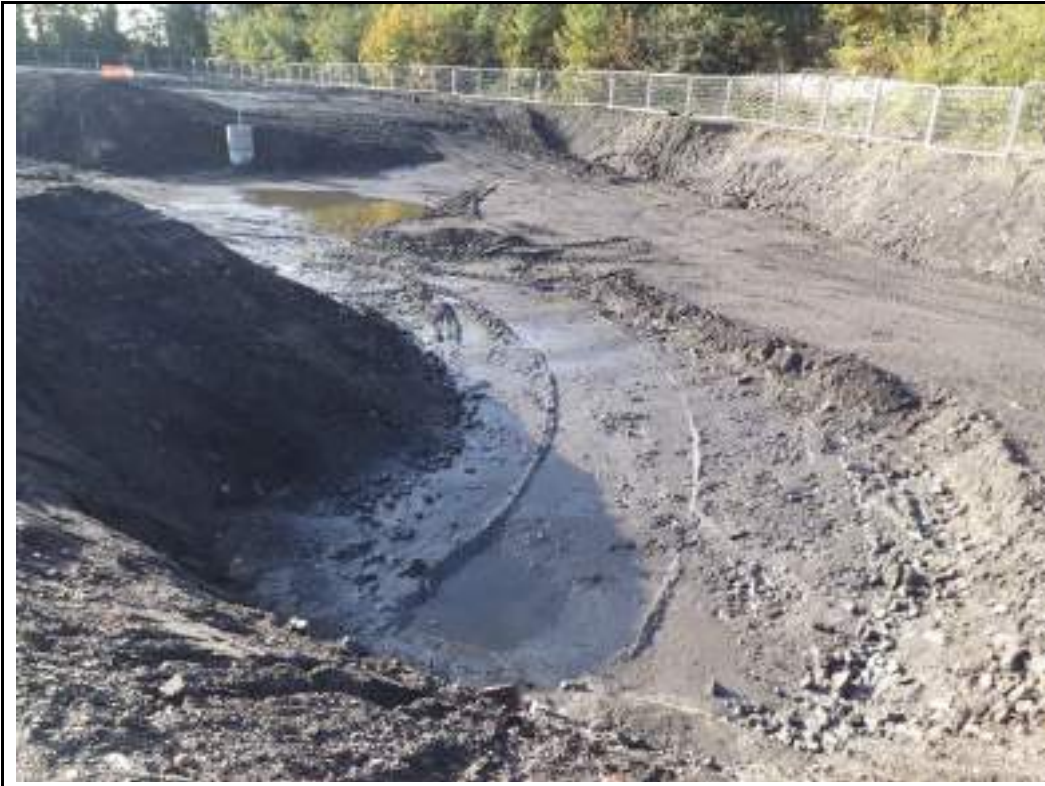
Photograph 17: Standing water in excavation in western boundary of the site.
