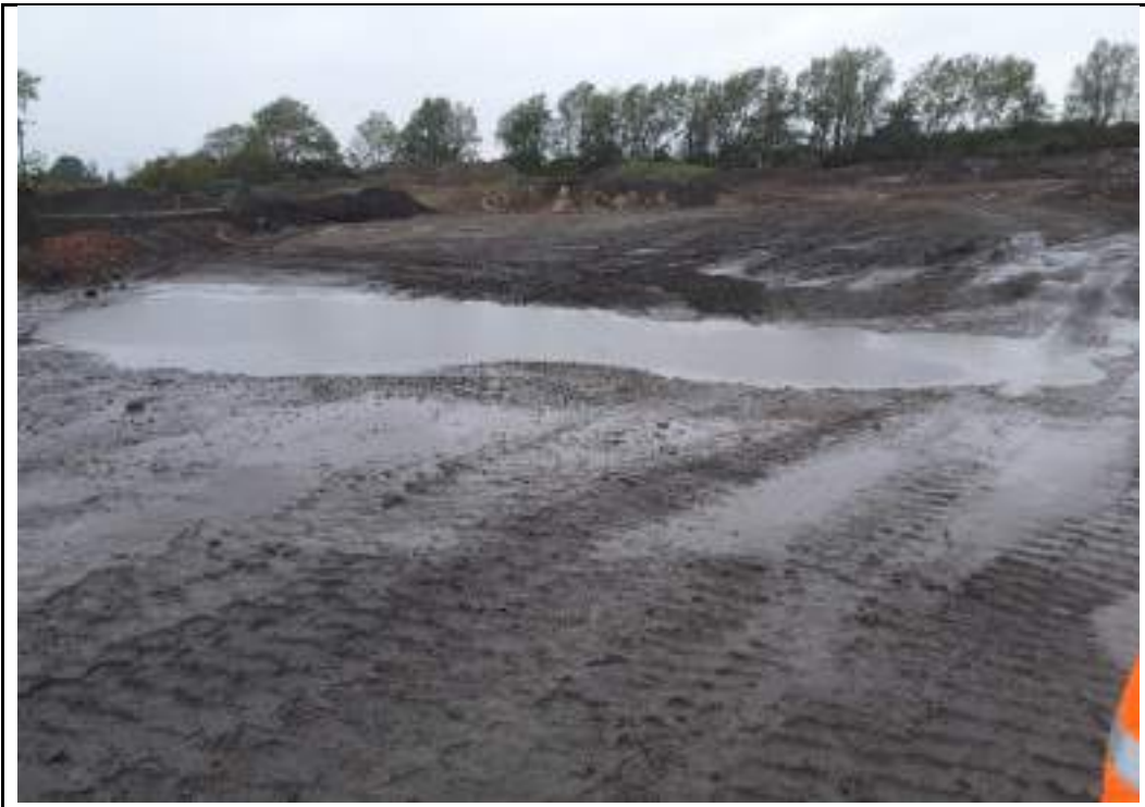
Photograph 14: Standing water in northern part of the site.
