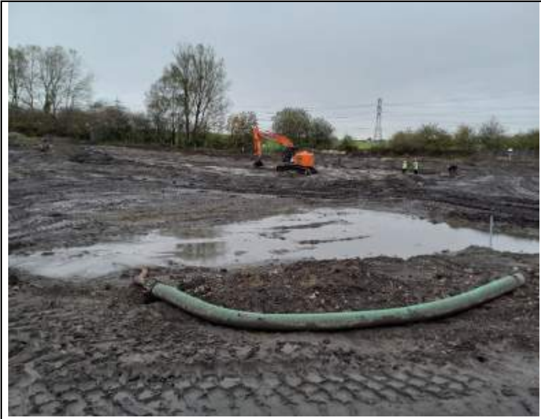
Photograph 9: Standing water in northern part of the site.
