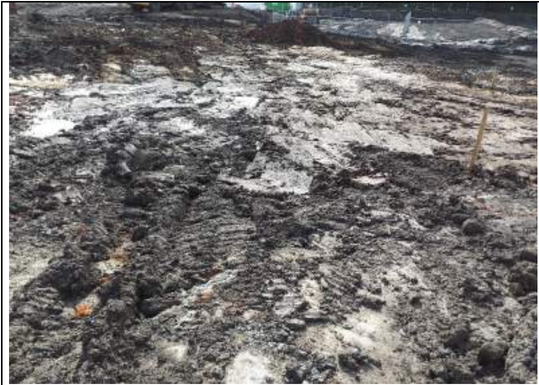
Photograph 169: Potentially TPH contaminated area in excavation in southeastern part of the site.
