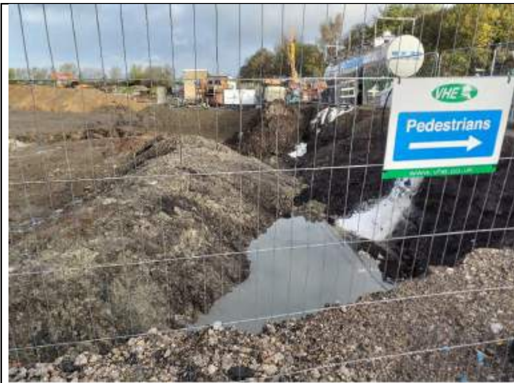
Photograph 12: Standing water and stockpile of unsuitable materials in southeastern part of the site.
