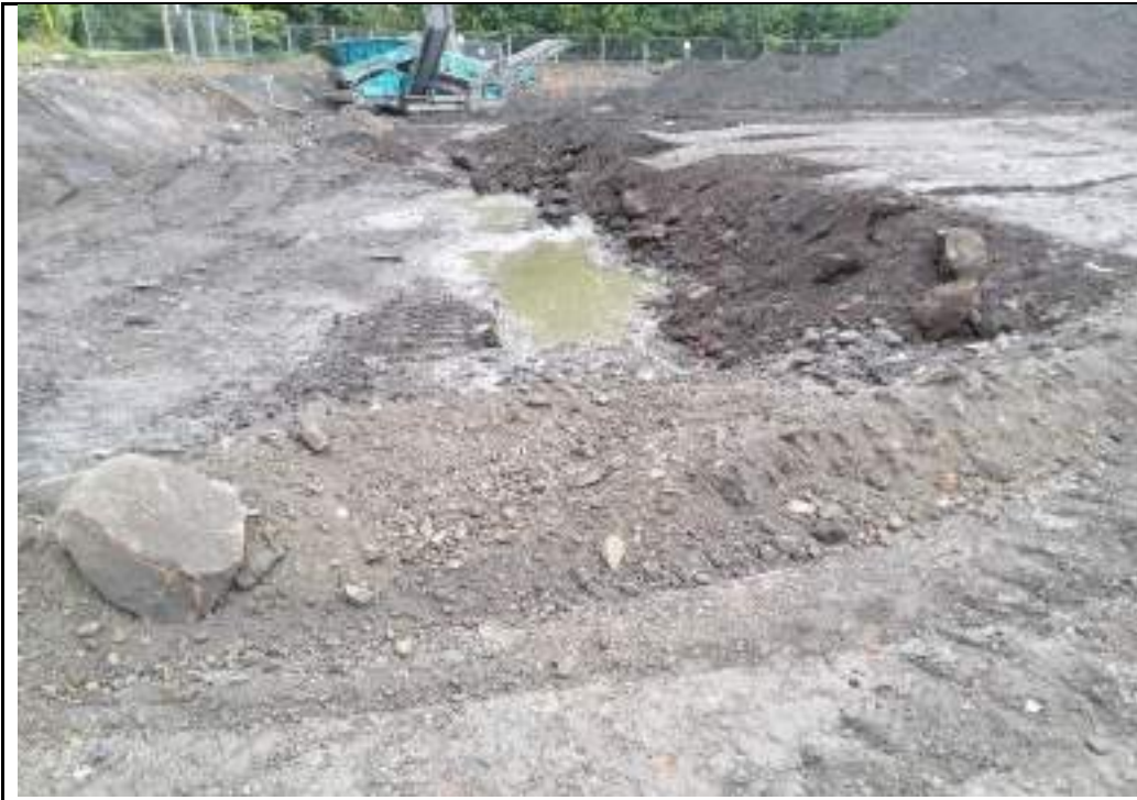
Photograph 25: Oversize in fill material in southern part of the site.
