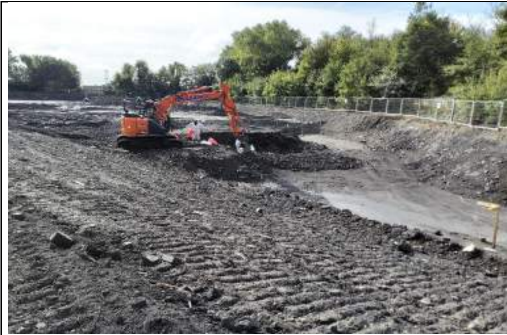
Photograph 23: Hand picking of asbestos from asbestos contaminated stockpile in western part of the site.
