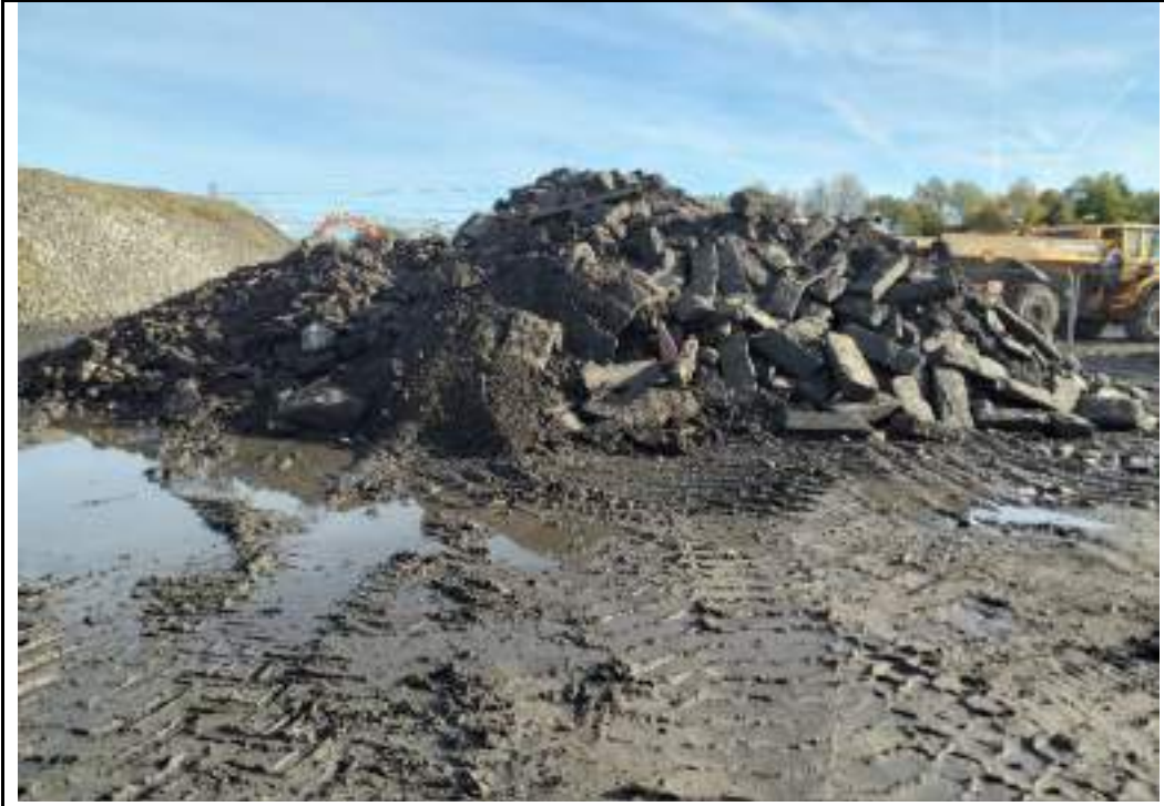
Photograph 93: Deleterious materials in stockpile of concrete and oversize materials in northwestern part of the site.
