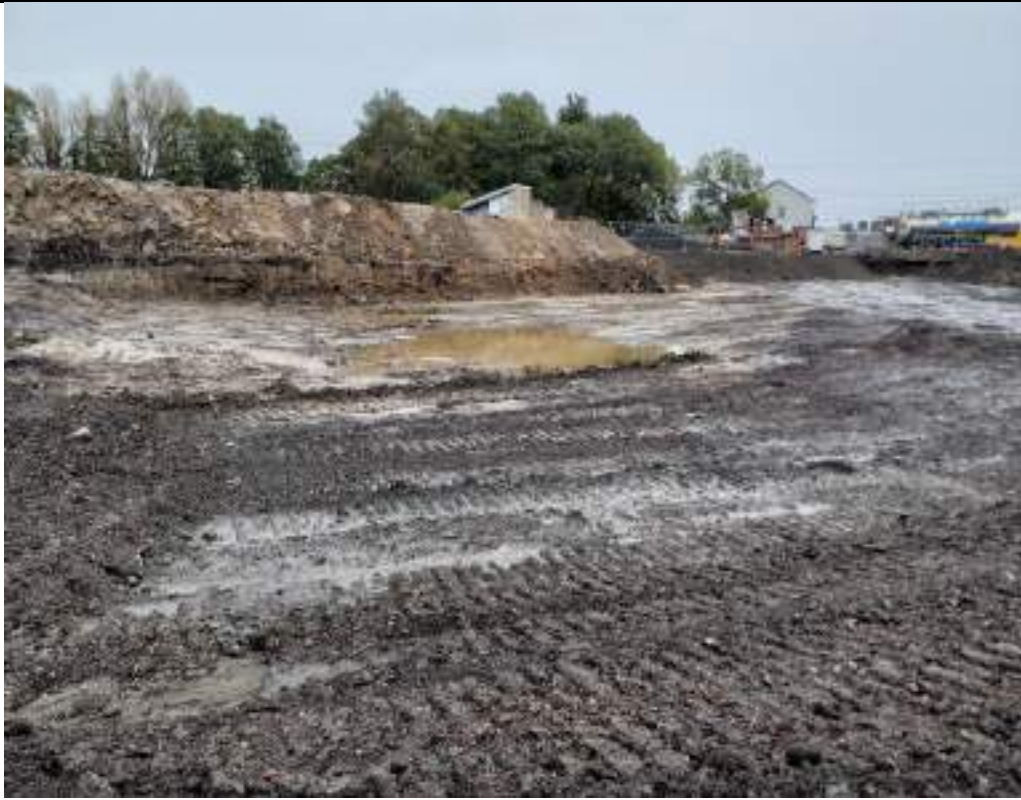
Photograph 19: Standing water in southeastern part of the site.
