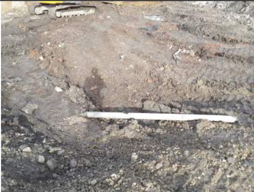
Photograph 18: Deleterious material in excavation in southeastern part of the site.
