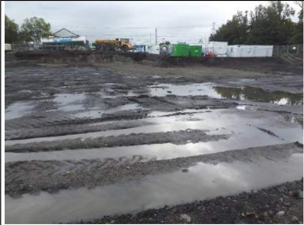
Photograph 93: Standing water and stockpile of soft spot material in southern part of the site.
