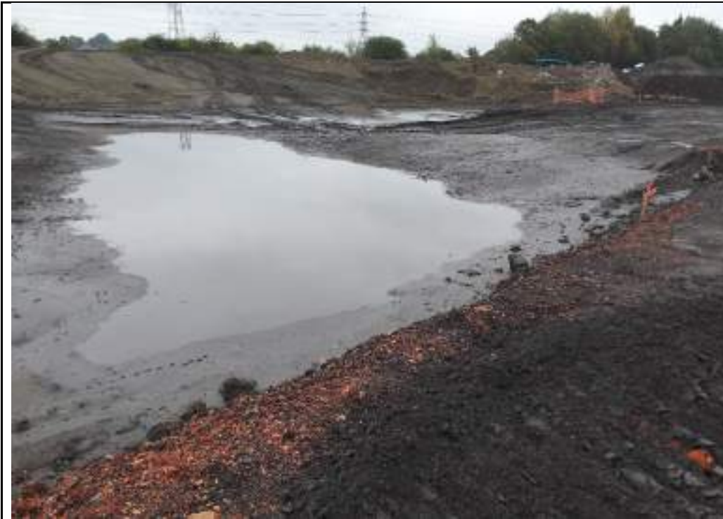
Photograph 125: Standing water in northern part of the site.
