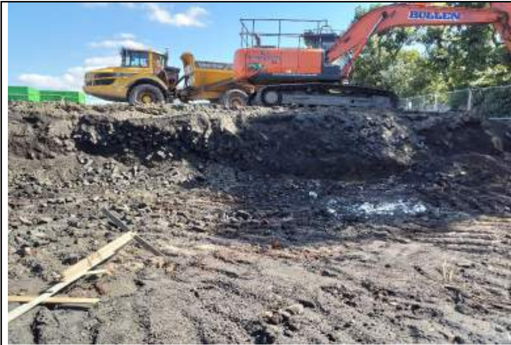
Photograph 189: High quantity of bricks and deleterious material in excavation in southern part of the site. Avoid transporting to fill areas
