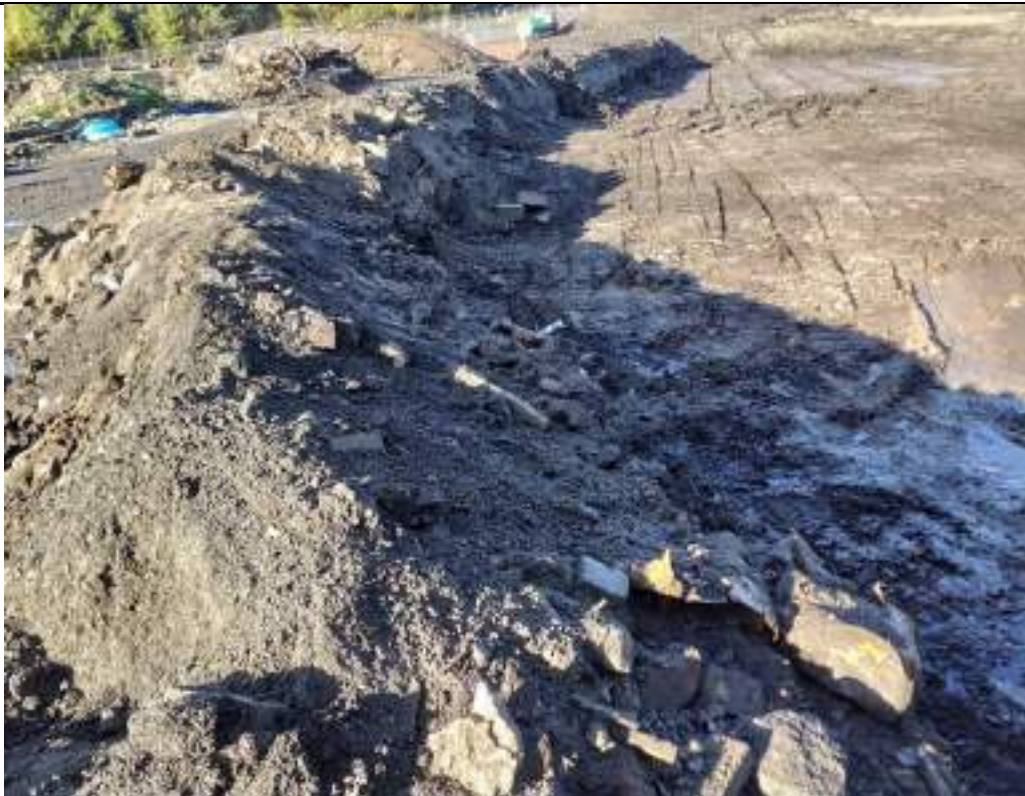
Photograph 20: Deleterious and oversized materials in excavation in eastern part of the site.
