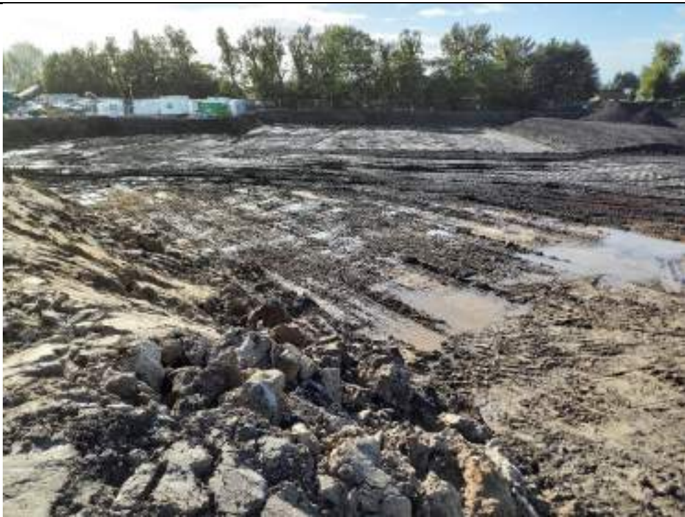
Photograph 6: Standing water in excavation in central part of the site.
