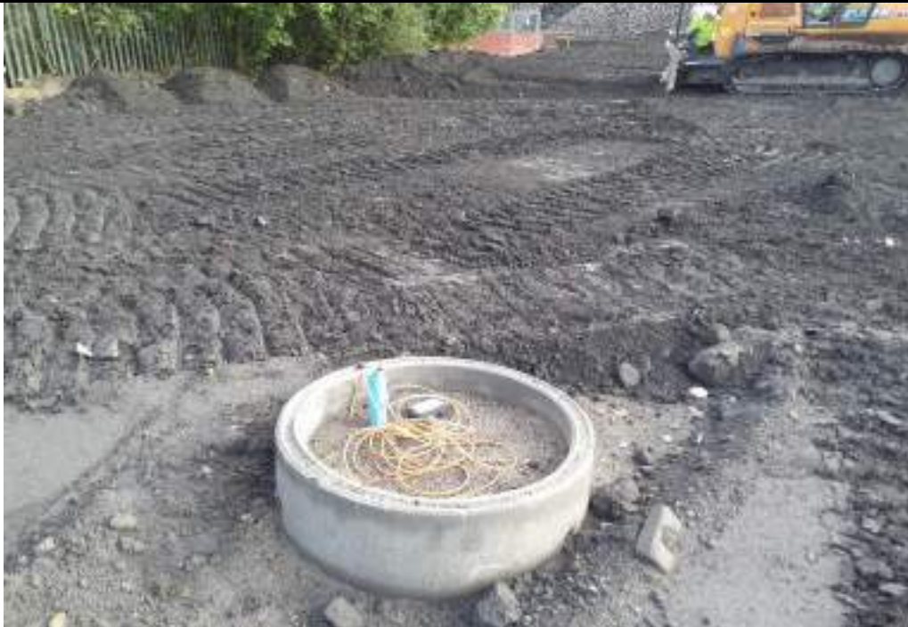
Photograph 20: Rod Settlement Gauge and Vibrating Wire piezometer in western part of the site.
