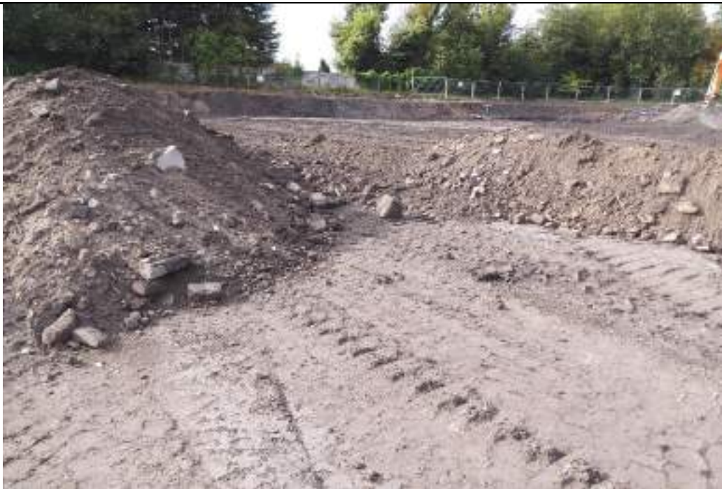
Photograph 20: Existence of oversize in fill material in southern part of the site. Material from northeastern stockpile.
