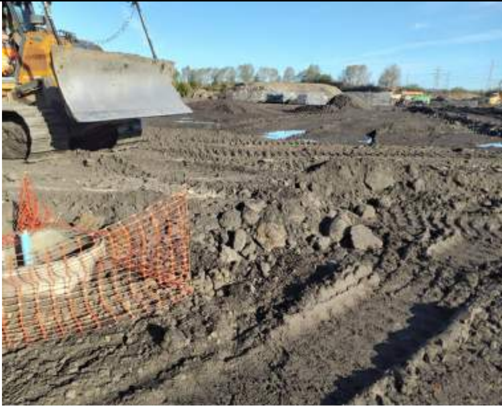
Photograph 19: Existence of oversized materials in fill in southwestern part of the site.
