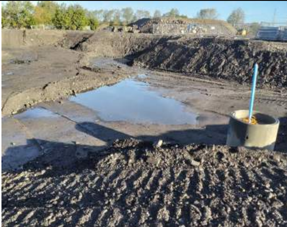
Photograph 7: Standing water in western part of the site.
