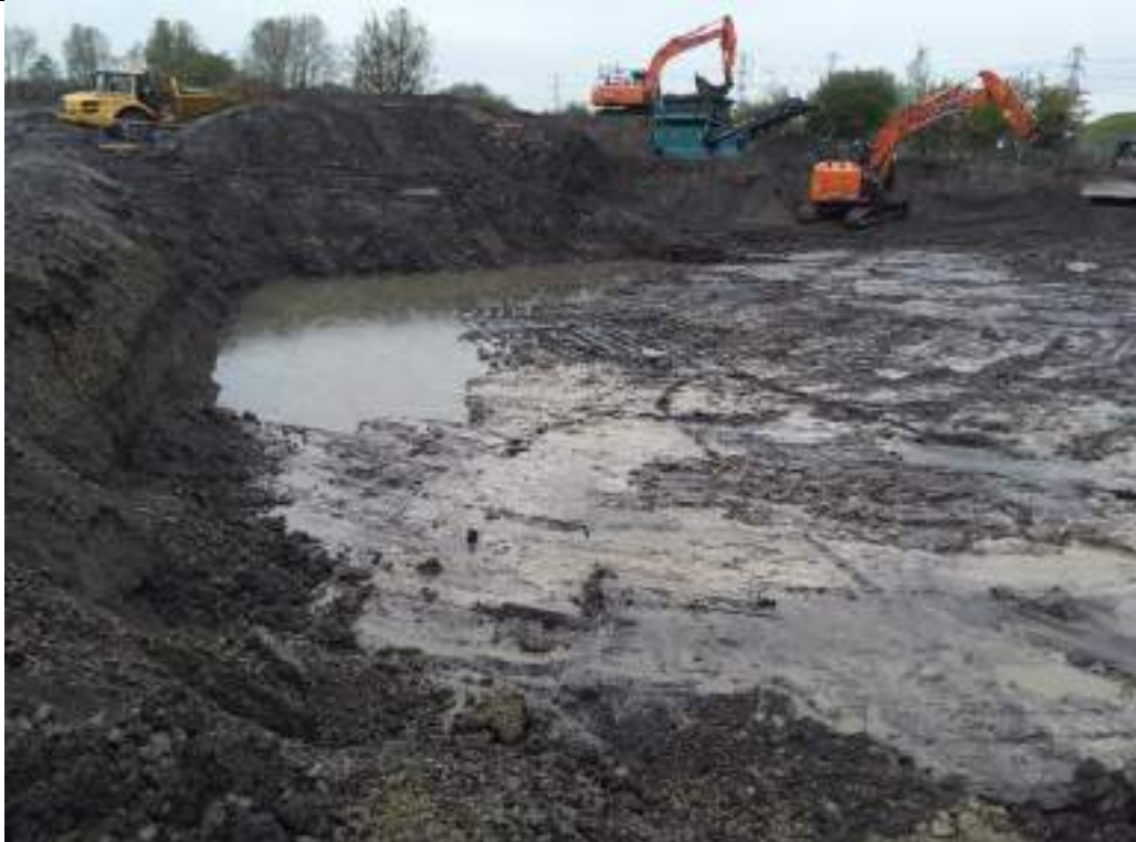
Photograph 16: Standing water in northeastern excavation.
