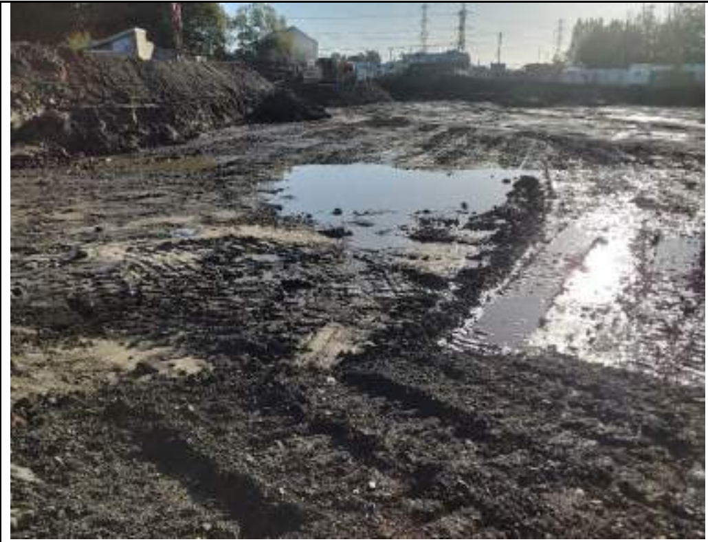
Photograph 9: Standing water in southeastern part of the site.
