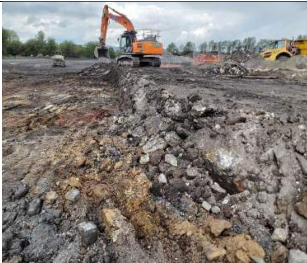
Photograph 8: Deleterious materials in excavation in southeastern part of the site.
