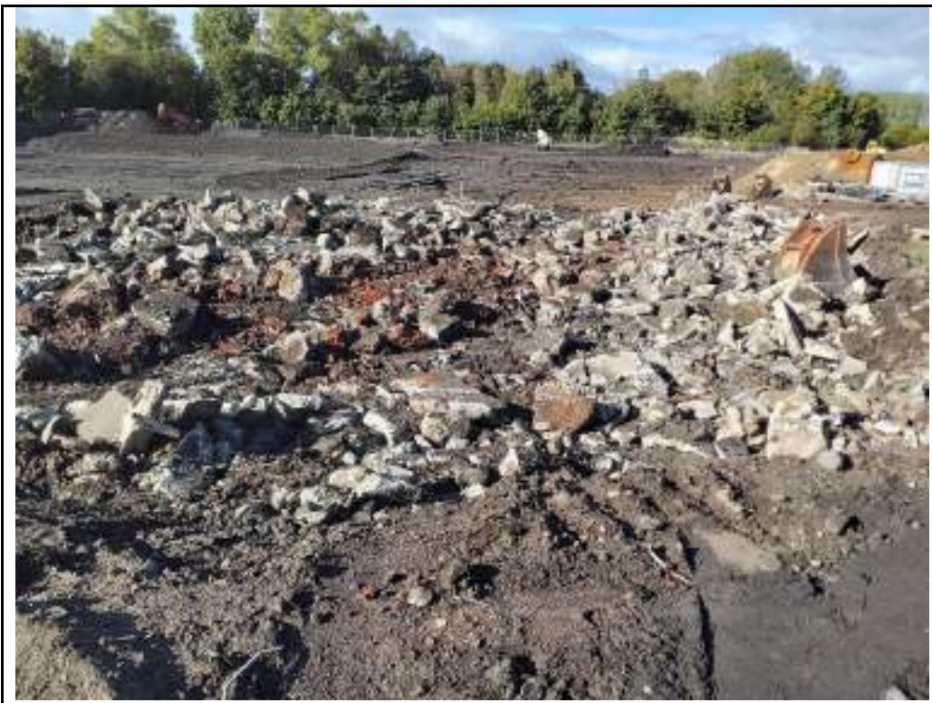
Photograph 2: Broken out concrete slab in southeastern part of the site.
