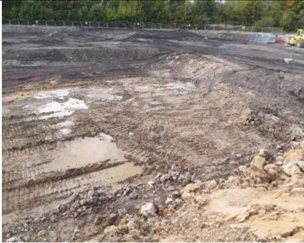
Photograph 23: Standing water in southeastern excavation.
