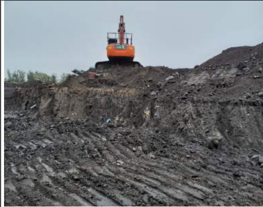
Photograph 15: Unbattered excavation in northeastern part of the site.
