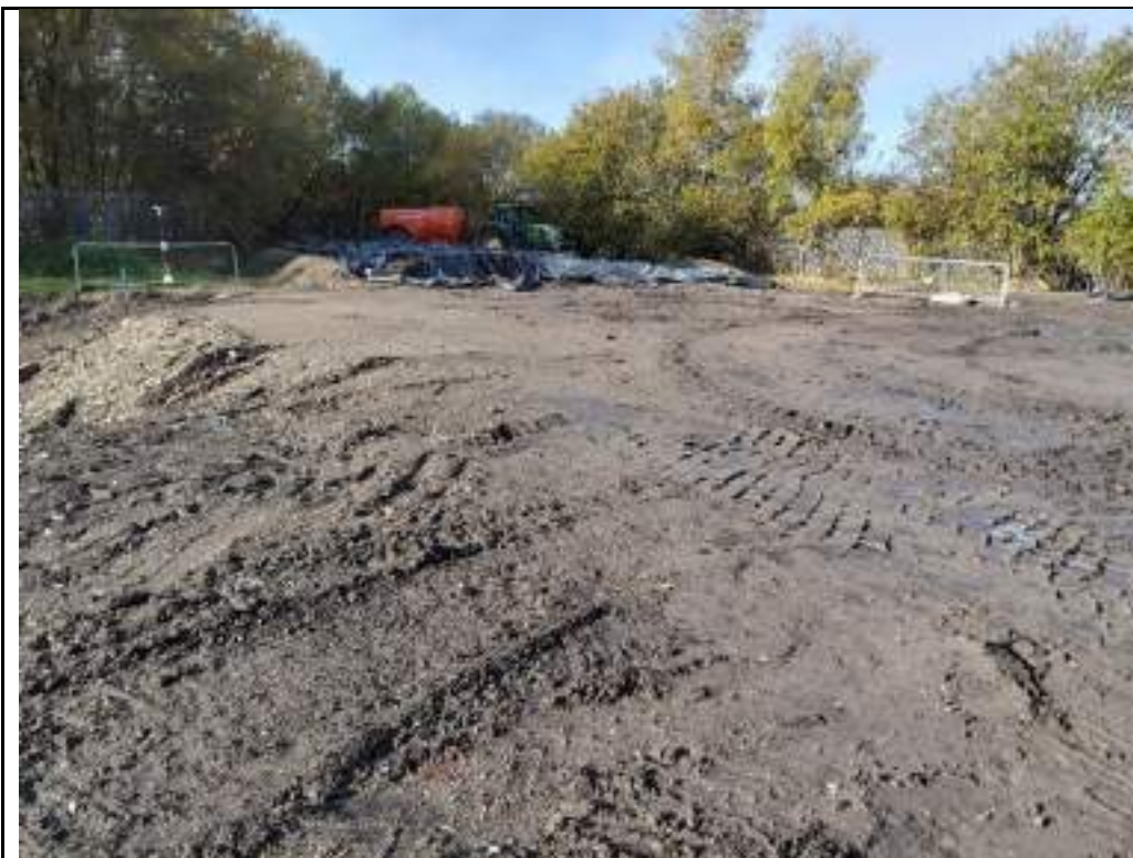
Photograph 12: Stockpile of TPH contaminated materials in northwestern boundary of the site.
