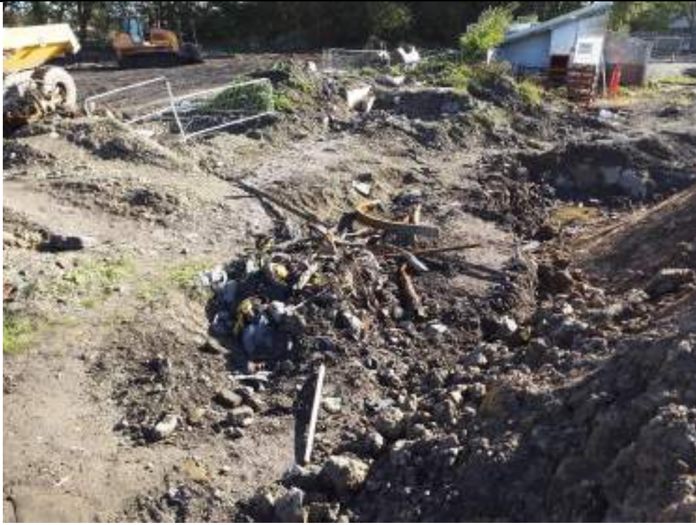
Photograph 5: Deleterious material in eastern part of the site.
