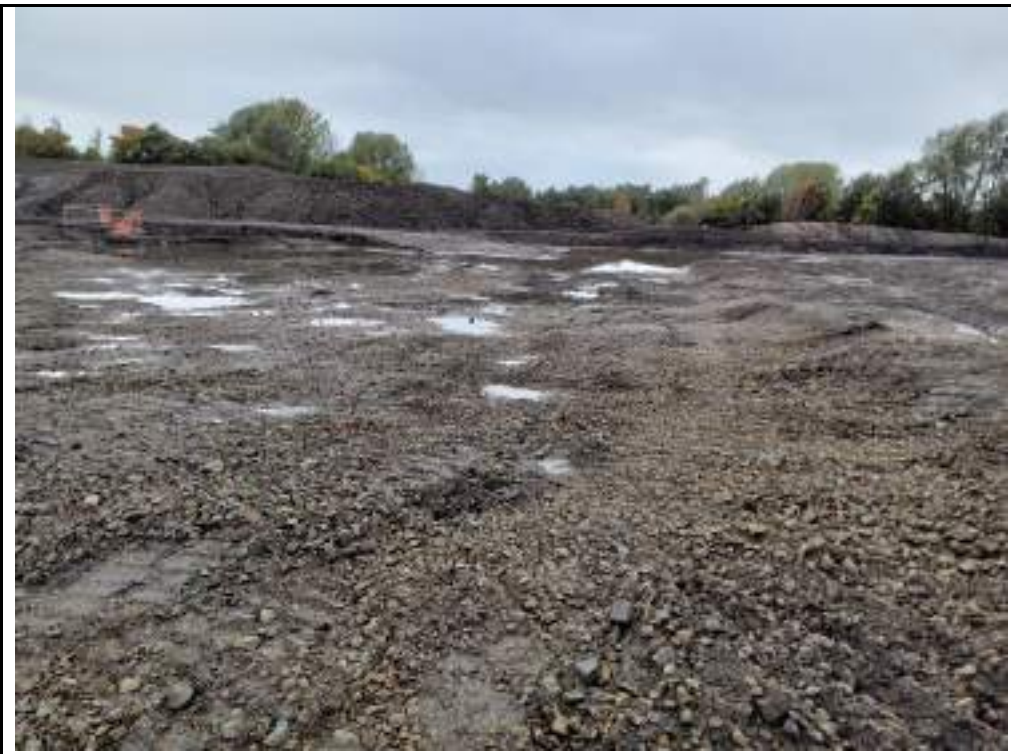
Photograph 4: Standing water in northern part of the site.
