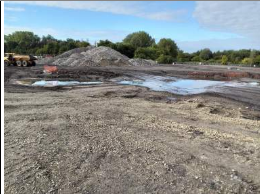
Photograph 9: Standing water in northern part of the site.
