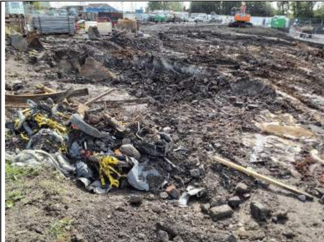
Photograph 147: Deleterious material in southeastern part of the site.
