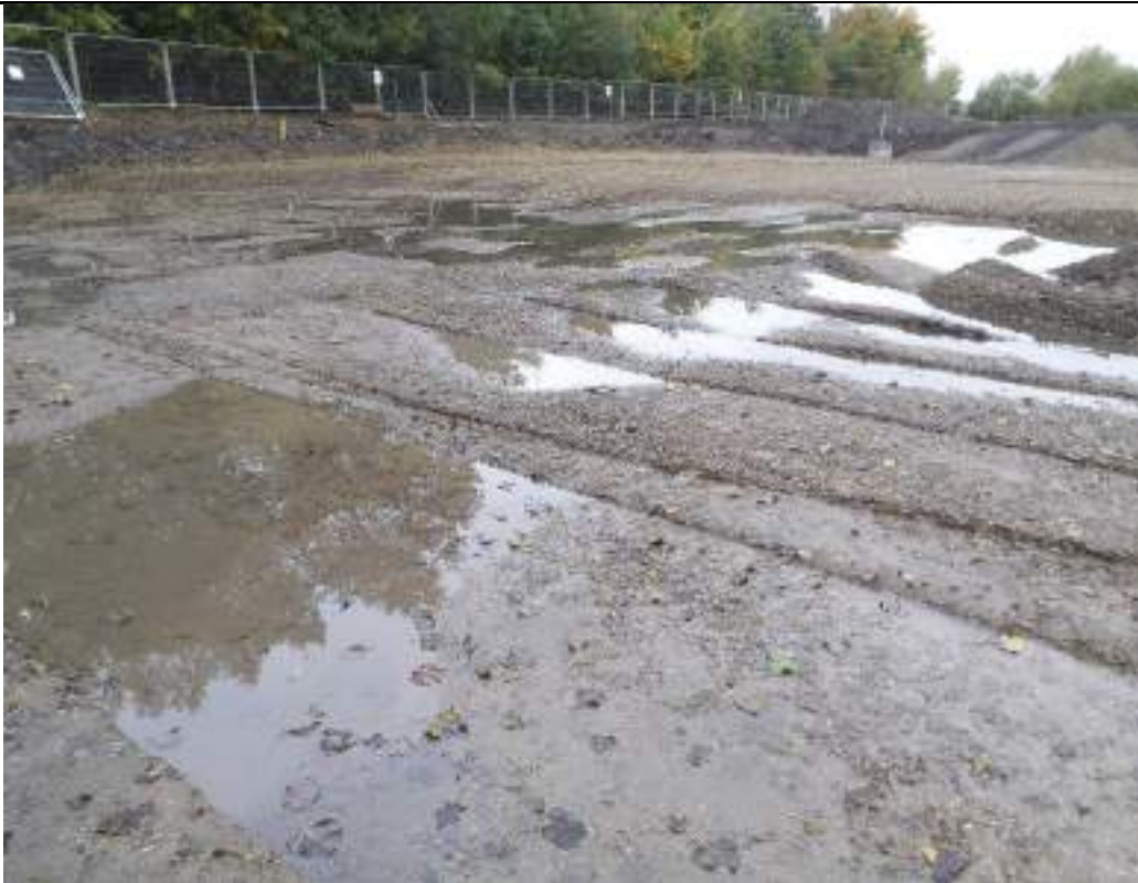
Photograph 16: Standing water in southwestern part of the site.
