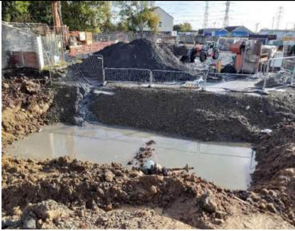
Photograph 7: Standing water in southeastern part of the site.
