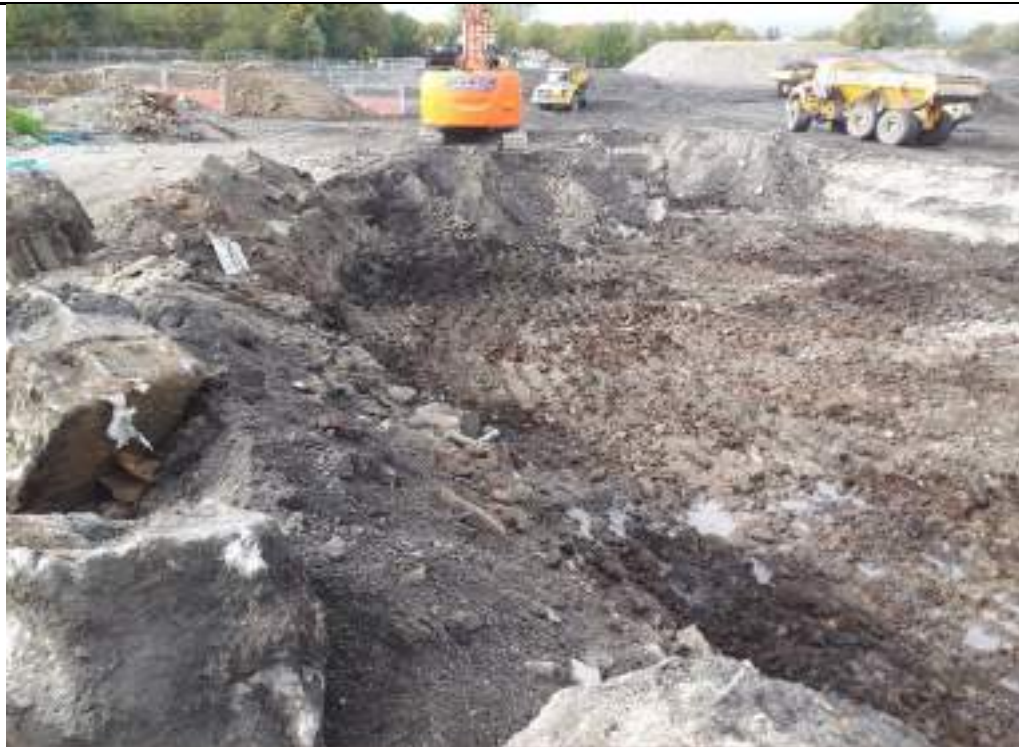
Photograph 18: Oversize and deleterious material in excavation in eastern part of the site.
