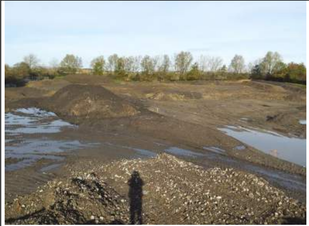
Photograph 15: Overview of stockpiles of unsuitable materials in northern part of the site.
