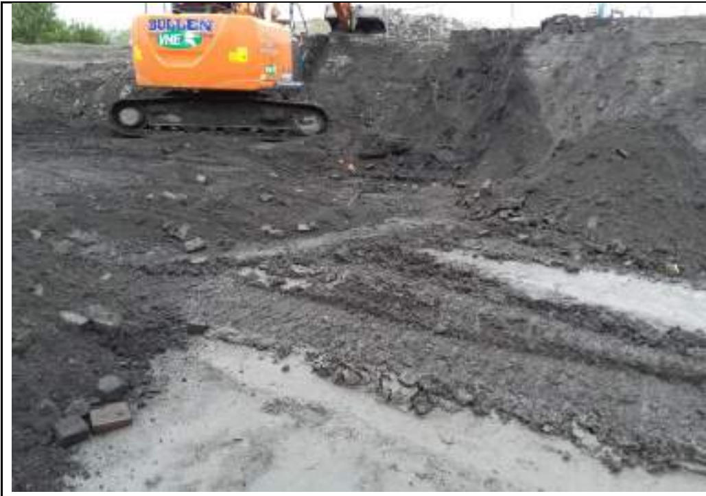
Photograph 11: Deleterious material in excavation in western part of the site.
