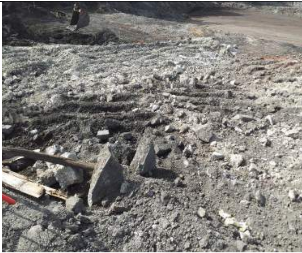
Photograph 8: Deleterious material in excavation in southern part of the site.
