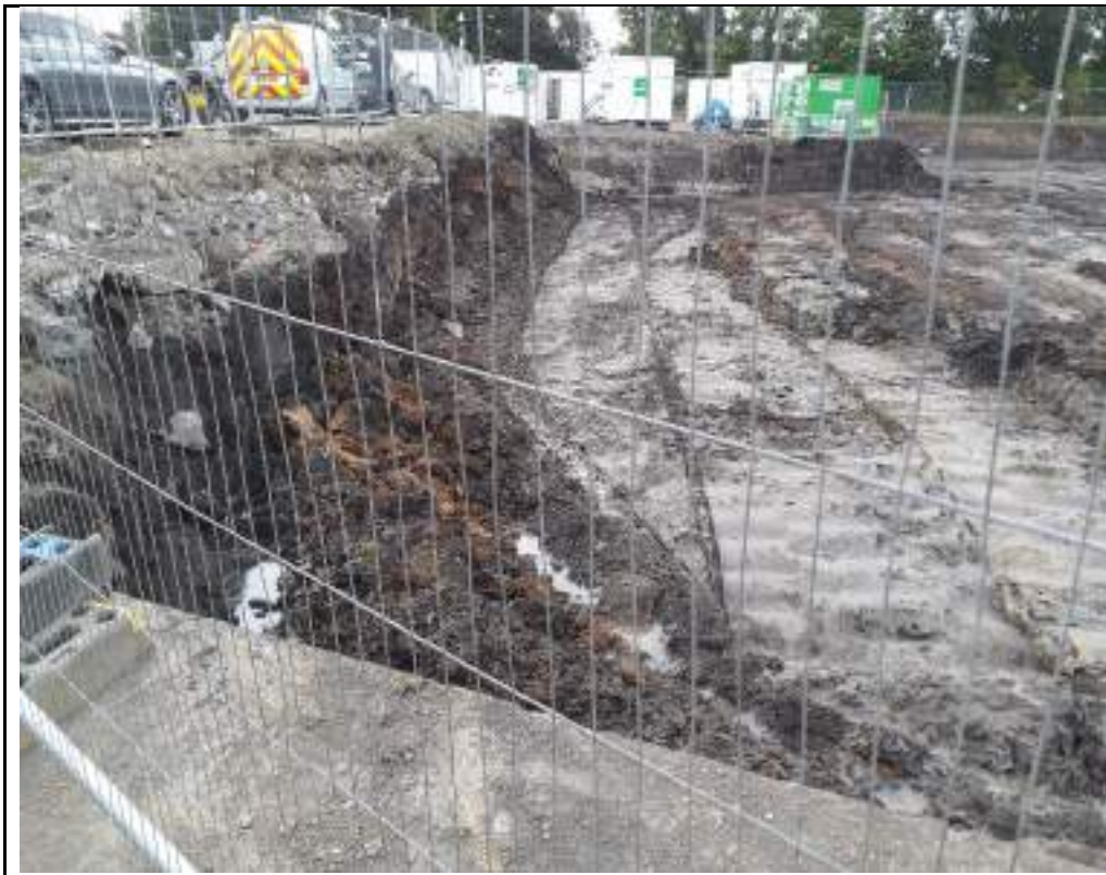
Photograph 2: Unbattered excavation in southeast of the site.
