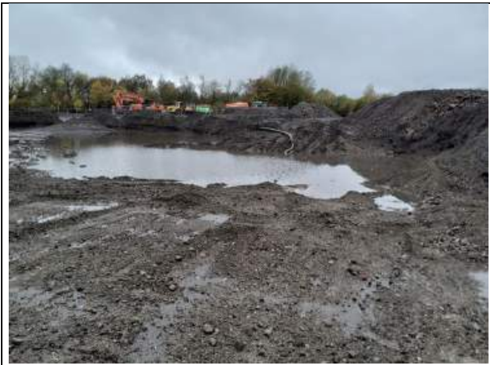
Photograph 4: Standing water in northeastern part of the site.
