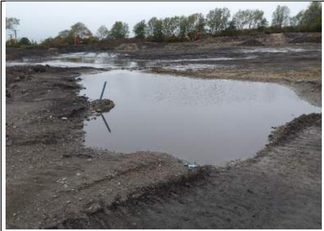
Photograph 9: Standing water in northern part of the site.
