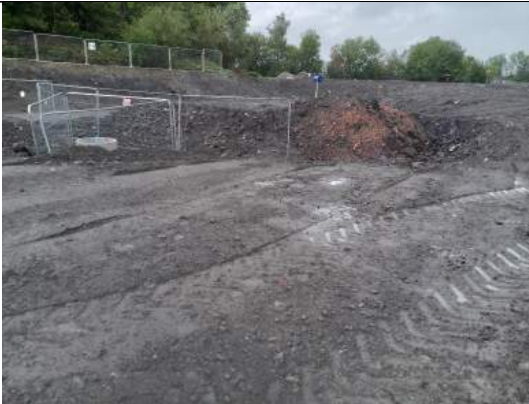
Photograph 10: Asbestos contaminated material stockpile in western part of the site.
