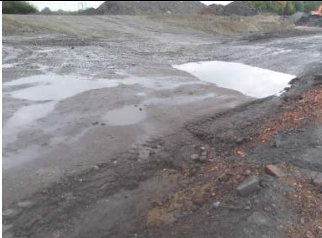
Photograph 12: Standing water in northern part of the site.
