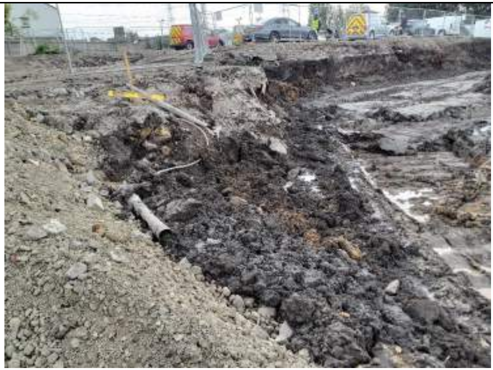
Photograph 4: Deleterious material in southeastern excavation.
