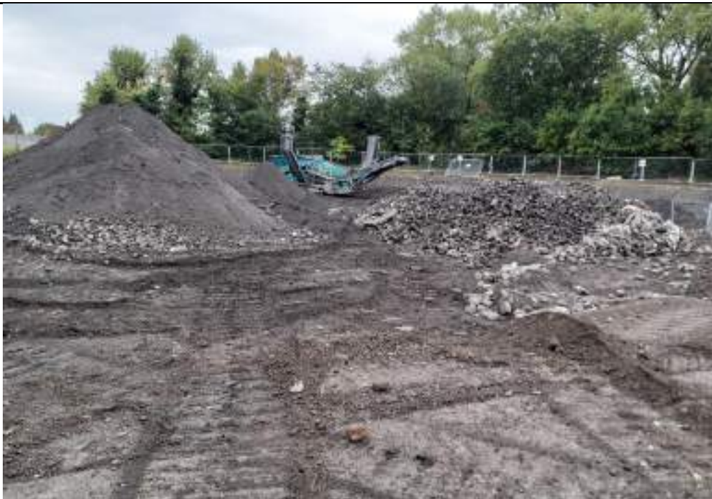
Photograph 26: Stockpile of asbestos contaminated material in southwestern part of the site after completion of processing and hand picking of asbestos.
