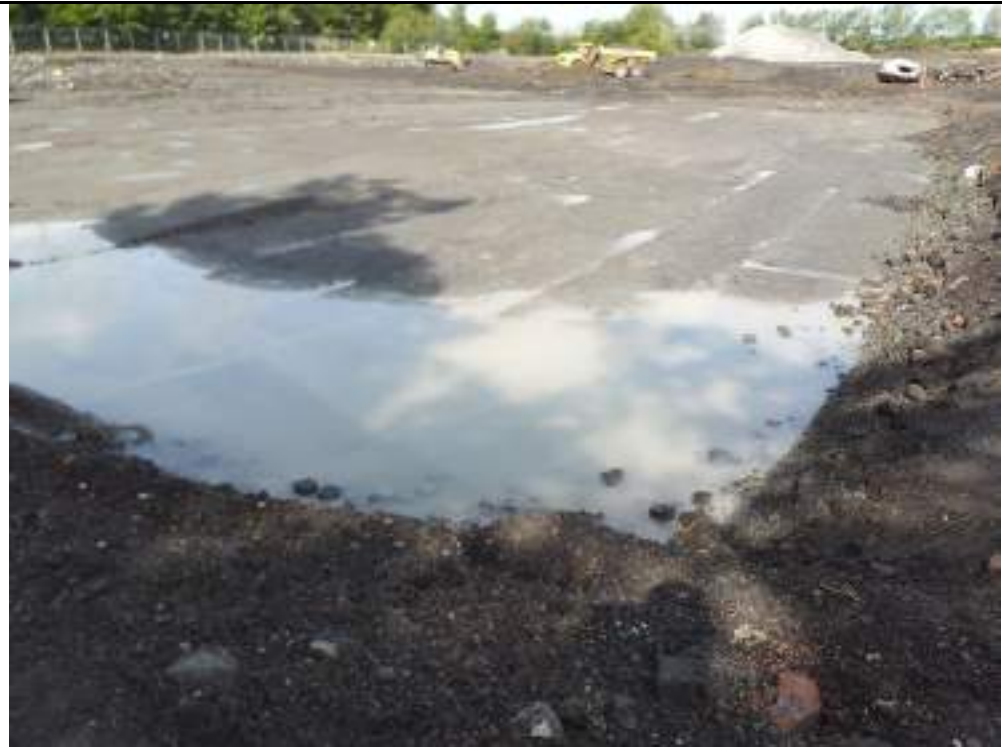
Photograph 4: Standing water in excavation in southern part of the site.
