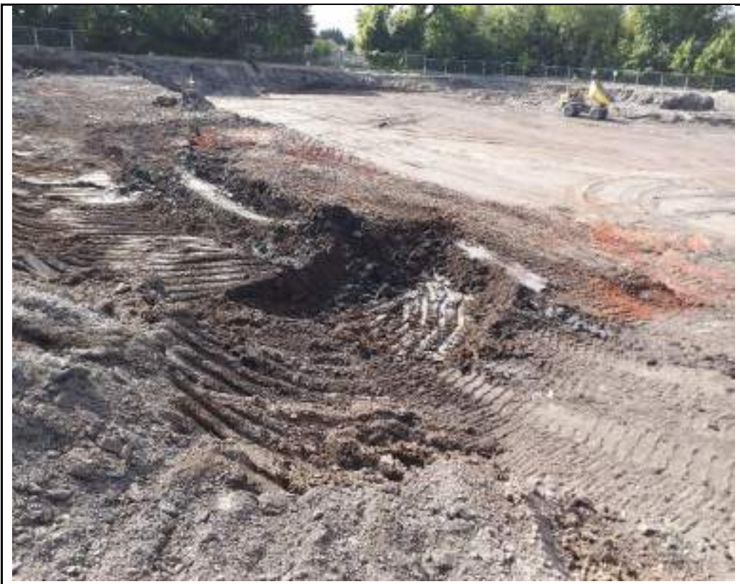
Photograph 110: Soft spot in excavation in southern part of the site.
