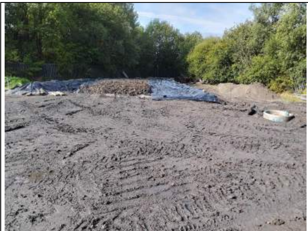
Photograph 110: Stockpile of potentially TPH contaminated material in northeast of the site. Material from excavation in southeastern part of the site.
