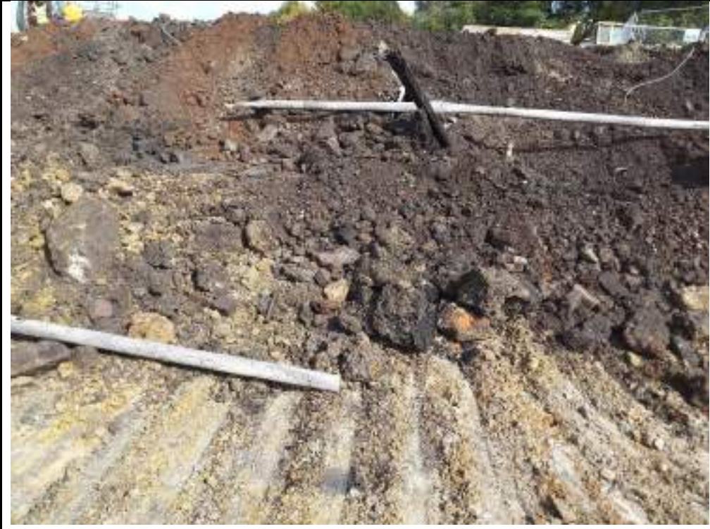
Photograph 3: Deleterious material in excavation in southern part of the site.
