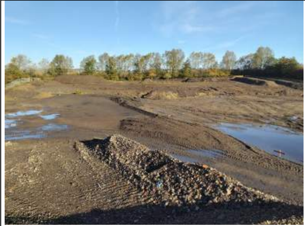
Photograph 93: overview of soft spot and Topsoil stockpiles in northern part of the site.
