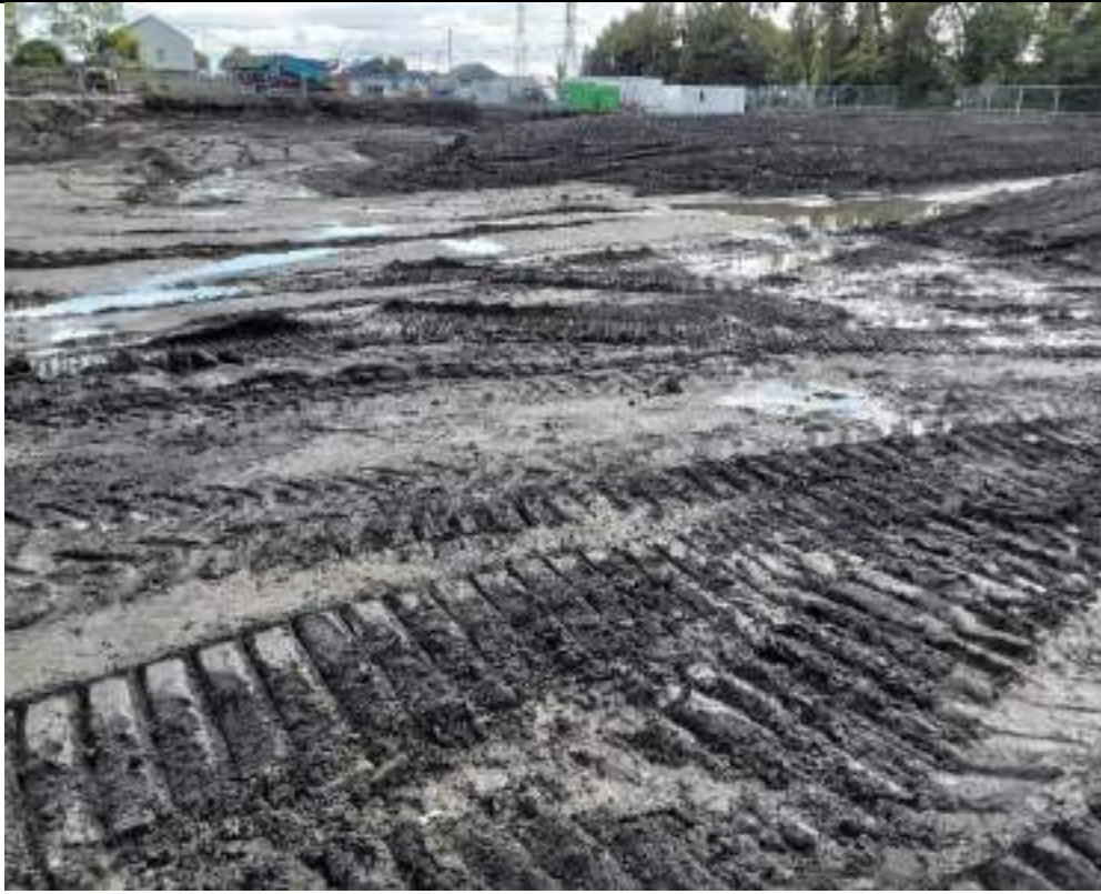
Photograph 7: Standing water in excavation in southern part of the site.
