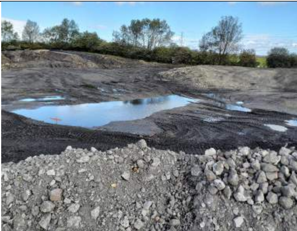
Photograph 18: Standing water in northern part of the site.
