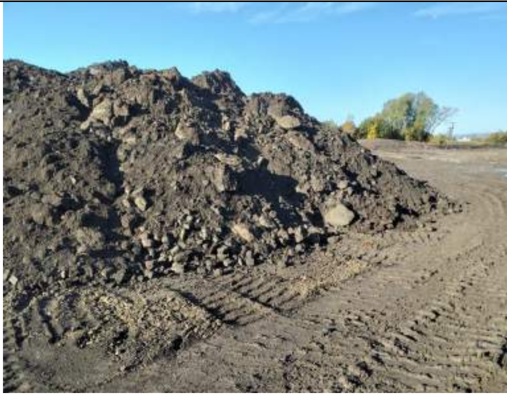
Photograph 15: Deleterious and oversized materials in stockpiled material in northeast of the site. Materials excavated from eastern excavation.
