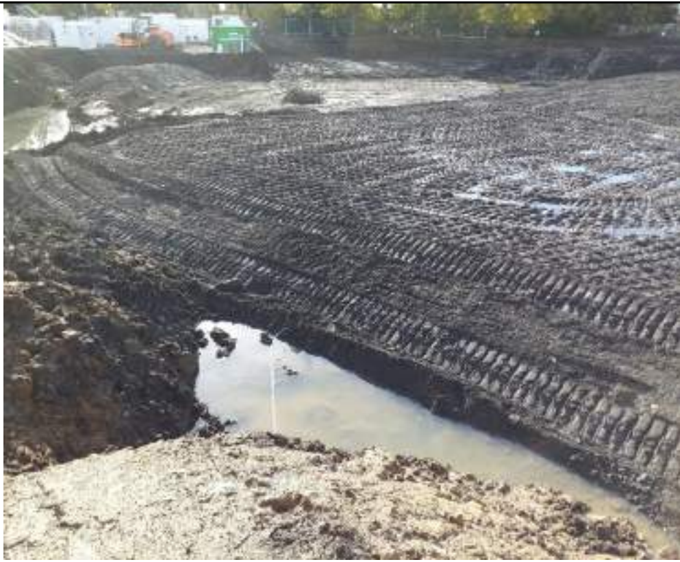
Photograph 8: Backfilled area and standing water in southeastern part of the site.
