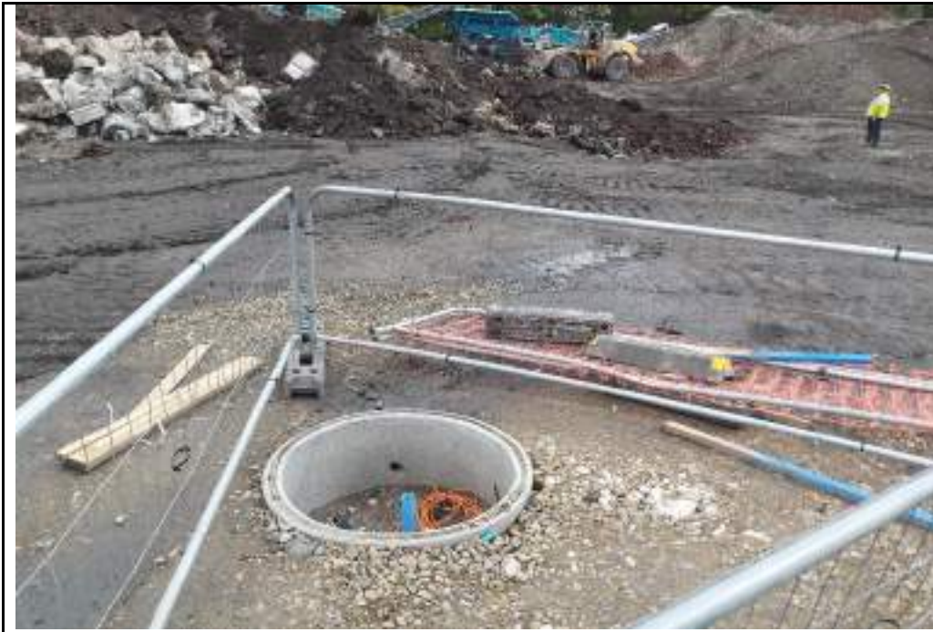
Photograph 179: Rod Settlement Gauge and Vibrating Wire piezometer in eastern part of the site.
