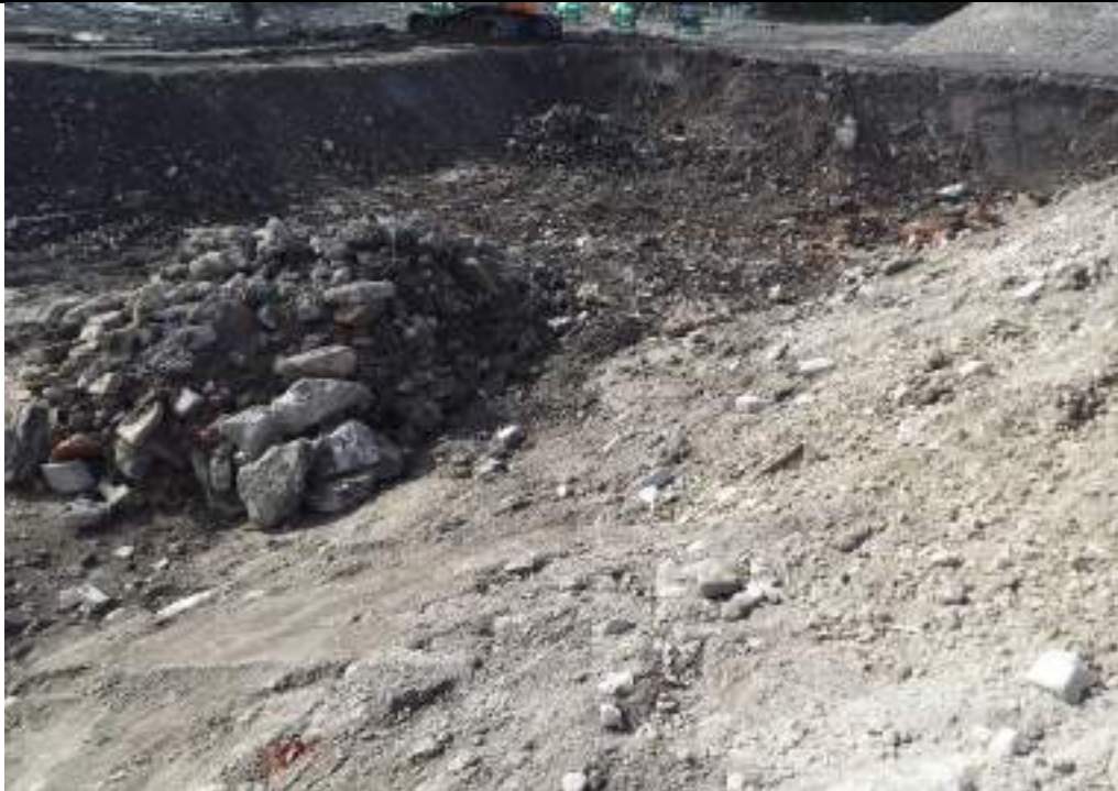
Photograph 20: Stockpile of oversize and deleterious materials in northeastern part of the site.
