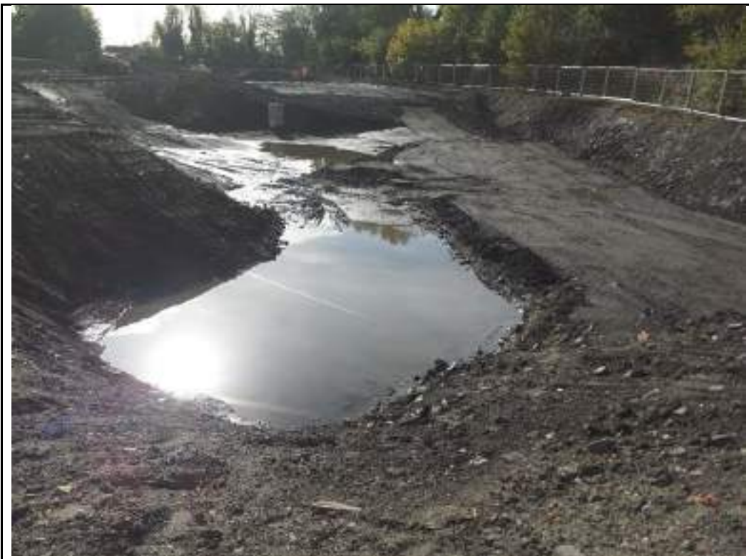
Photograph 14: Standing water in excavation in western part of the site.
