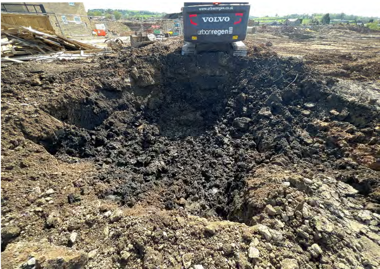
Photograph 27 – Area of deep Made Ground comprising hydrocarbon contaminated soils at northern extent.
