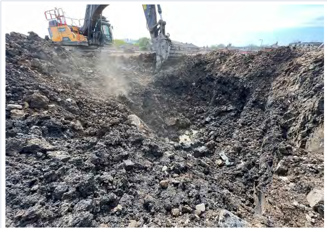
Photograph 28 – Area of deep Made Ground comprising hydrocarbon contaminated soils at northern extent.
