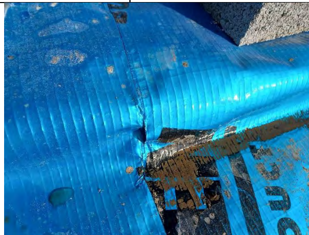
Plot 169: Joint requiring repair
