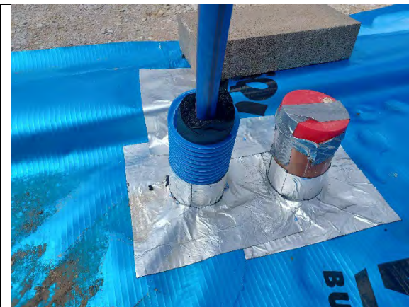
Plot 155: Service entry sealed with double and single sided tape.
