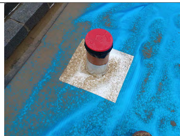
Plot 165: Service entry sealed with double and single sided tape.
