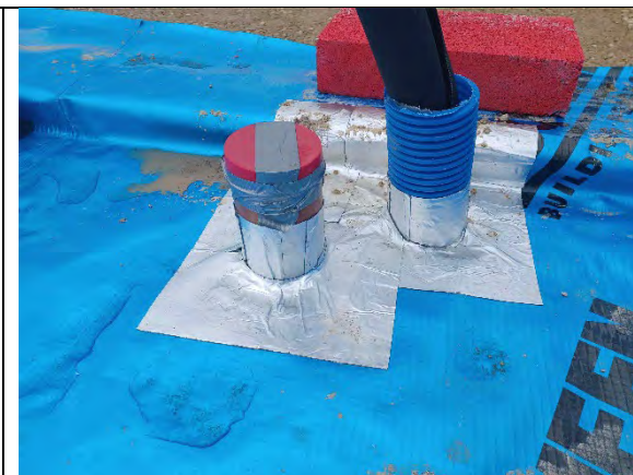
Plot 157: Service entry sealed with double and single sided tape.
