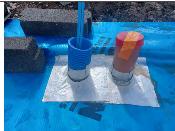
Plot 163: Service entry sealed with double and single sided tape.
