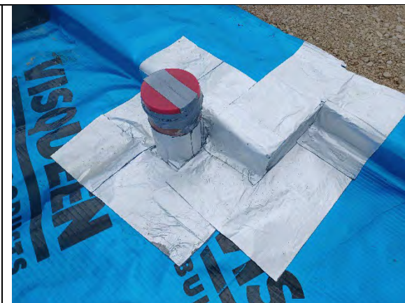
Plot 158 - Service entry sealed with double and single sided tape.
