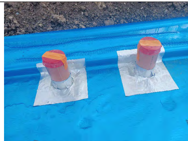
Plot 161: Service entry sealed with double and single sided tape.
