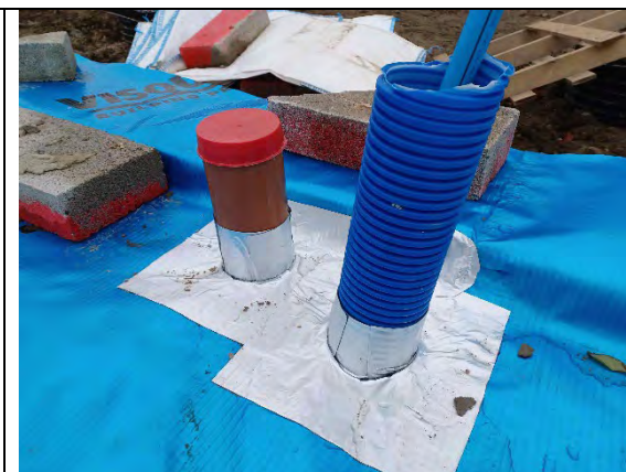
Plot 179: Service entry sealed with double and single sided tape.
