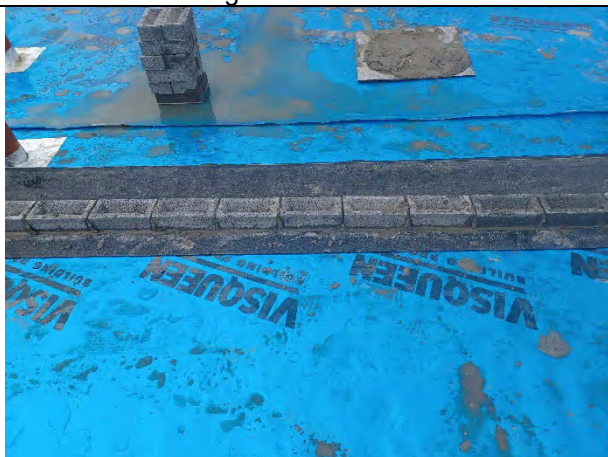
Plot 162: Membrane extends under the interior wall.
