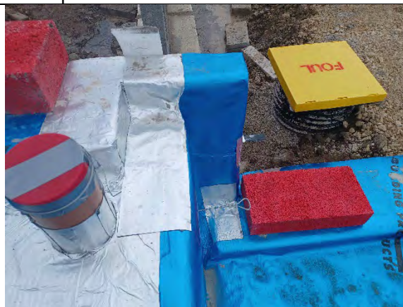
Plot 157: Membrane extending over external wall in Plot 158.
