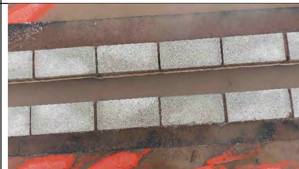
Plot 3 & 4 membrane runs under DPC spanning Cavity wall – this section is a single sheet with no joint to DPC
