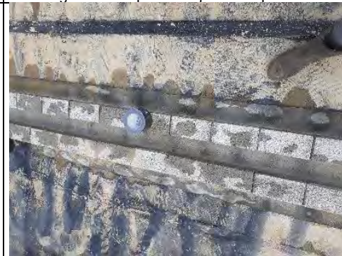
Plot 144-145: membrane runs under DPC spanning Cavity wall – this section is a single sheet with no joint to DPC
