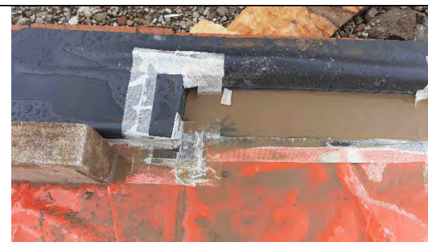
Plot 4: corner detail from folding DPC, some standing water no holes visible in joints
