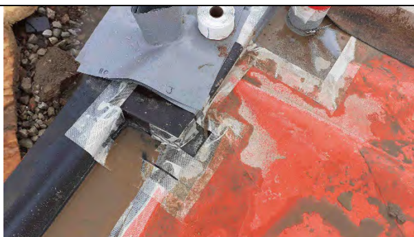
Plot 3: corner detail from folding DPC, some standing water no holes visible in joints
