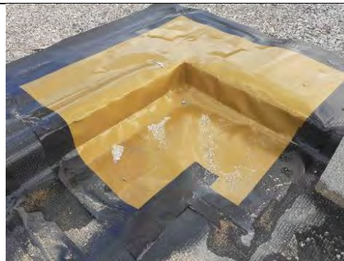
Plot 144: Corner detail, some standing water no holes visible in joints
