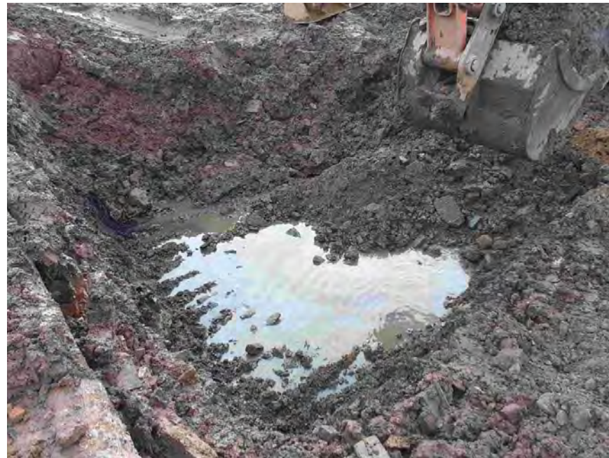
General view south over HS10-Cell 2- hydrocarbon sheen visible on groundwater ingress. Very strong white spirit / gasoline odour
