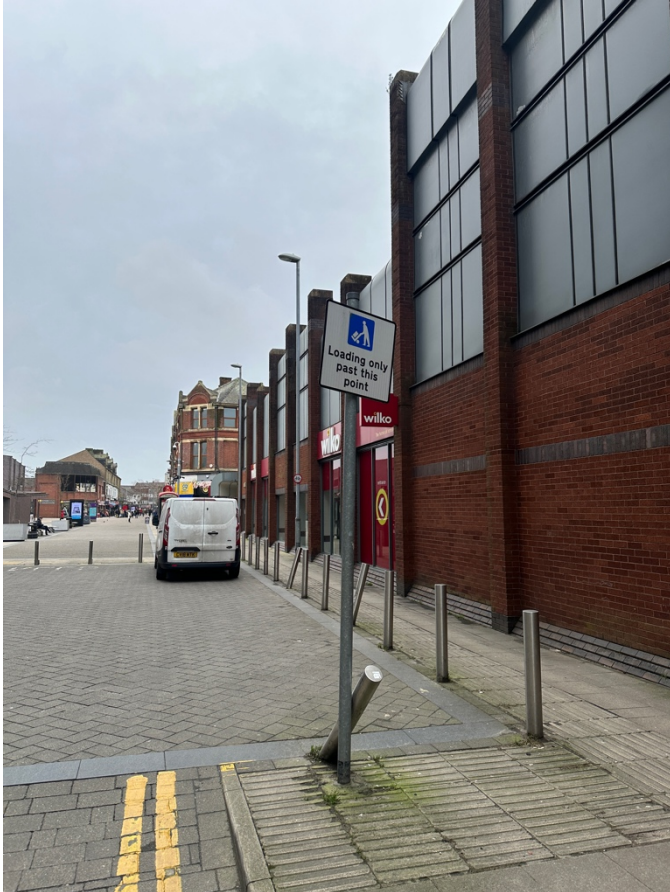
Damage to bollards within designated loading area.
