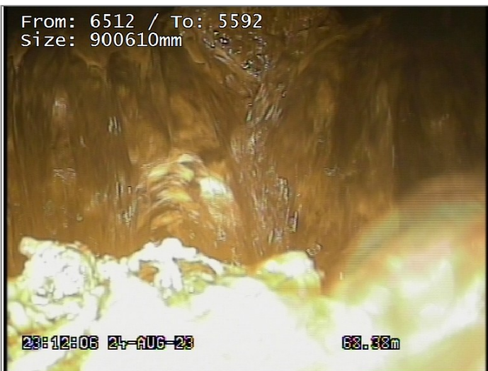
Finish node type, manhole, reference 5592
