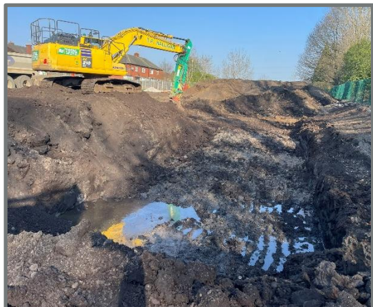
Soft spot in base of excavation
