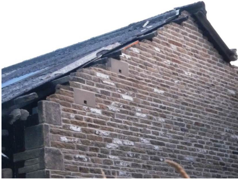
Example of Forticrete boxes in situ
